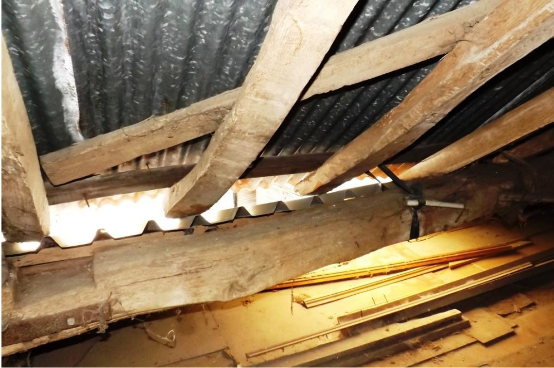
Plate 26. Rafters no longer supported or joined to top plate (evidence of lowering of roof)
