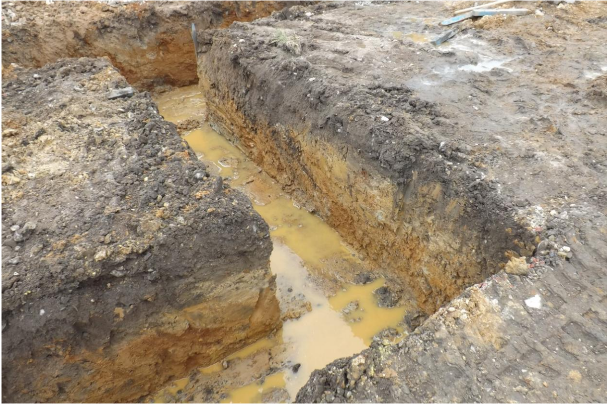
Plate 9. Section from footings trench (plot 2) , from the north-west (where sub-soil and some top soil remained on the west end of the site
