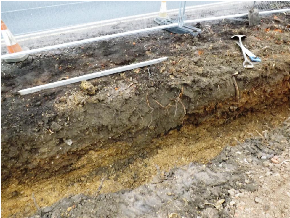
Plate 9. Section through Tr1 showing shallowest depth of (1042) layer, next to the road
