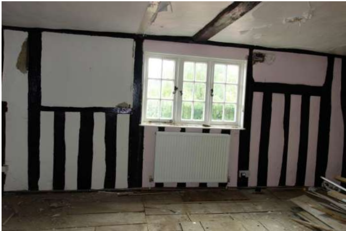
Plate 29. First floor of cross-wing showing original window casements, now blocked off either side of later window
