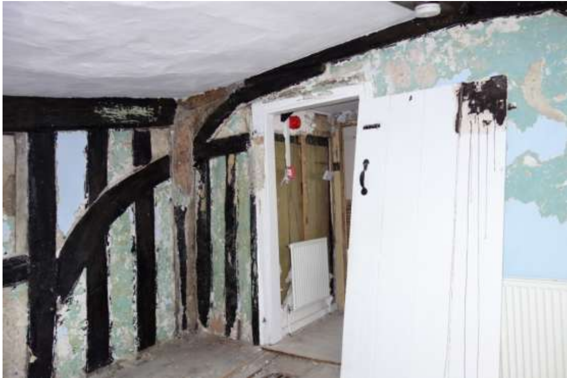
Plate 22. First floor studwork in phase 1 showing altered arch bracing to accommodate the doorway
