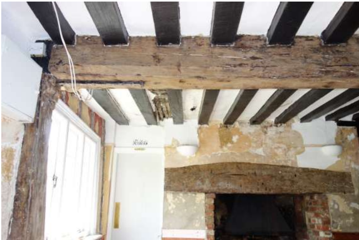
Plate 10. Bridging beam in hall/lounge showing Ogee moulding to top of storey post
