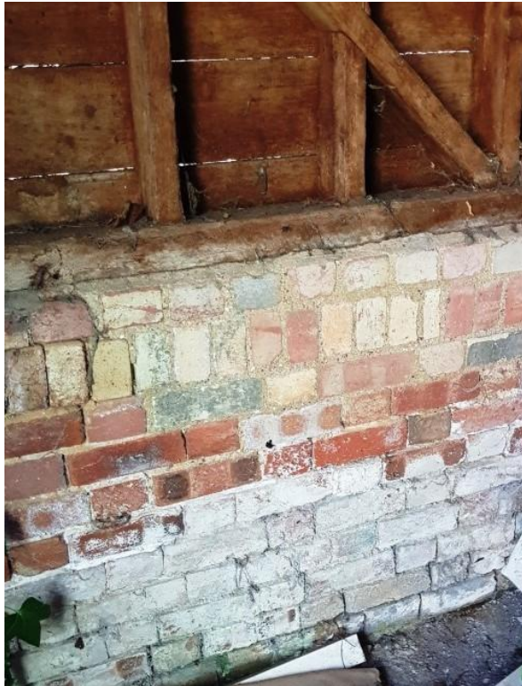
Plate 40. Interior of shed to west of cow house with 19th-20th century brickwork
