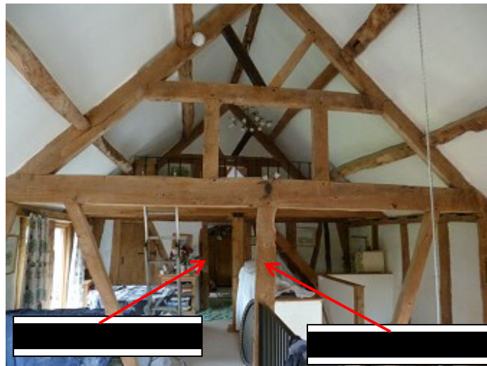
Figure 6c/d: Drawing (after Duncan James) and annotated photograph of the barn trusses to locate sampled timbers (see Table 1)
