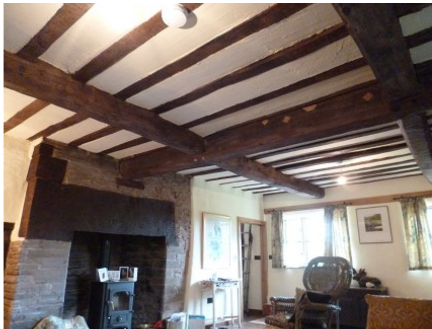
Figure 4a/b: Interior views of the cross-wing range; west purlins trusses 1 – 2 (top) and ground floor ceiling beams (bottom)
