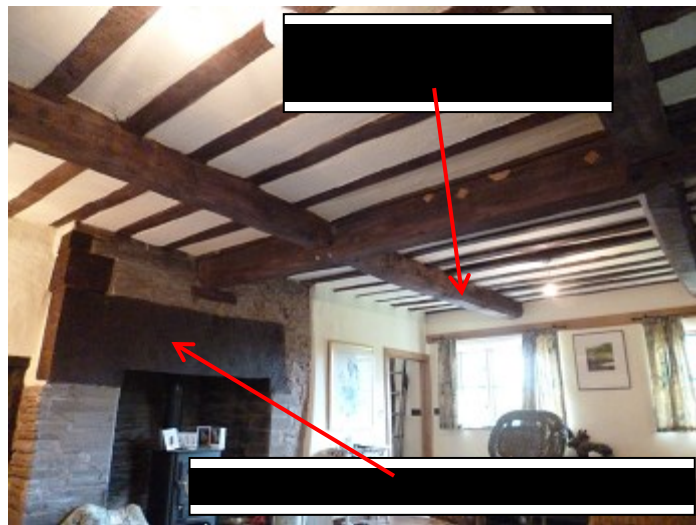
Figure 6a/b: Drawing (after Duncan James) and annotated photograph of the cross-wing to locate sampled timbers (see Table 1)
