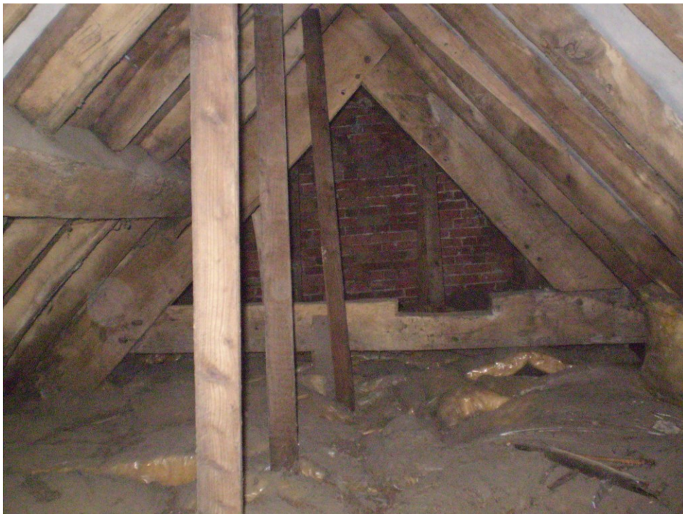
Figure 5a/b: Views of the coupled common rafter roof of the main range (top), and the southwest wing roof (bottom), with its potentially reused principal rafter truss.
