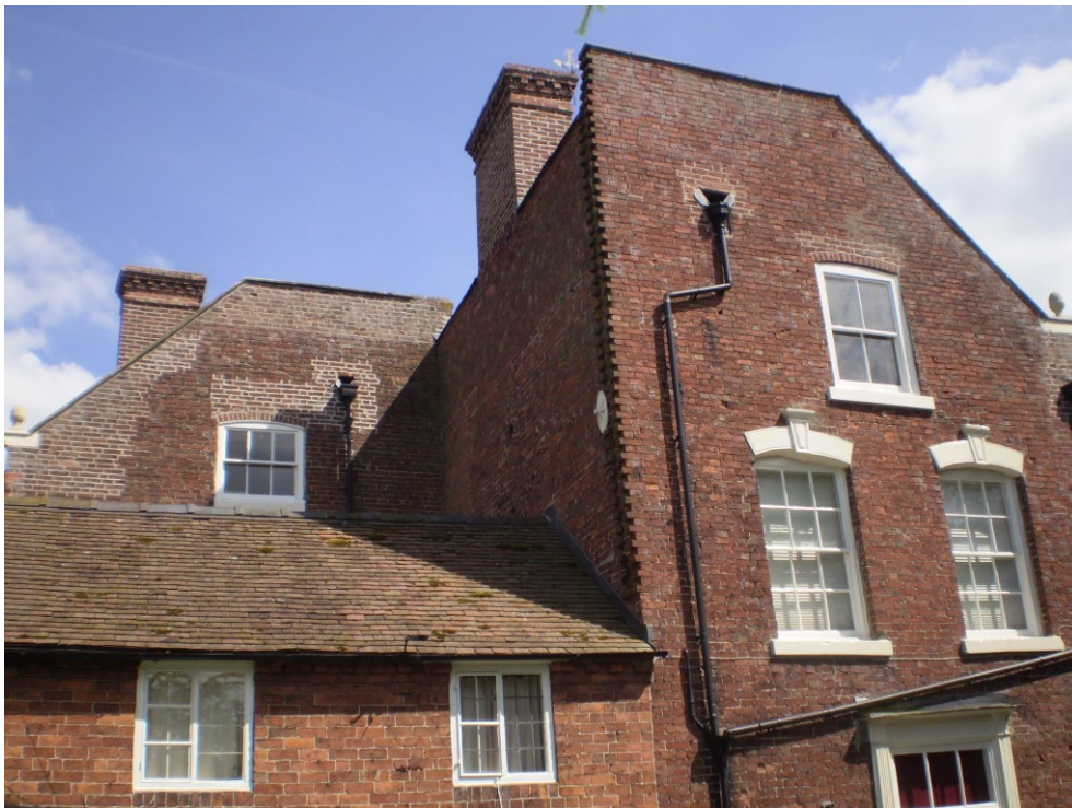
Figure 1a/b: Views of Wytheford House from the southwest (top) and northwest (bottom) showing how the northwest corner of the house has not been built
