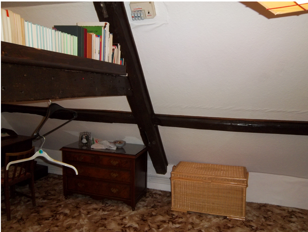
Figure 4a/b: View of the north principal of truss II (top) and the north principal of truss III (bottom)
