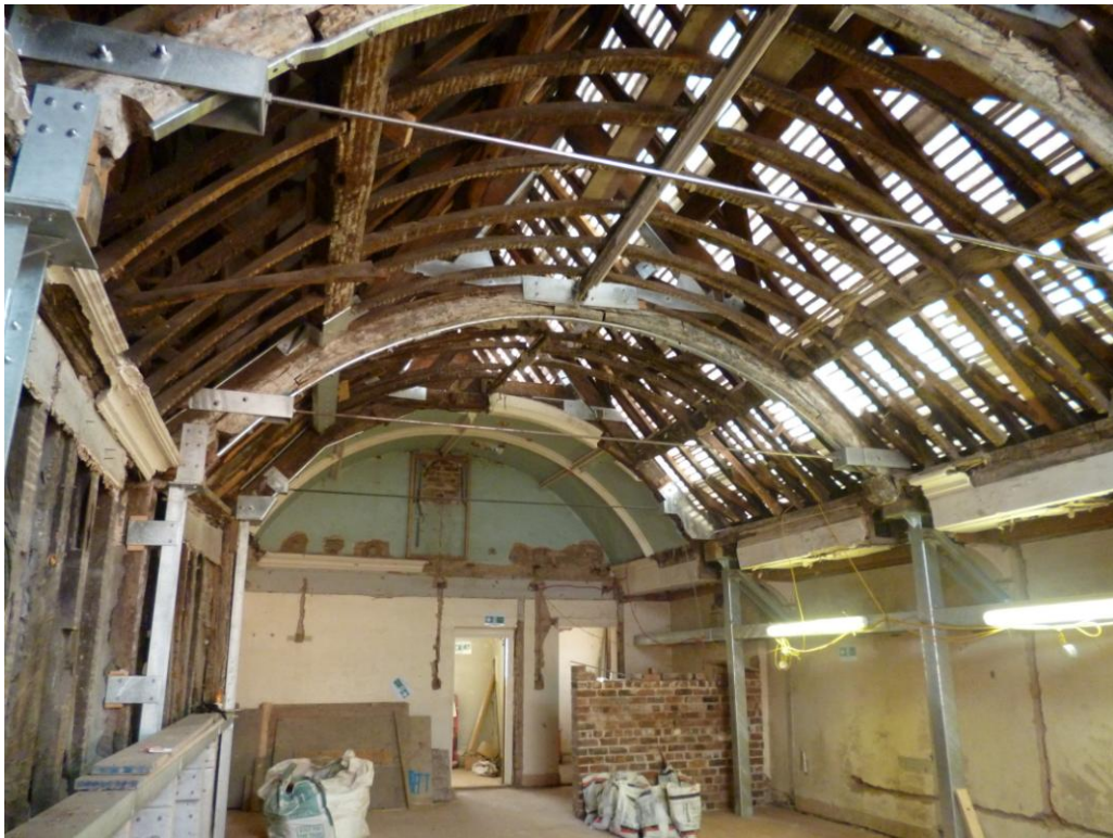
Figure 2a/b: View of the remnant west truss of the hall range, hidden by later studs (top), and the trusses of the west cross-wing (bottom)
