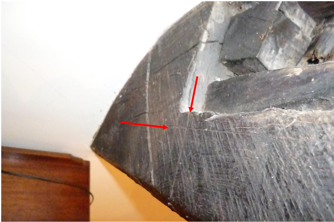
Figure 4a: Scribed marking-out lines for the cutting of the mortice joint in the front principal rafter
