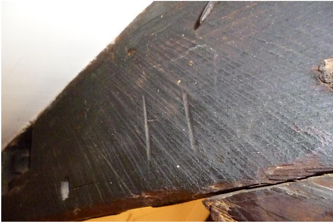
Figure 4b: Assembly mark for a mortice and tenon joint between collar and rafter
