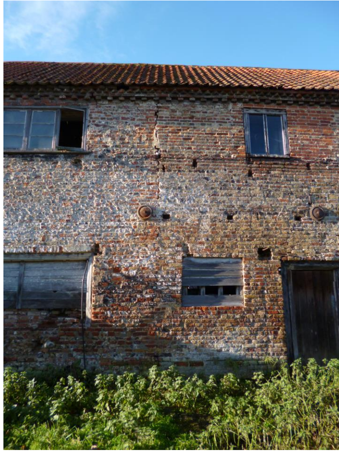
Figure 5: View of the open jointed brickwork to the east face of the barn believed to indicate a possible junction of two buildings.
