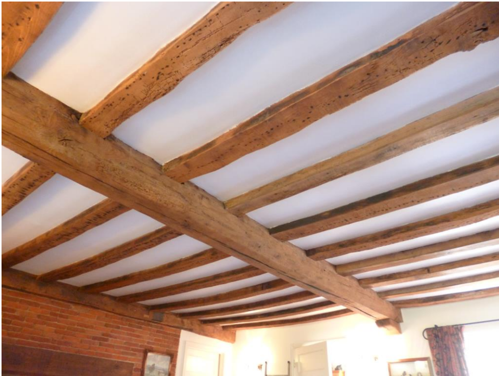
Figure 2a/b: External view of the Hall showing the primary range between the two projecting wings (top), and internal view of ground floor ceiling joists (bottom)
