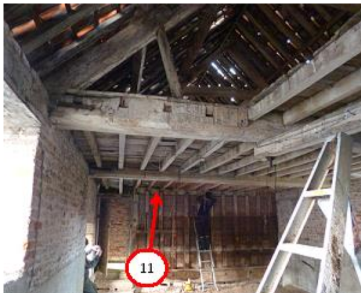
Figure 6c/d: Views of the interior of the barn to locate the sampled timbers (see Table 1)
