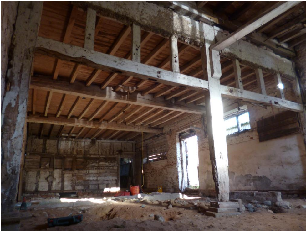
Figure 4a/b: View of the roof trusses to the barn (top) and the ground floor ceiling beams and partition wall (bottom)
