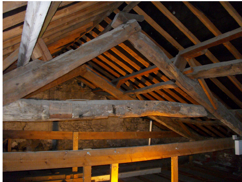
Figure 4f/g: View of the roofs to 2 Bridge Street (top) sampled as BID-A04–A11, and 3 Bridge Street (bottom), sampled as BID-A12–A19
