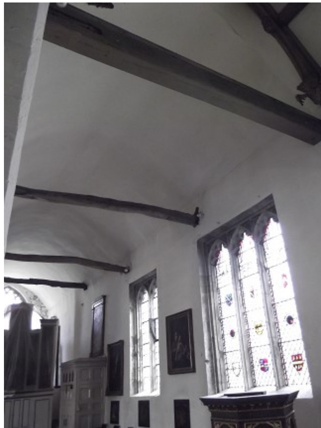
Figure 3a/b: Internal views of the north aisle looking west to east (top) and east to west (bottom). It is above this latter area that the samples analysed here have been obtained
