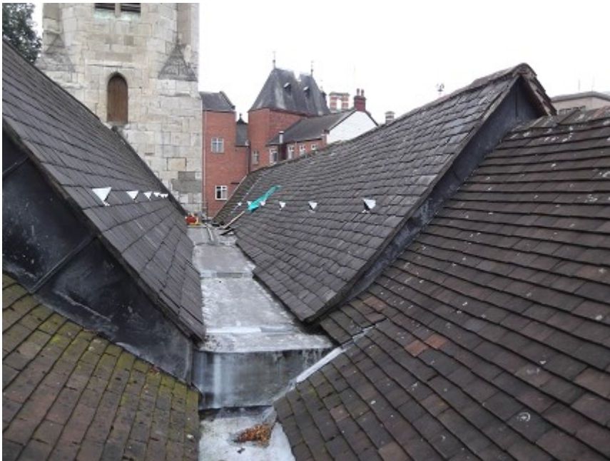
Figure 4a/b: Views of the north aisle roofscape looking west to east (top) and east to west (bottom)
