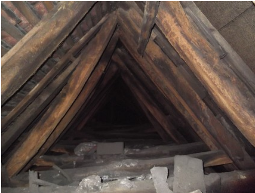
Figure 5a/b: Views of the roof trusses to the west end of the north aisle looking west to east (top) and east to west (bottom)
