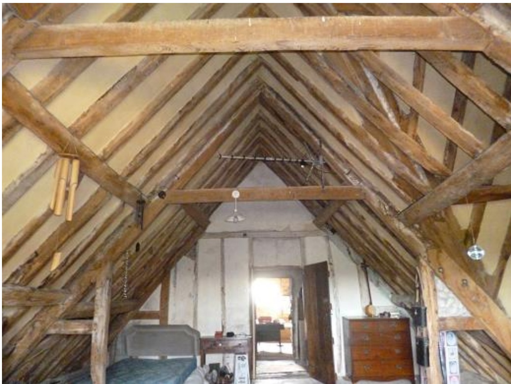
Figure 2a/b: Views of roof to the front wing, looking north to south (top) and to the west end of the rear range, looking west to east (bottom)
