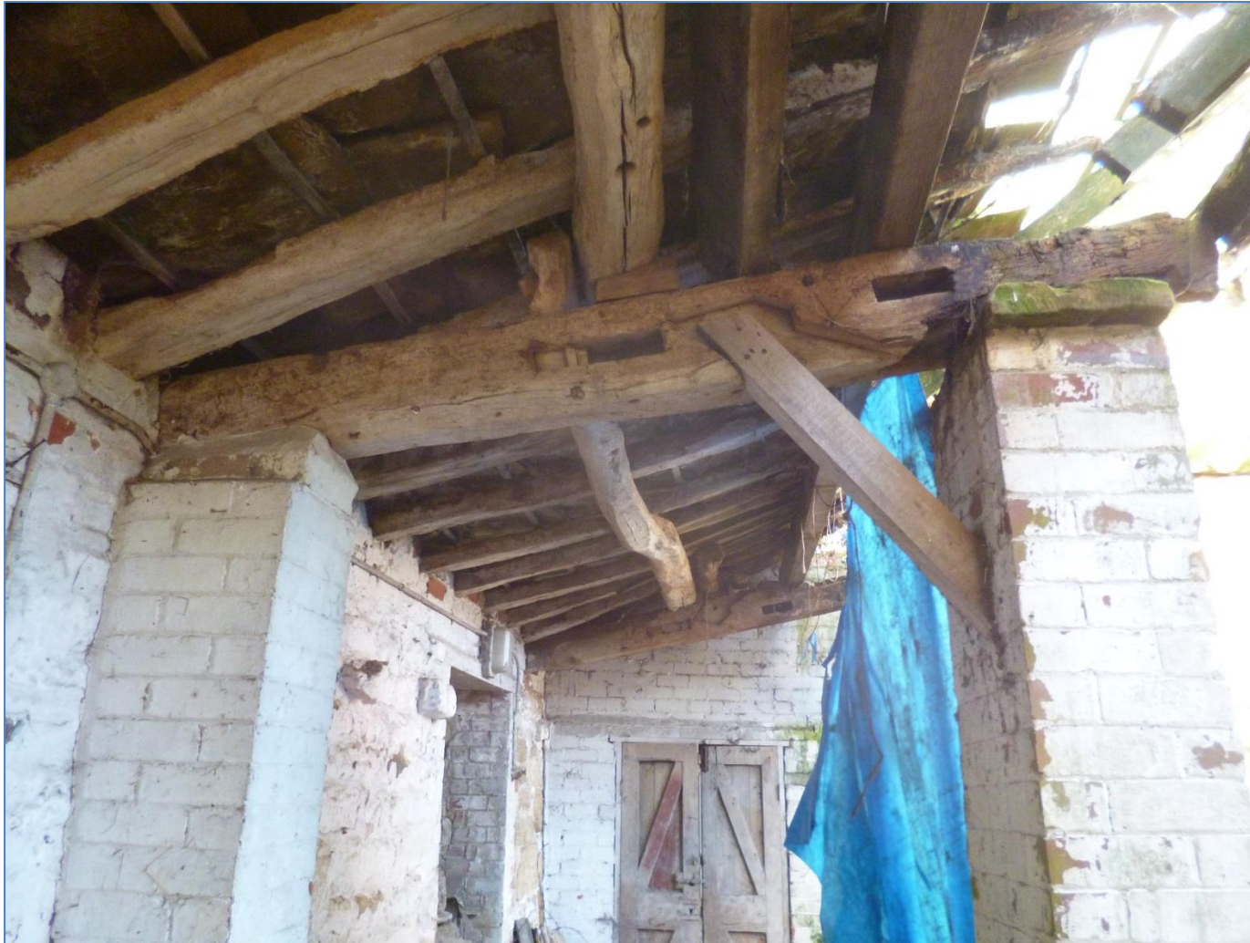
Figure 19: Aisle ties of the barn, the redundant mortices and lap joints clearly demonstrate a previous use for this timber (aisle tie 3) and the one in the background (aisle tie 2), photograph taken from the south
