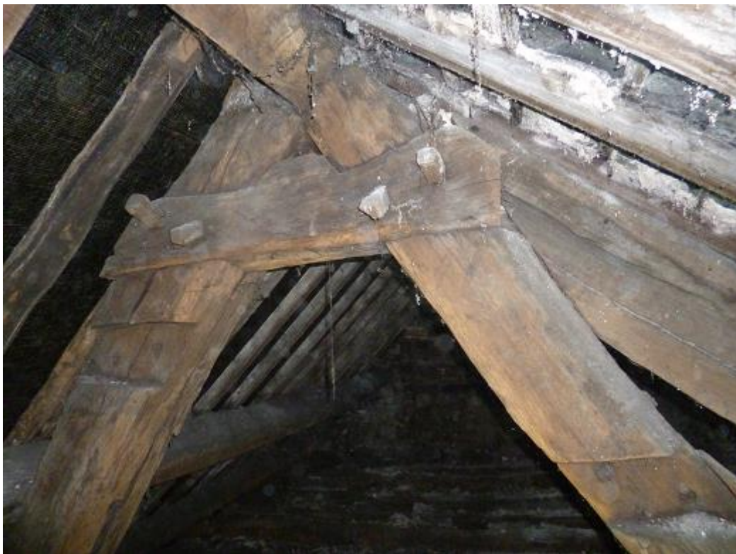
Figure 3a/b: View of truss 1 (east truss), showing east face (top) and truss 2 (west truss), also showing east face (bottom)
