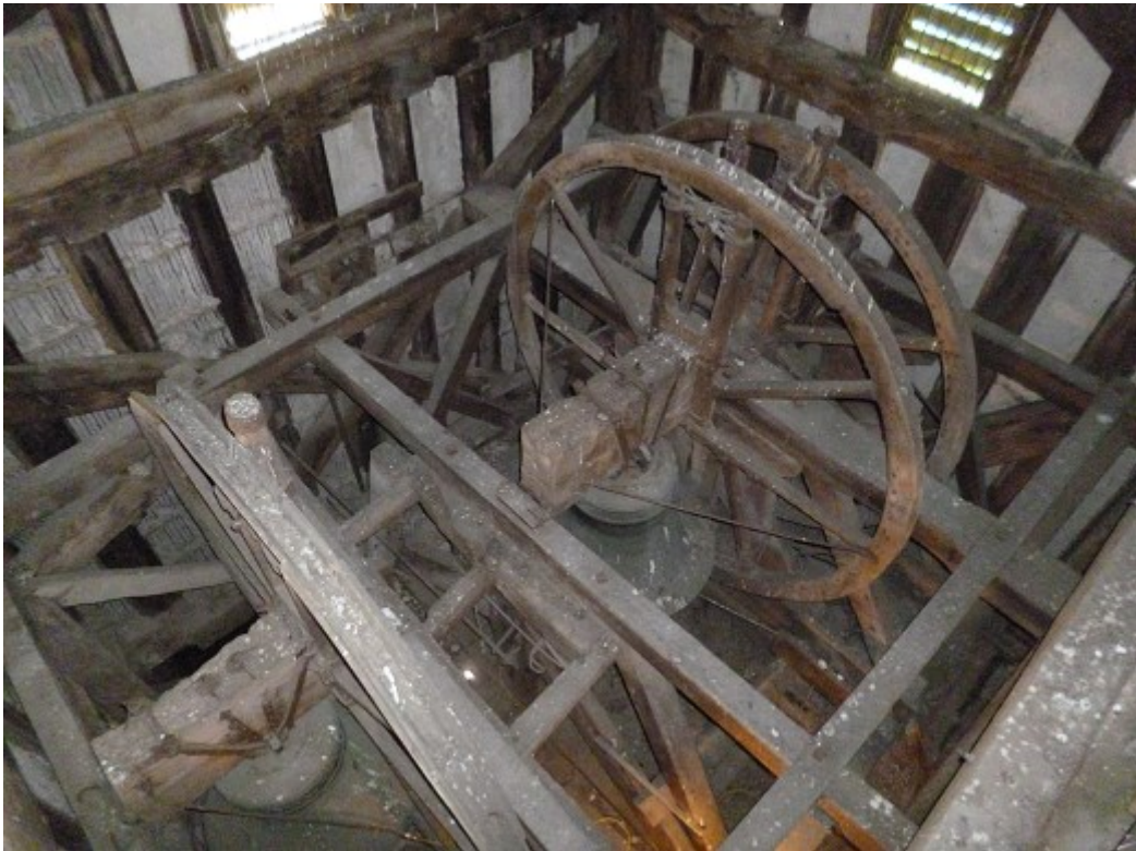
Figure 2c/d: Views of the upper timbers, looking east (top), and the bell frame, looking northwest (bottom)
