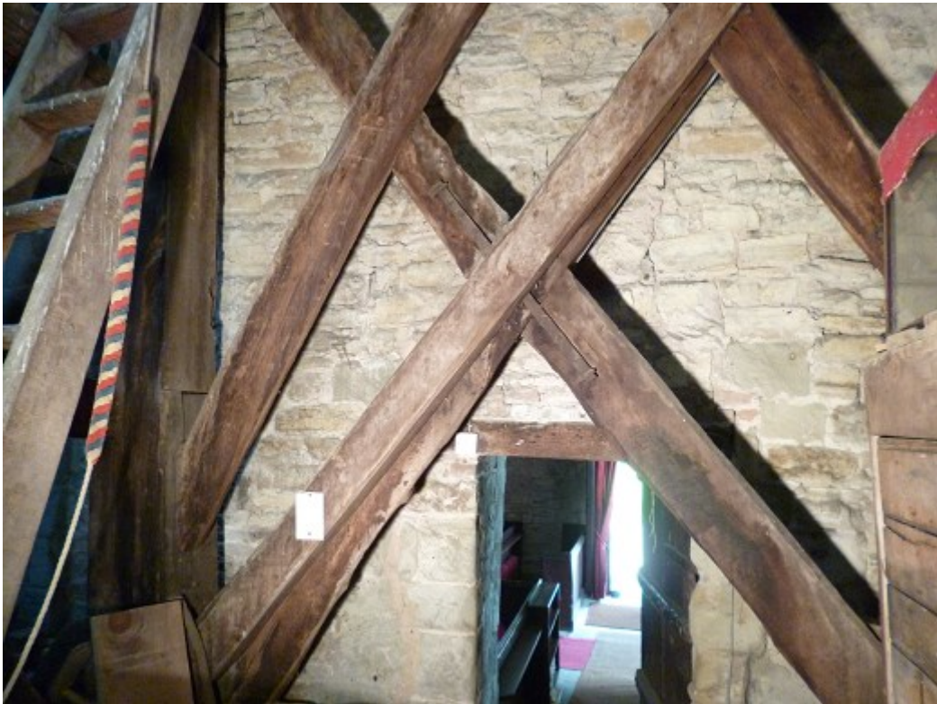
Figure 2a/b: Views of the internal framing of the tower, looking east (top) and south (bottom)
