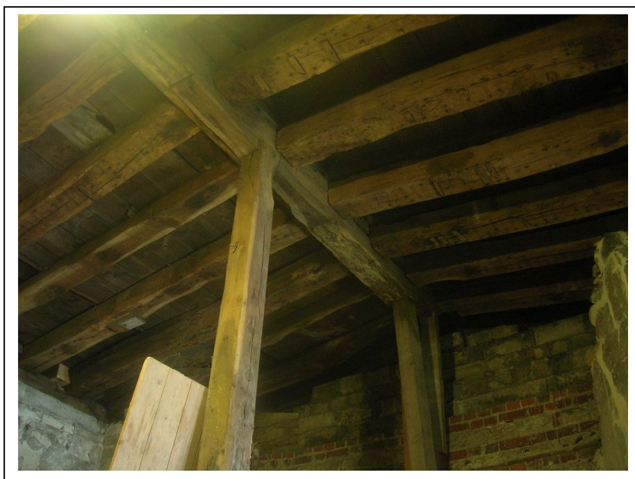
Figure 5a/b: View of St Anselm's Tower, top, and the 'Bakehouse' roof, bottom
