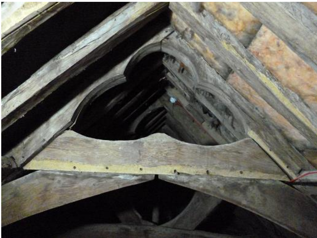
Figure 3a/b: Views of cross-wing roof trusses; closed crown-stud truss (top) and open trefoil cusped truss (bottom)
