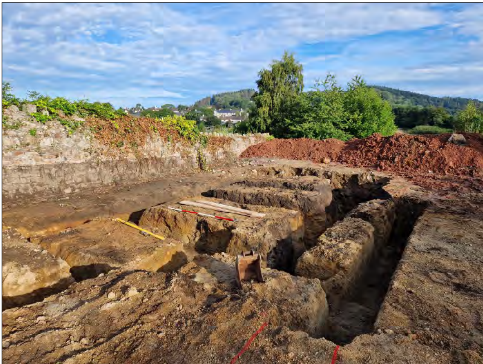
Pl. 7 General view of foundations at northern end of site showing increasing depth of topsoil (1001). 2m scale. Looking northwest.
