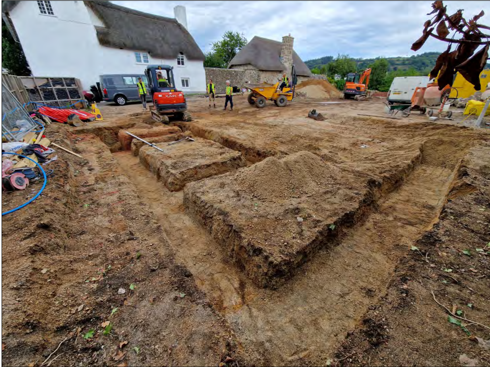
Pl. 5 General view of the trenching at the southern end of the site showing extensive level of truncation associated with the construction of the Greenhill School extension in 1961. Looking northwest.
