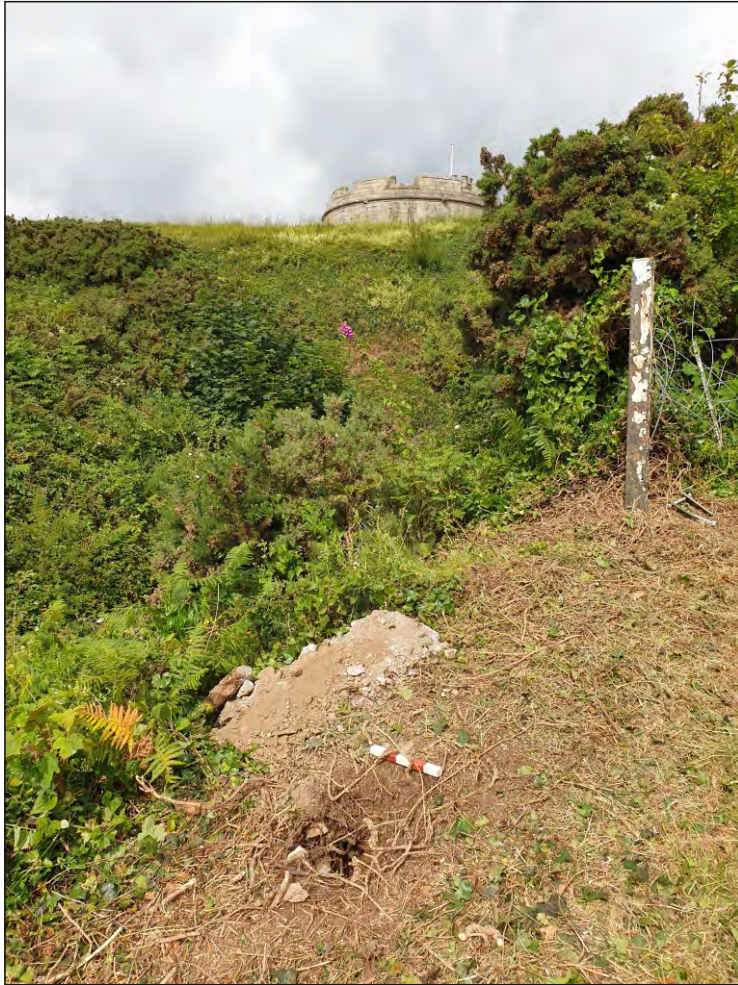
Pl. 1 General view of PH 1 with Pendennis Castle and the late 19th century rebuilt rampart section in the background, and the open passage to the 'bulwark' on Pendennis headland in the foreground. 0.25m scale. Looking west.
