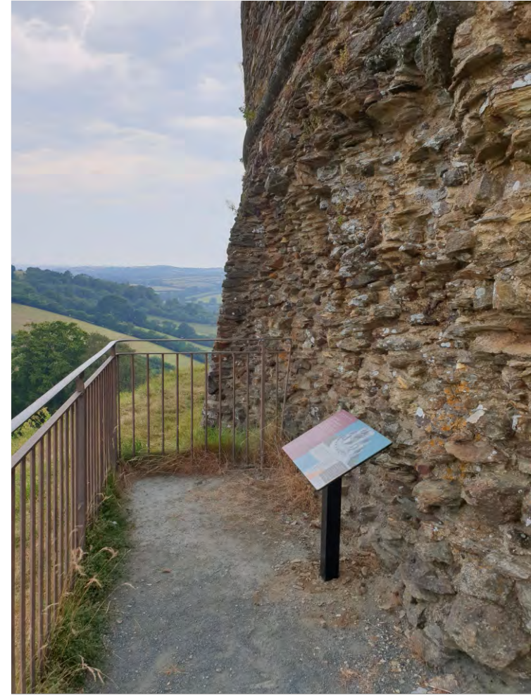
Pl. 2 General view of PH 1 showing position of panel immediately in front of partly robbed exterior face of shell keep. Looking northwest.
