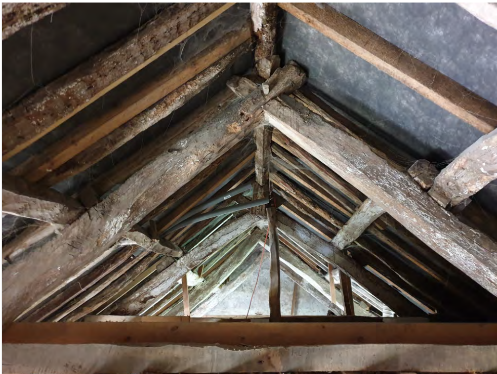
Pl. 14 General view of original main truss construction over the main range. Looking southwest.
