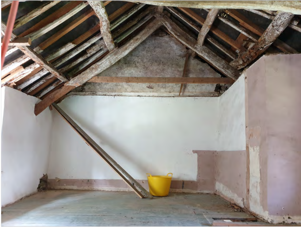
Pl. 13 General view of original main truss construction with two sets of trenced staggered purlins and ridge purlin. Looking southwest.
