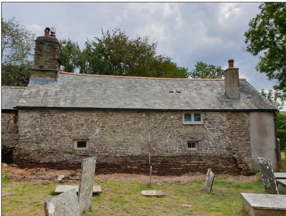
Pl. 1 General view of the rear elevation of Church Cottage showing extent of external groundworks. 2m scale. Looking southeast.
