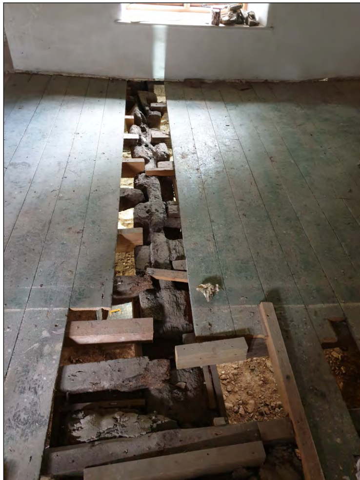
Pl. 8 General view of upper side of beam showing original and later floor joists. Looking southeast.
