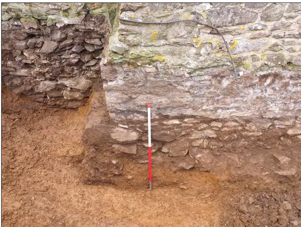
Pl. 6 Close-up of northeast corner of Church Cottage showing foundation (106) sealing two graves. 1m scale. Looking southeast.
