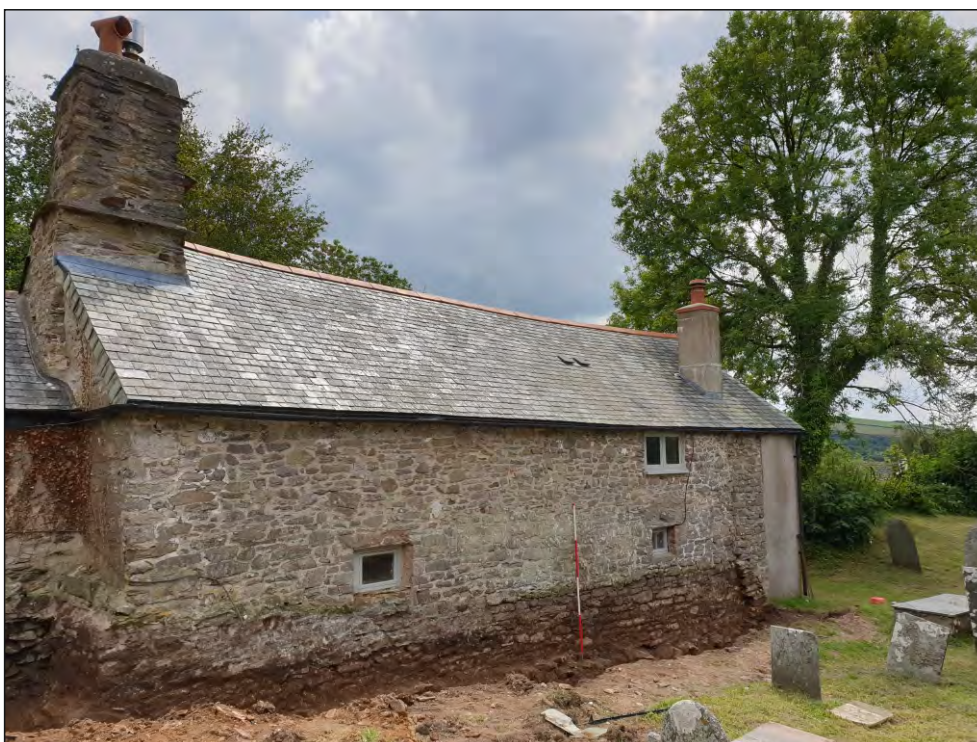
Pl. 2 General view of the rear elevation of Church Cottage showing extent of external groundworks. 2m scale. Looking southwest.
