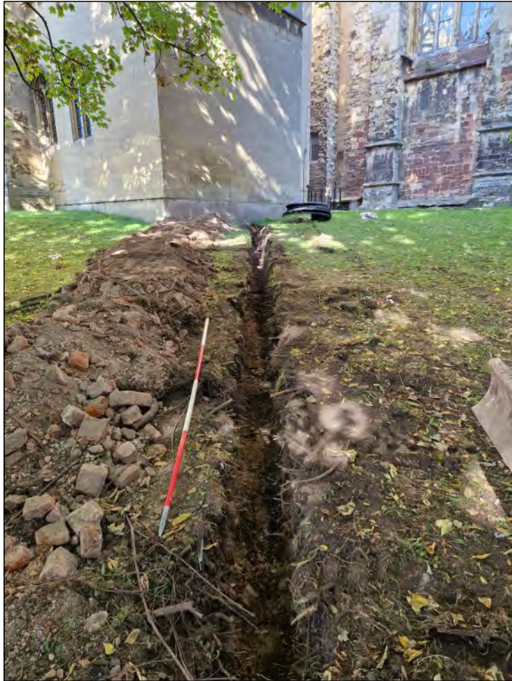
Pl. 3 General view of new service trench showing demolition deposit (105). 2m scale. Looking northwest.
