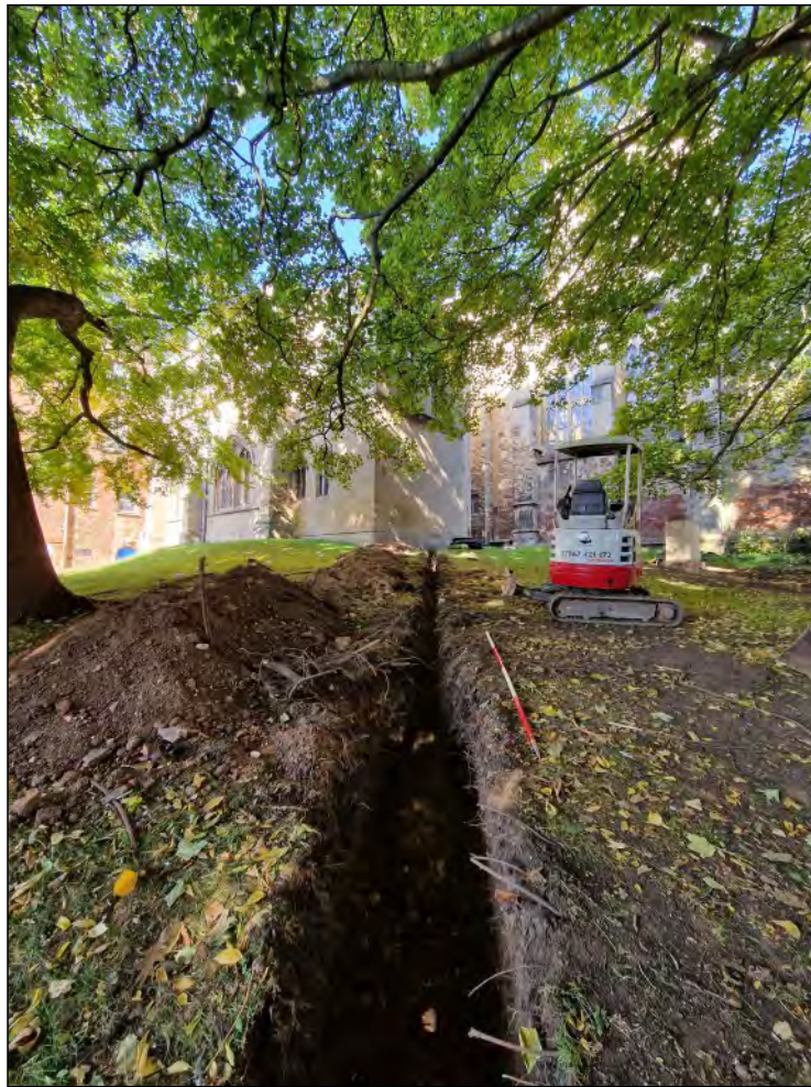
Pl. 1 General view of new service trench showing extensive late 19th century landscaping deposits (103-4). 2m scale. Looking northeast.
