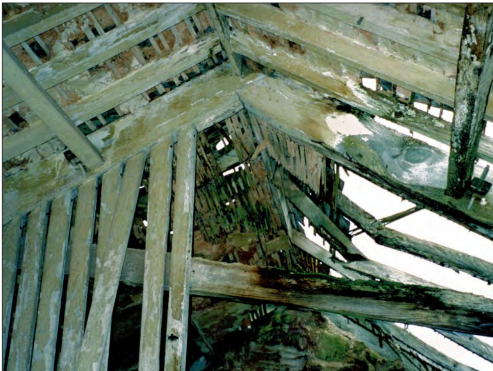
Pl. 14 General view of the roof structure at the southern end showing possible evidence for torching between the rafters. Looking northwest.
