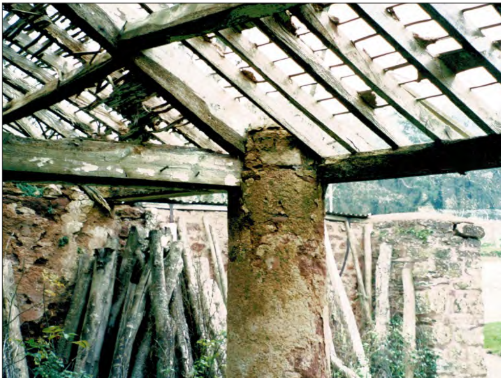
Pl. 12 Close-up of cylindrical pier showing details of the roof construction and tie-beam. Looking northeast.
