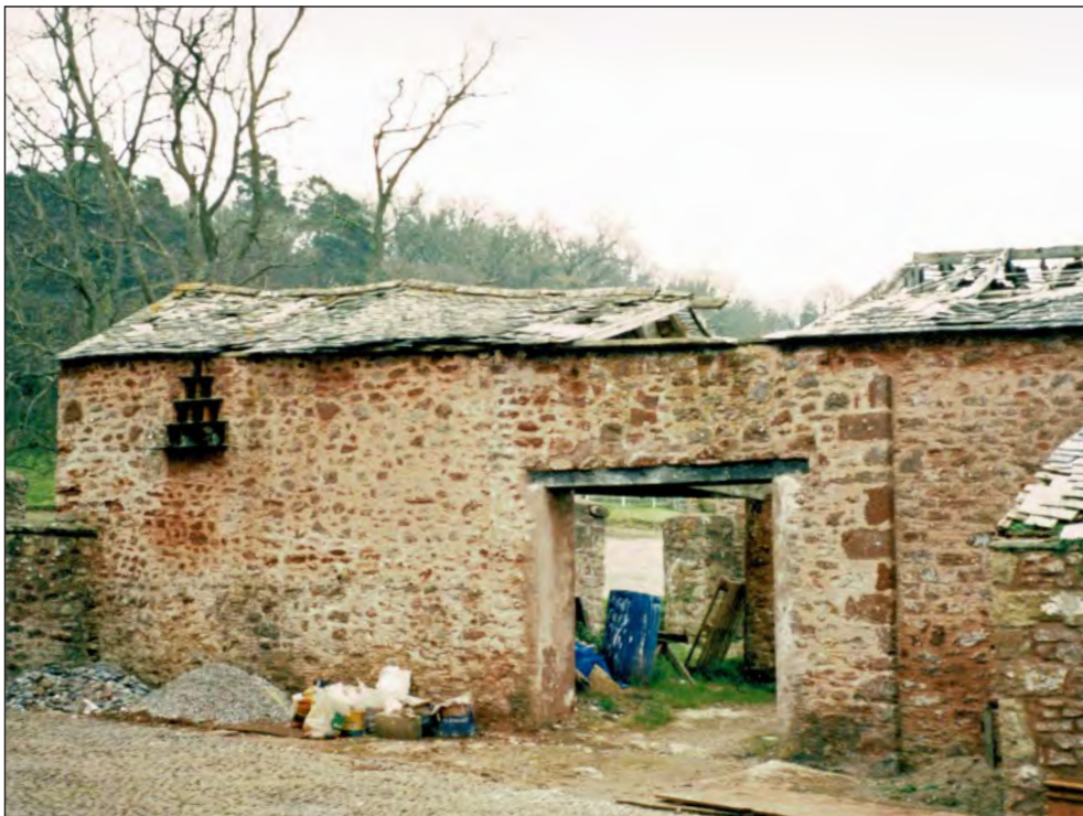
Pl. 10 General view of the former linhay prior to the demolition of the roof structure from the stable yard to the west. Looking northeast.
