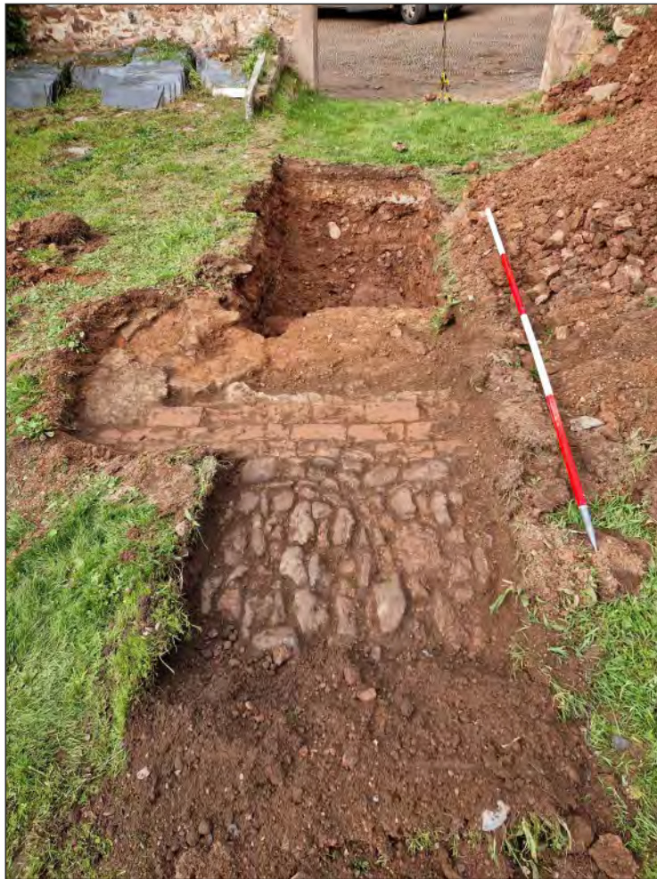
Pl. 27 General view of Trench 2 showing cobbled yard surface (206), brick drain (208), pier foundation (205) and concrete floor (209). 2m scale. Looking northwest.
