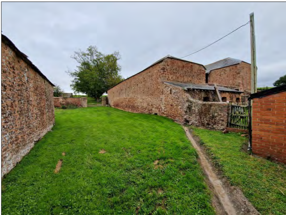
Pl. 16 General view of the stock yard showing the coach house (left), the pig buildings (right foreground), stable and bank barn (background). 2m scale. Looking northeast.
