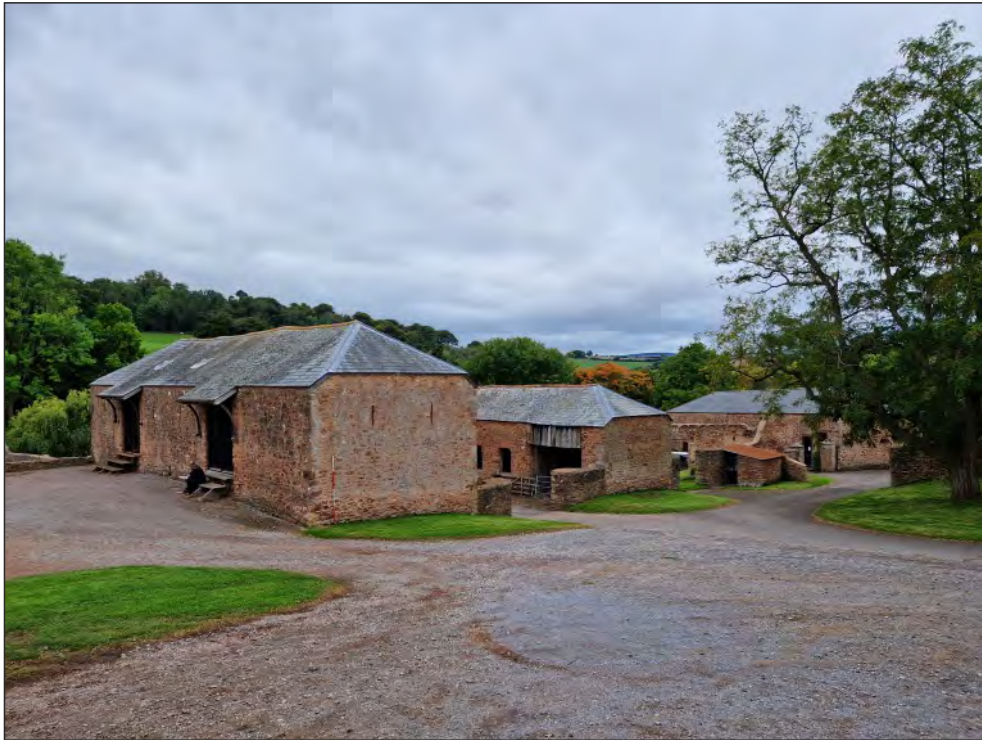
Pl. 1 General view of the bank barn, the former stables, linhay and formal stables. 2m scale. Looking southwest.
