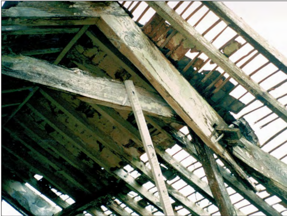
Pl. 13 General view of the roof structure showing possible evidence for torching between the rafters.
