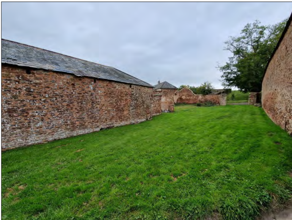
Pl. 8 General view of the stock yard with the linhay in the background. 2m scale. Looking northwest.
