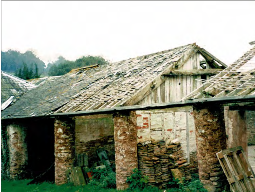
Pl. 9 General view of the south end of the former linhay prior to demolition showing the cylindrical piers and roof structure. Looking southwest.
