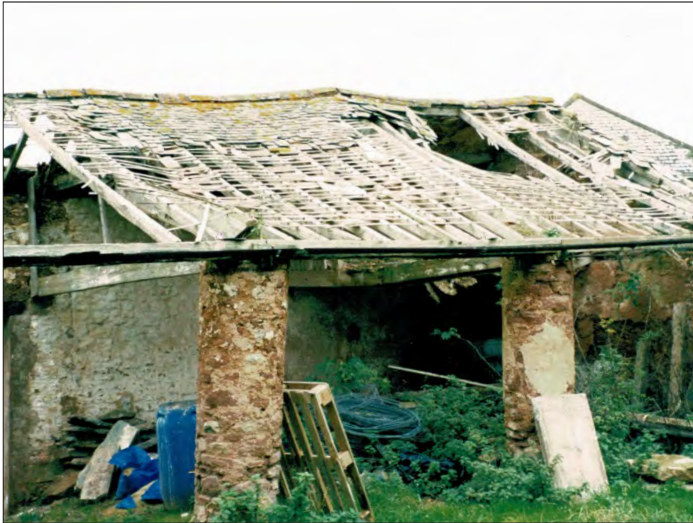
Pl. 11 General view of the north end of the former linhay prior to demolition showing the cylindrical piers and roof structure. Looking northwest.
