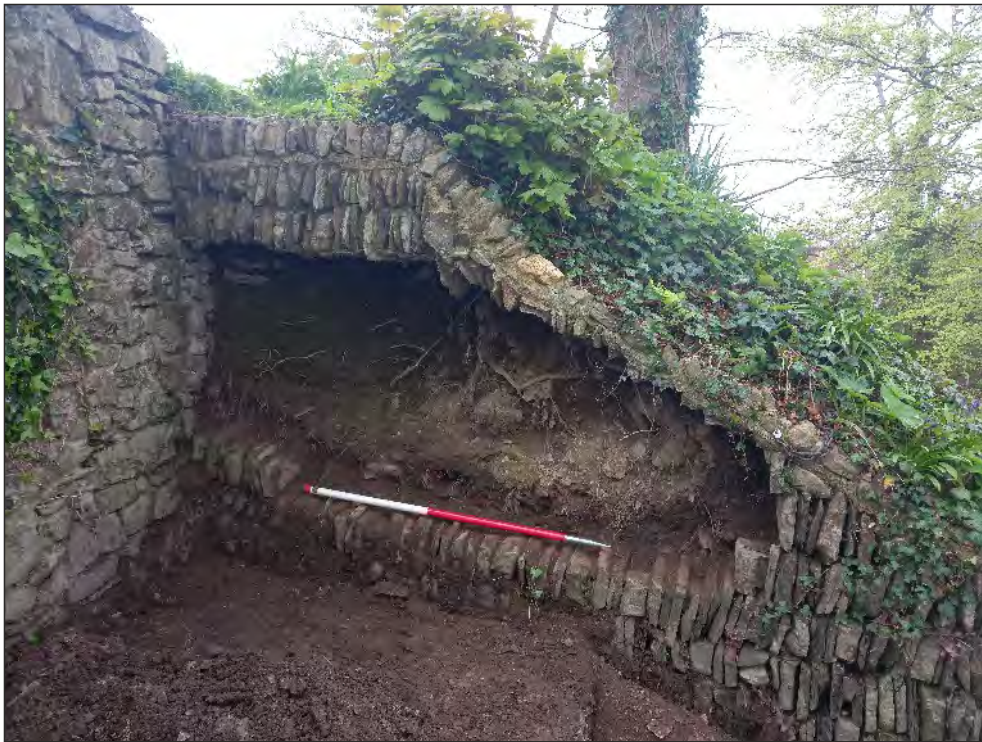
Pl. 9 General view of damaged retaining wall. 1m scale. Looking southwest.
