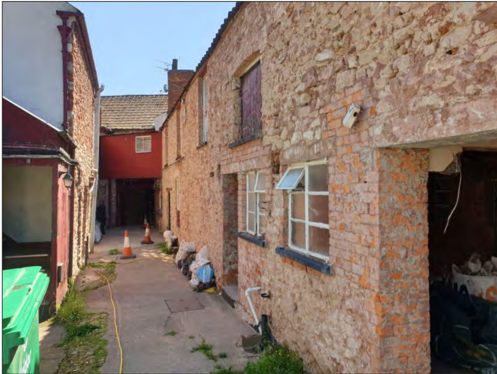
Pl. 35 General view of the north end of the west range rebuilt in the 20 th century with openings with concrete lintels and metal Crittall window frames. Looking southwest.
