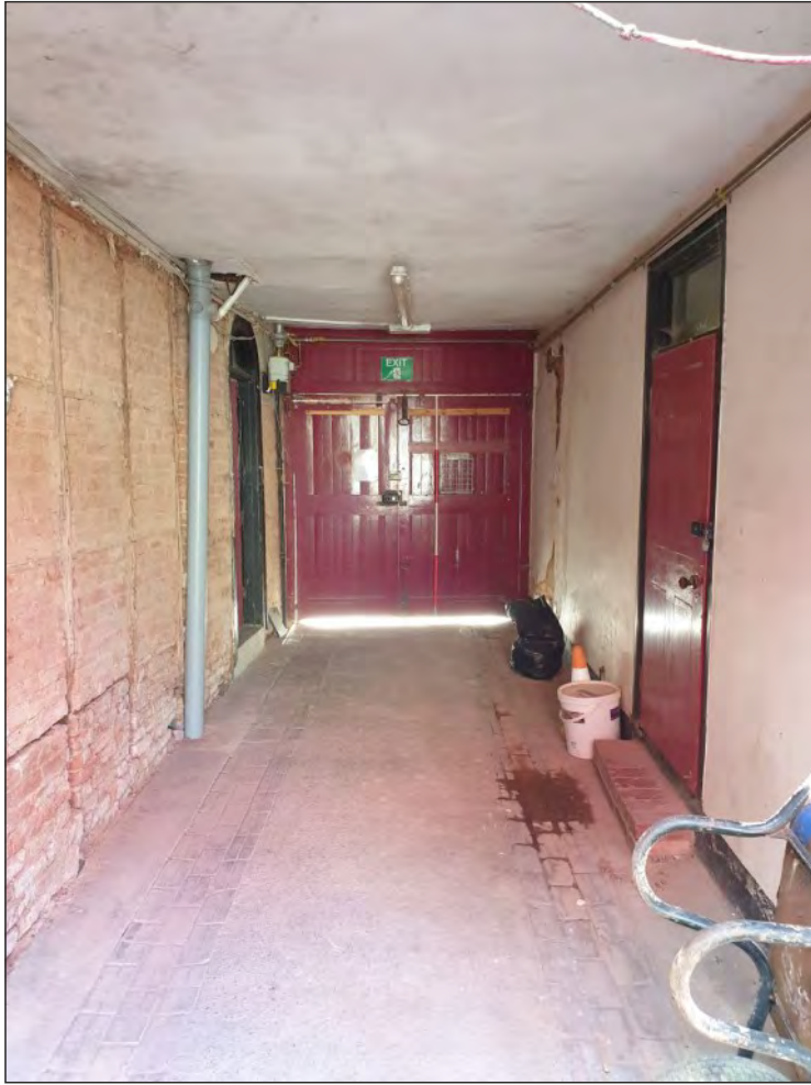
Pl. 5 General view of the carriageway through the south range of the building with the 19th- or early 20th-century double doors at its south end. 2m scale. Looking southwest.
