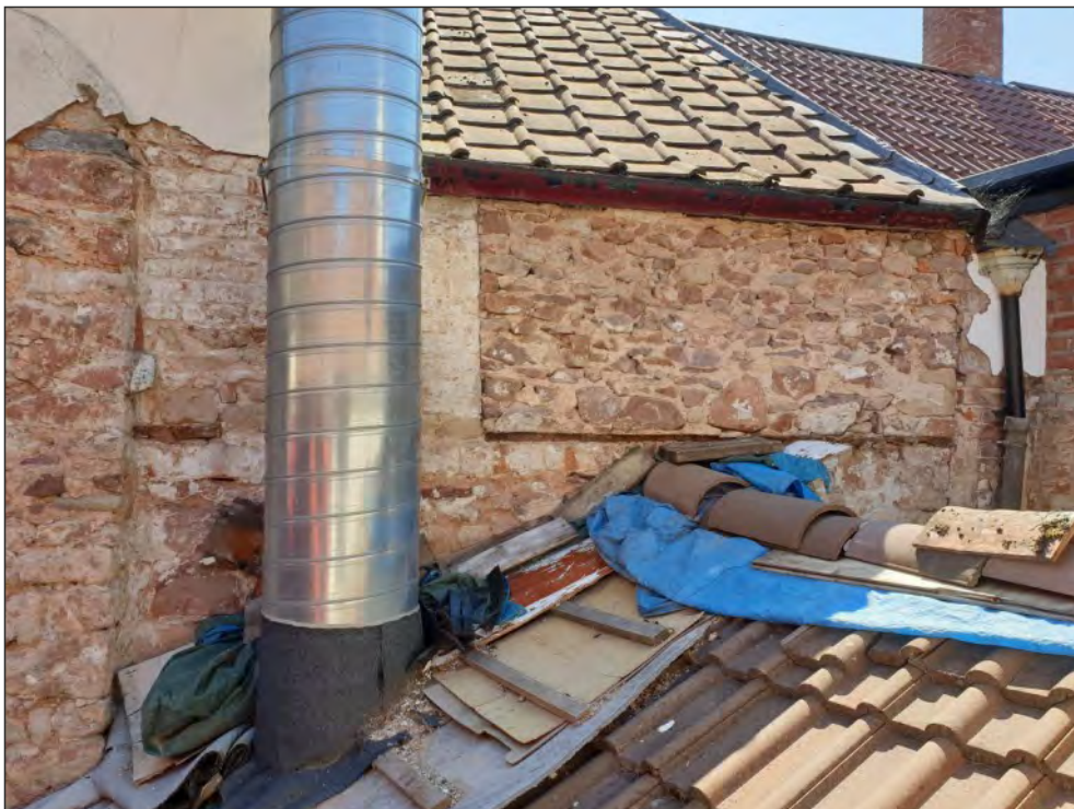
Pl. 4 General view of blocked window (right) and coping stone on west side of chimneystack (centre left). Looking southwest.
