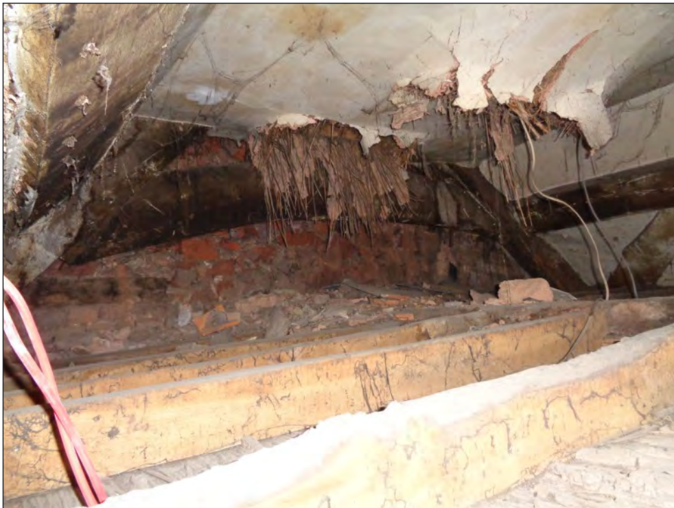
Pl. 22 General view of A-frame end truss without arch bracing and with a high, cranked collar. Looking southeast.
