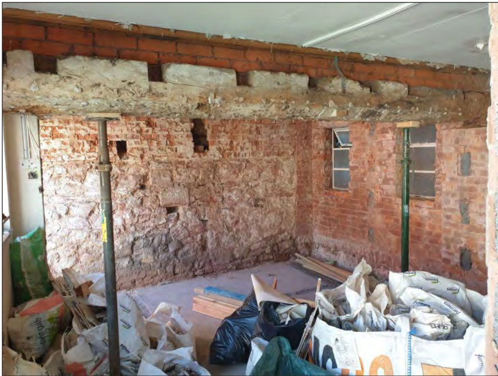
Pl. 38 General view of the principal beam supporting the first floor with chamfered undersides and deep housings for substantial joists. Looking southwest.
