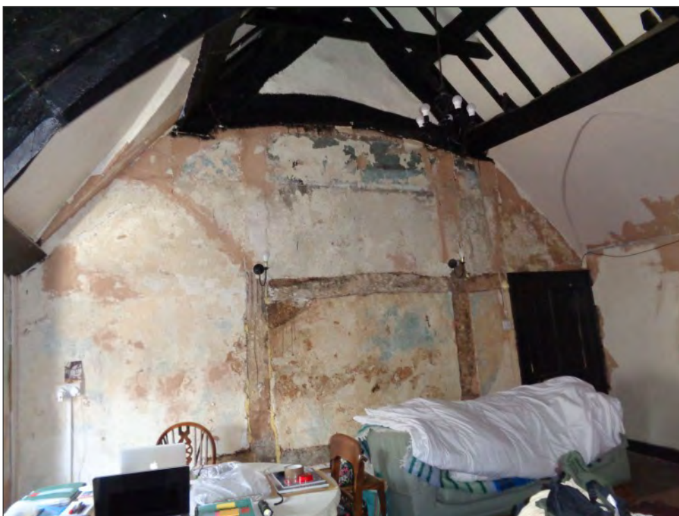
Pl. 16 General view of the full height timber and plaster partition on the west side of room F02. Looking northwest.
