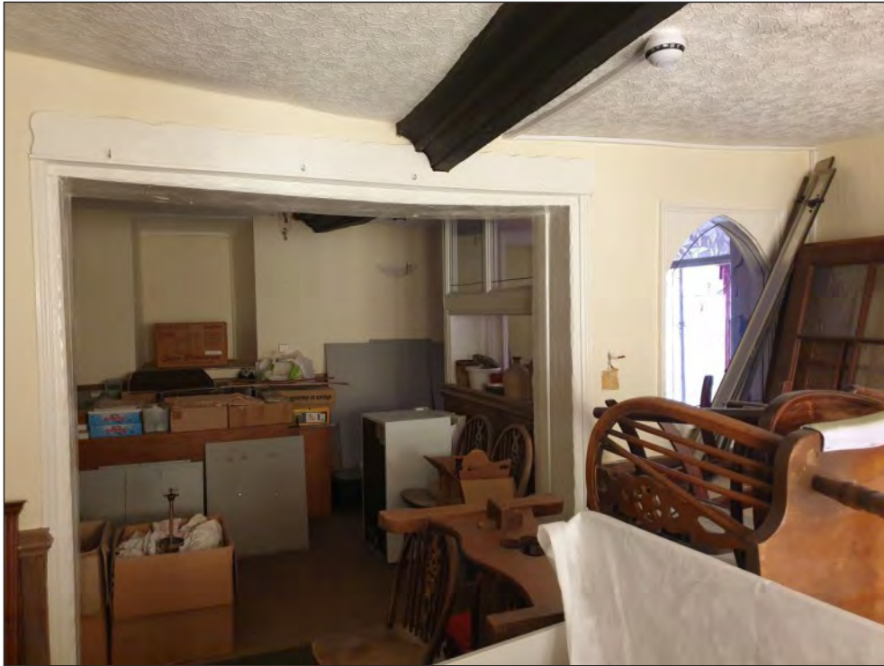
Pl. 9 General view of the western room (G05) divided by a central spine wall containing a flat arch and a 'gothick' arch, and by a subsidiary screen forming a glazed porch within the door to the carriageway. Looking northeast.
