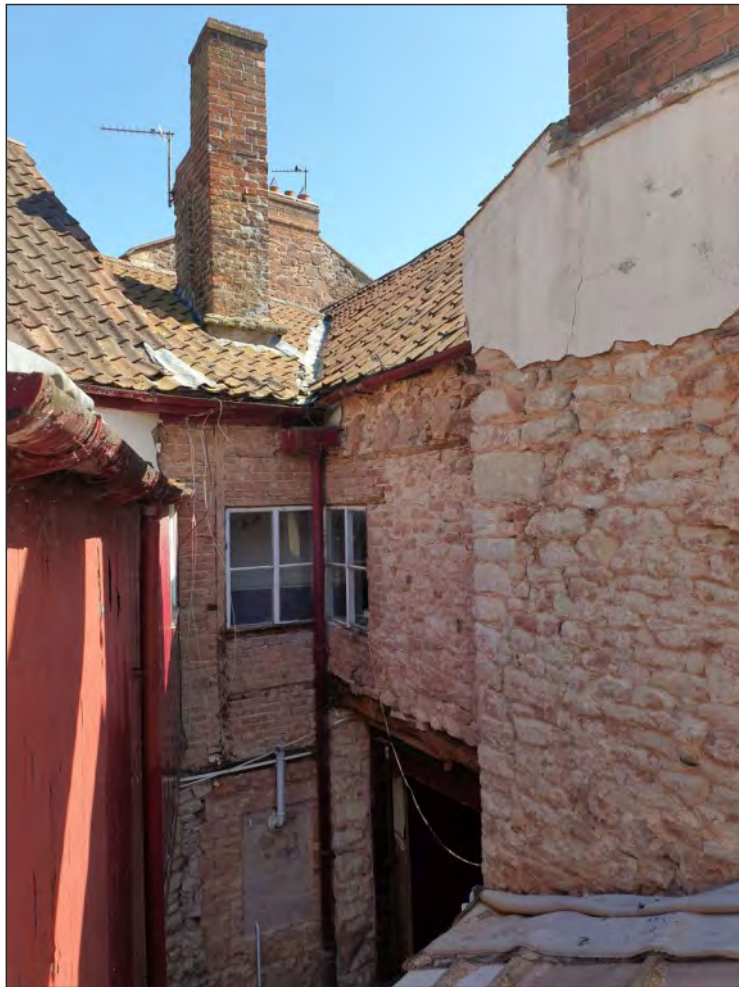
Pl. 3 General view of the rear elevation of the south range showing raised wall level. Looking southeast.
