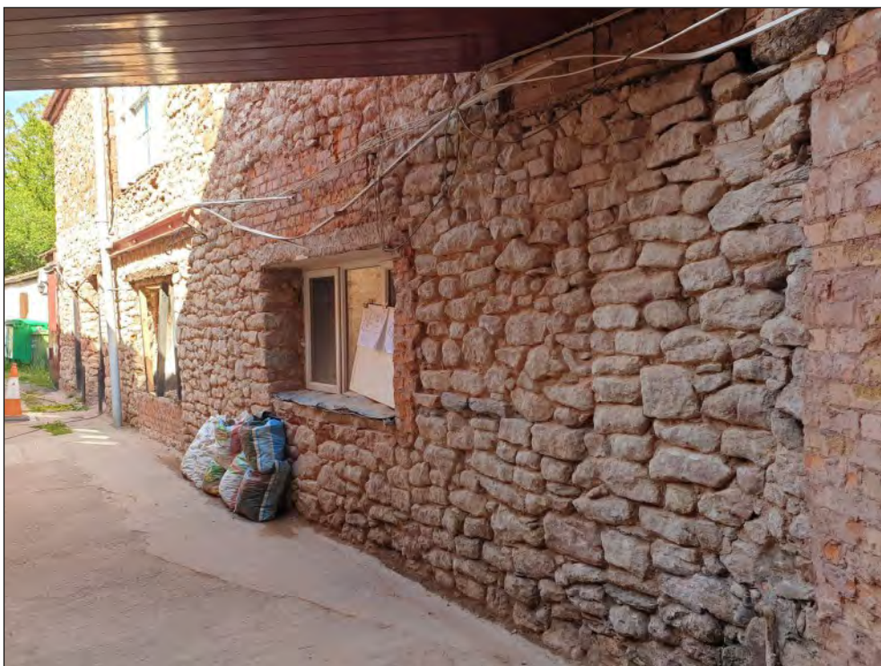
Pl. 26 General view of the west elevation of the east range with the late 19 th - or early 20 th -century enclosure, at ground-floor level, of the western part of the small courtyard between the chimneystacks, visible to the right. Looking northeast.
