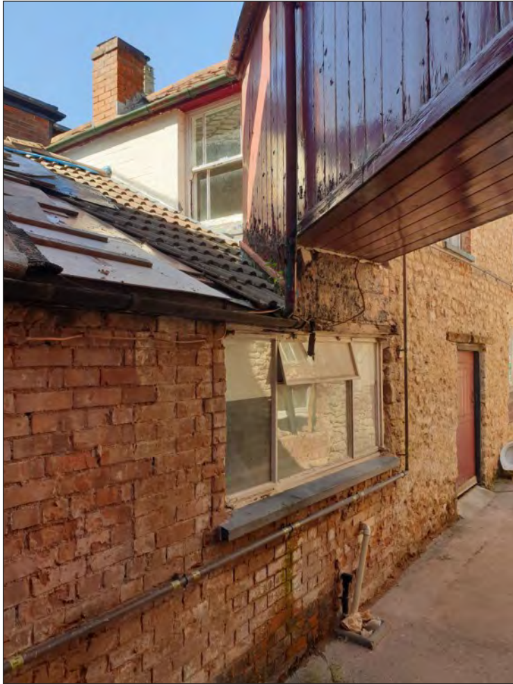
Pl. 33 General view of the late 19 th -century single-storey brick infill at the south end of the north range containing openings blocked the late 19 th or early 20 th century. Looking north.
