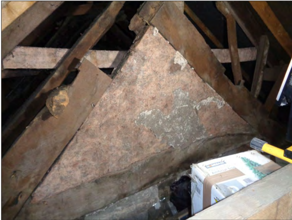
Pl. 19 Close-up of cranked collar and without arch braces, with intact plaster infilling. Looking northwest.
