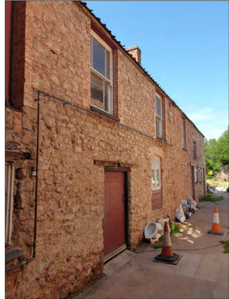
Pl. 34 General view of the east elevation of the west range showing rebuilt upper elevation. Looking north.
