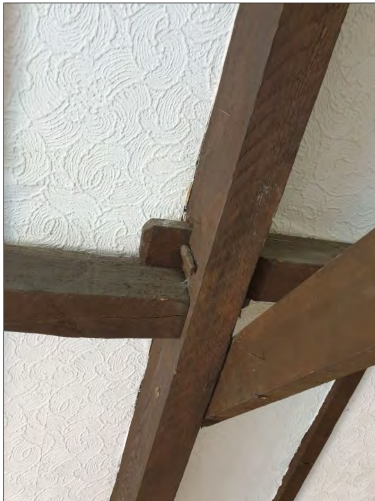
Pl. 40 Close-up of the late 19th century roof structure in F18 with staggered butt purlins secured within the principals by pegs. Looking southeast.
