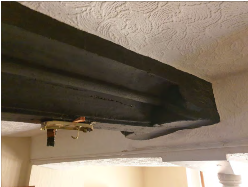
Pl. 10 Close-up of the ceiling beam showing deep hollows and a central moulded fillet on each side. The stops at the south end of the beam are convex run-out stops of a type typical of the early 16 th century. Looking south.
