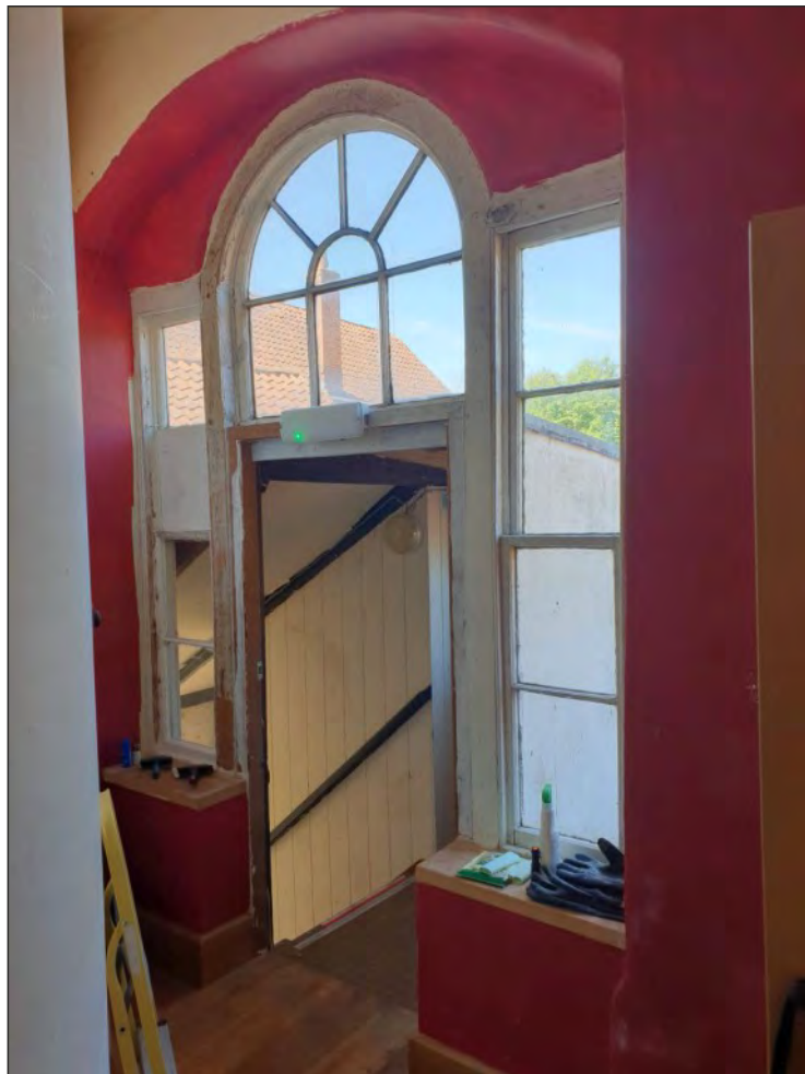
Pl. 32 Close-up of the 'Venetian' window at the north end of the former assembly rooms. Looking northwest.
