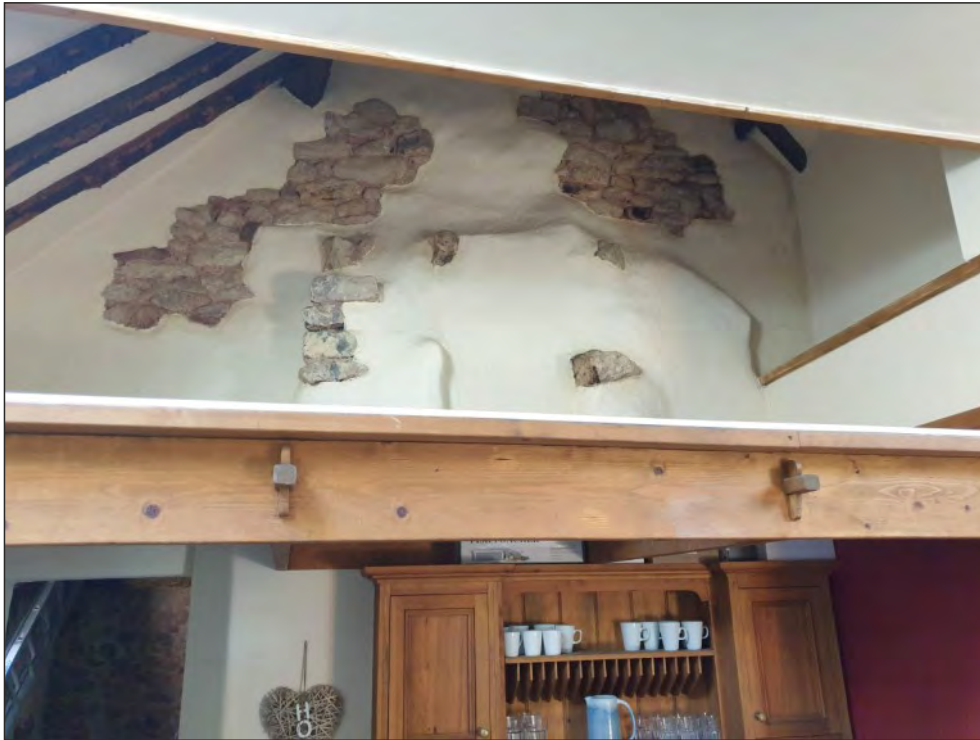
Pl. 31 General view of the south wall of the earlier building showing the remains of a tall, tapering hood of a very large fireplace and chimneystack extending to full height of the gable. Looking southwest.
