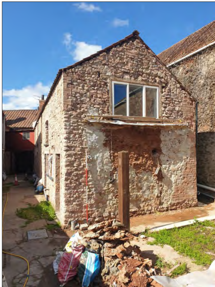
Pl. 36 General view of the north elevation of the north range showing the large area of cob walling forming the centre of the gable end. 2m scale. Looking southwest.
