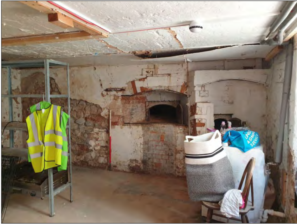
Pl. 37 General view of the mid- to late 19th century oven in room G15. 1m scale. Looking north.
