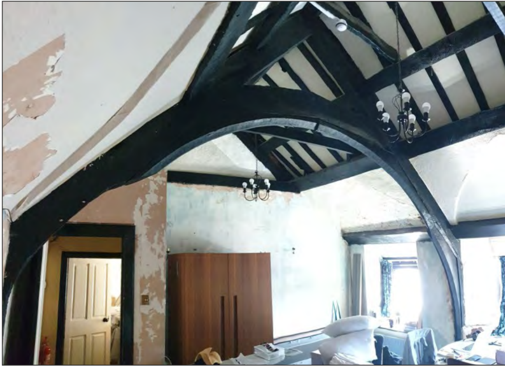
Pl. 21 General view of the single medieval roof truss supported by chamfered upper and lower arch braces and with a high, cranked collar. There are three levels of purlins, the lower sets being linked by curved, flat wind braces, and a very large, diagonally-set ridge tree. Looking southeast.
