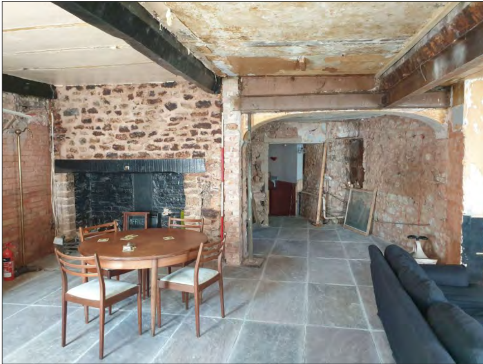
Pl. 13 General view of heavily rebuilt fireplace in north elevation of room G01, with wide archway into the adjacent trapezoidal room G06 to the right. 2m scale. Looking northeast.
