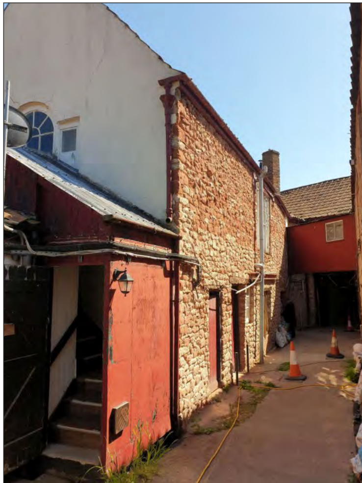
Pl. 28 General view of the north wall of the east range, with the 'Venetian' window partly obscured by a relatively modern external stair, probably a fire escape. Looking south.
