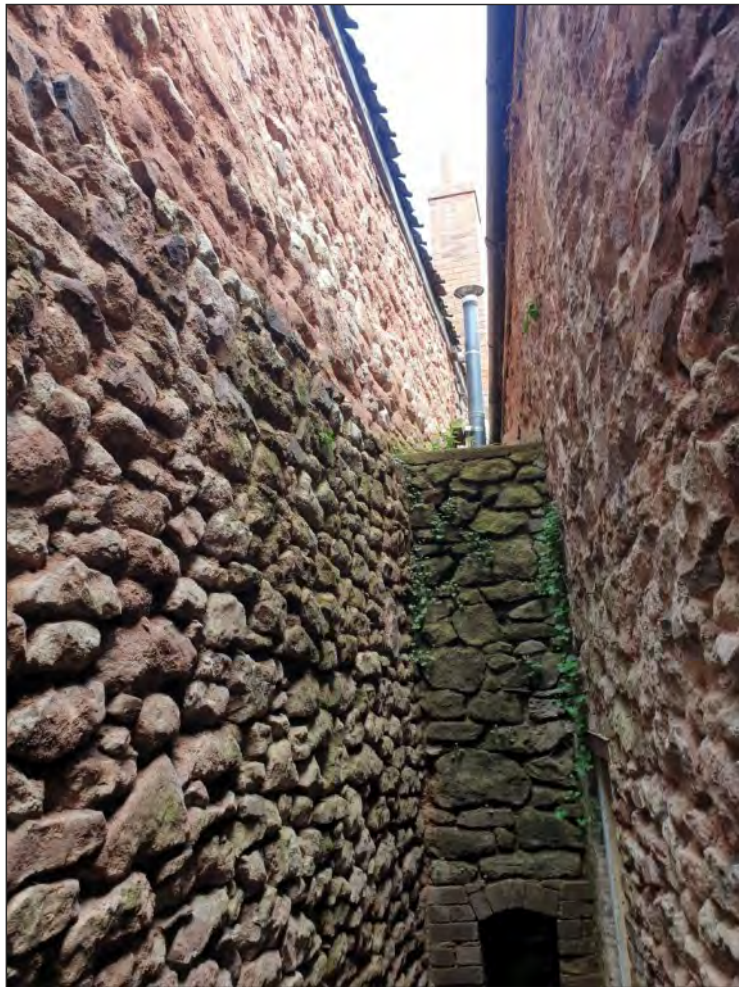
Pl. 25 General view of the very narrow passage between the east range and the adjacent building. Looking northeast.
