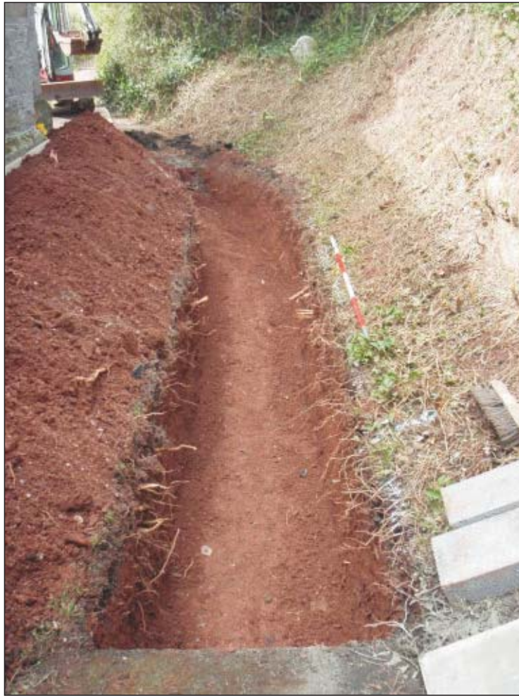
Pl. 1 General view of new foul drain and soakaway. 2m scale. Looking west.
