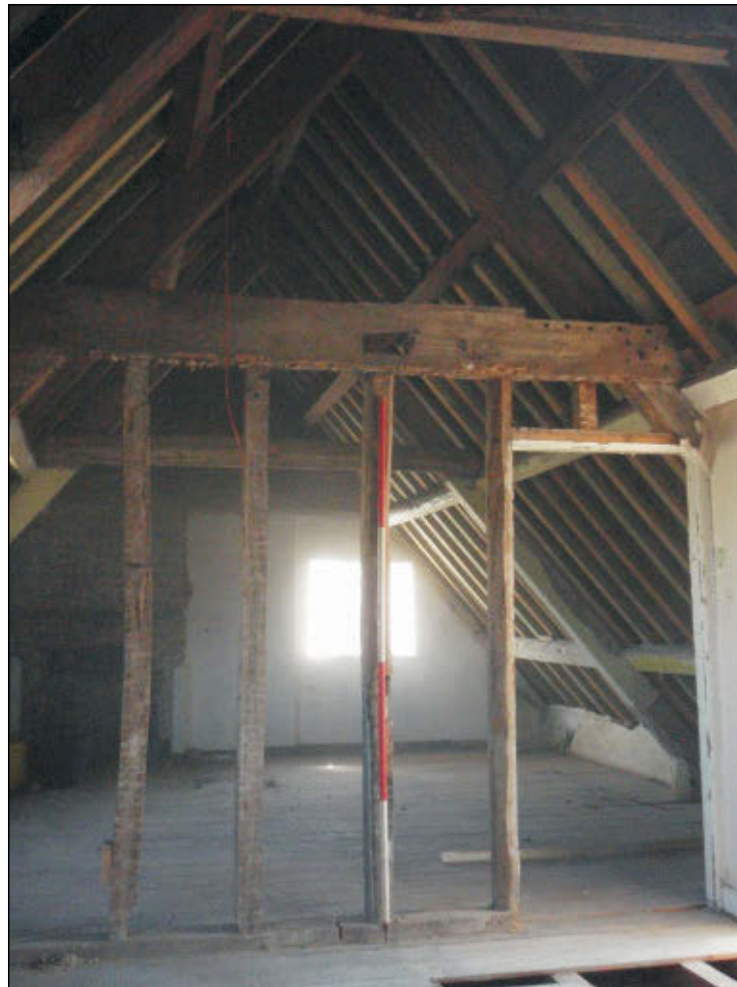
Fig. 15 Second floor, main house showing typical 18th century partition and roof truss.
