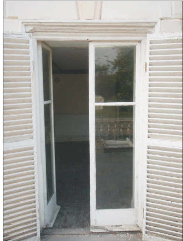
Pl. 6 Close-up of ground floor rear door showing earlier door lintel. Looking southeast.
