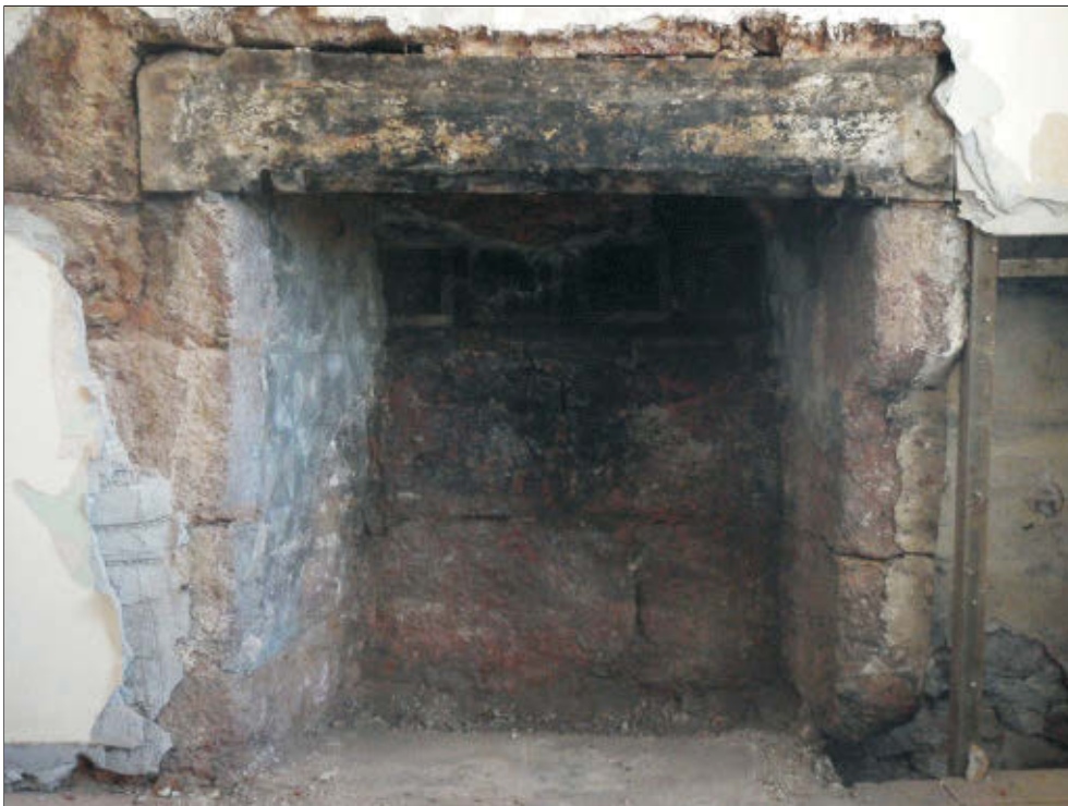
Pl. 10 General view of first floor C17th sgraffito fireplace with decorated wooden lintel. Looking southwest.
