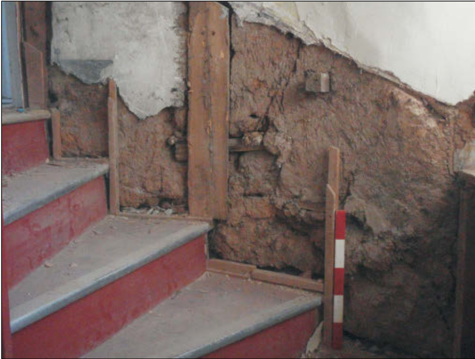
Pl. 9 Close-up of earlier stairs leading to first floor. 0.5m scale. Looking northeast.
