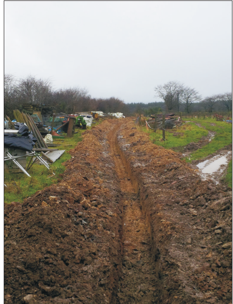
Pl. 2 General view of cable trench from farmyard showing modern made ground in foreground. Looking southwest.
