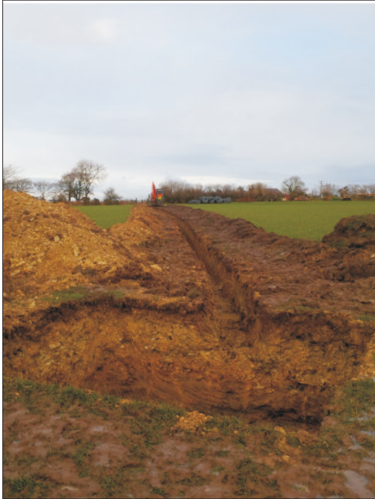
Pl. 1 General view of wind turbine foundation showing depth of topsoil (100) and underlying natural subsoil (101). Looking northeast.
