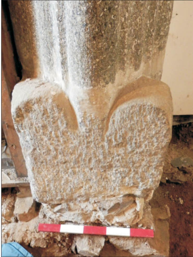
Pl. 11 Arcade: Close-up of western pillar base and foundation. 0.5m scale. Looking west.
