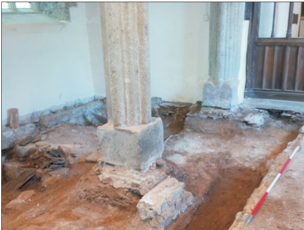
Pl. 2 General view of north aisle and arcade foundations. 2m scale. Looking northeast.
