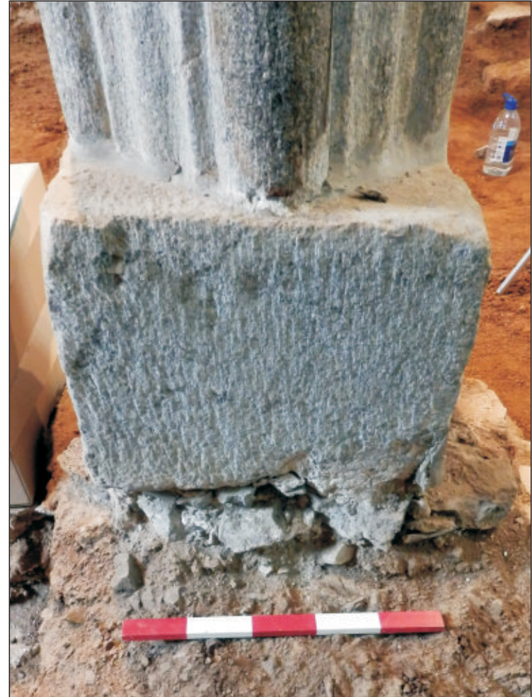
Pl. 12 Arcade: Close-up of central pillar base and foundation. 0.5m scale. Looking west.
