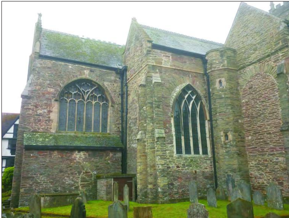
Pl. 2 General view of exterior north chancel wall showing small blocked window. Looking south.
