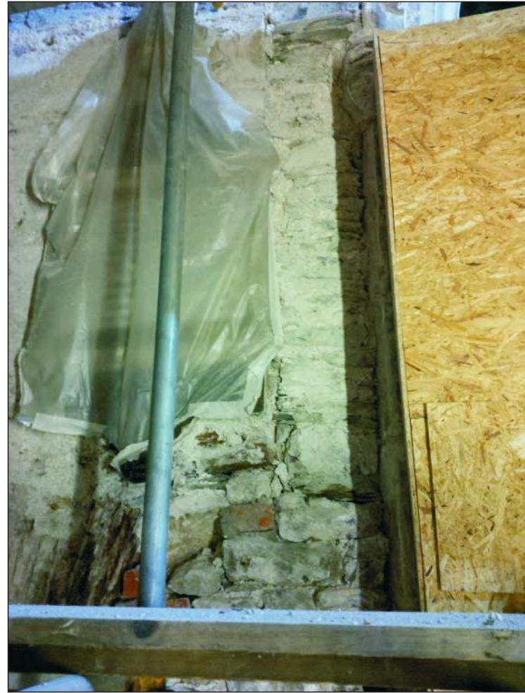
Pl. 4 Close-up of building break in south chancel wall. Looking southwest.
