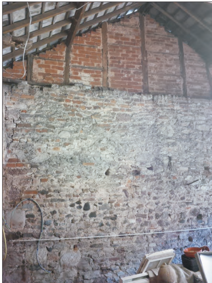
Pl. 20 Detail of west end elevation showing detail of masonry and rebuilding of gable.
