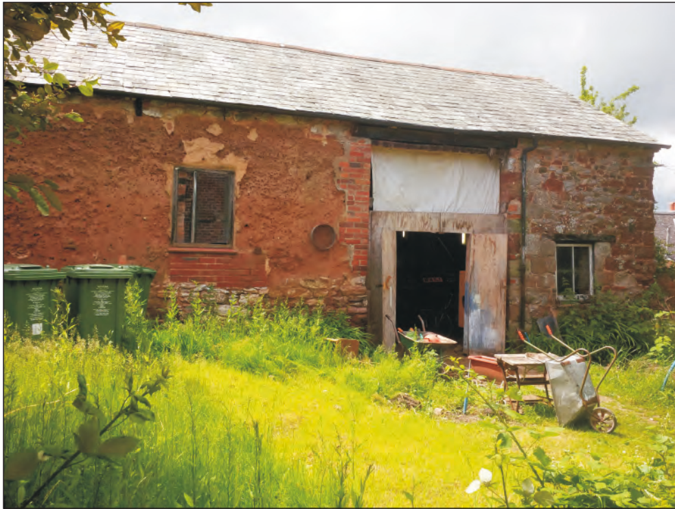
Pl. 3 General view of north elevation showing extensive 19th century rebuilding of west end (right).
