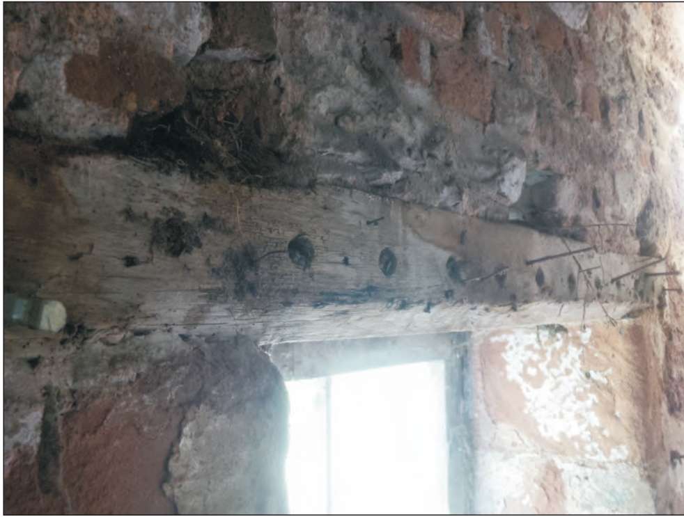
Pl. 19 Detail of timber lintel with stepped run-out stop and 12 holes for rod laths.
