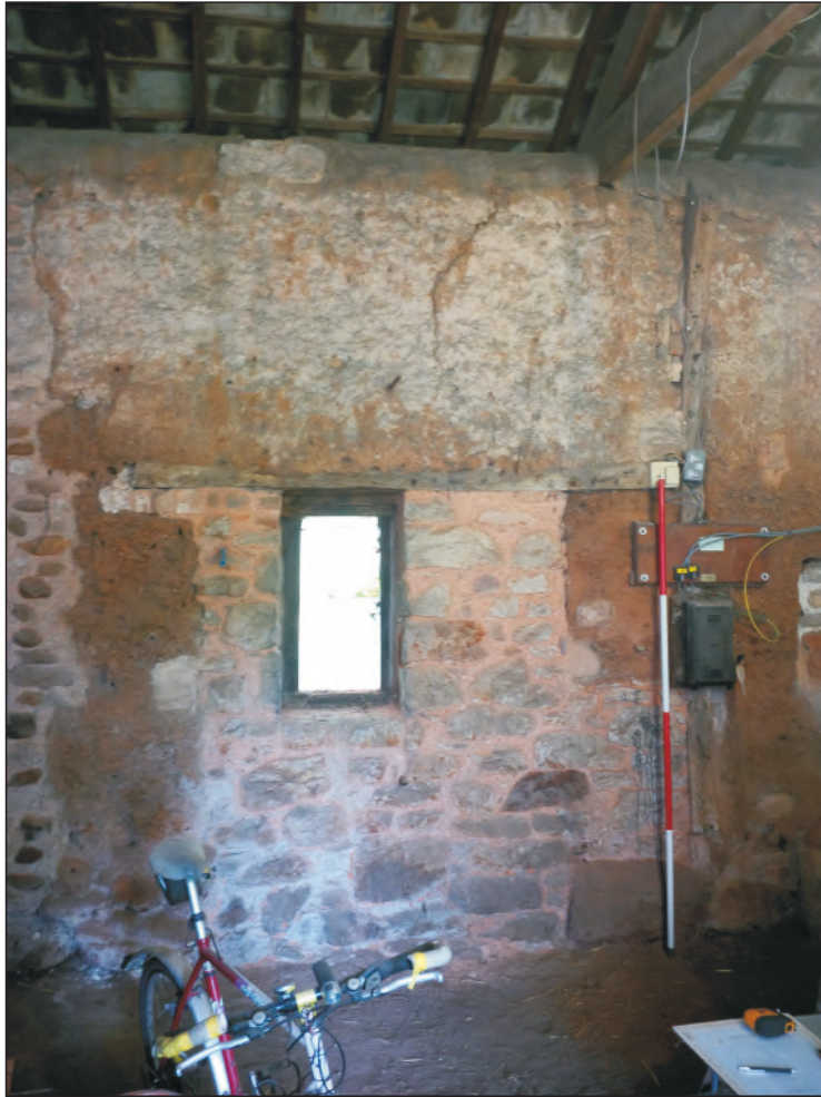
Pl. 13 Detail of south elevation showing blocked doorway and sawn-off cruck (right).
