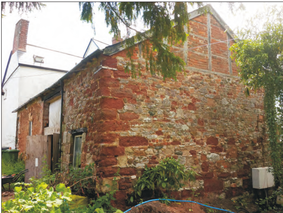
Pl. 4 Detail of west end elevation showing detail of masonry and rebuilding of gable.
