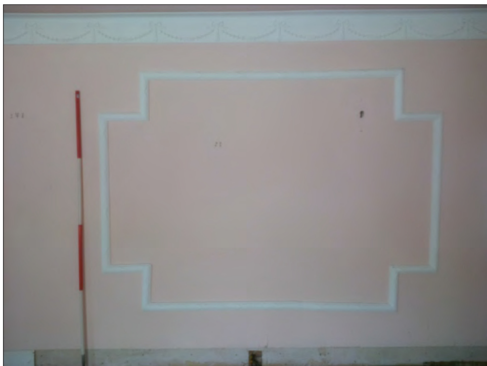
Pl. 12 General view of reed and ribbon decorated plaster panel moulding and swag and bow decorated cornice. 2m scale. Looking east.
