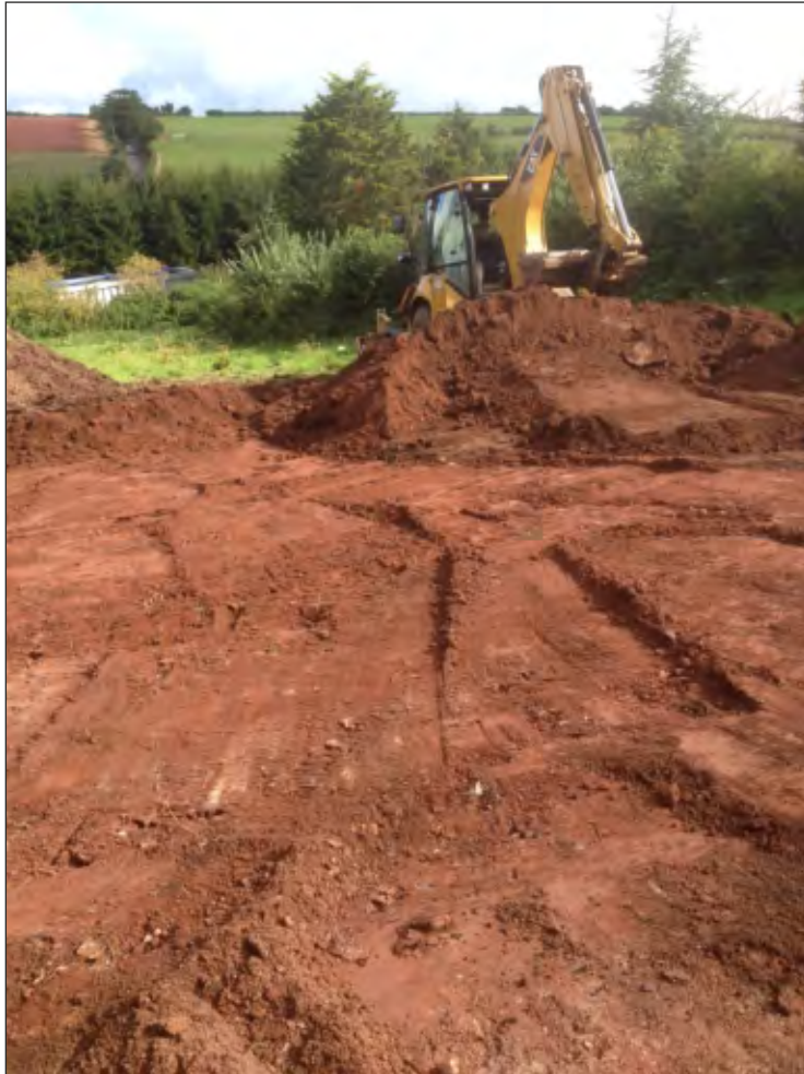
Pl. 1 General view of site showing depth of excavations and exposed subsoil (101). Looking northeast.
