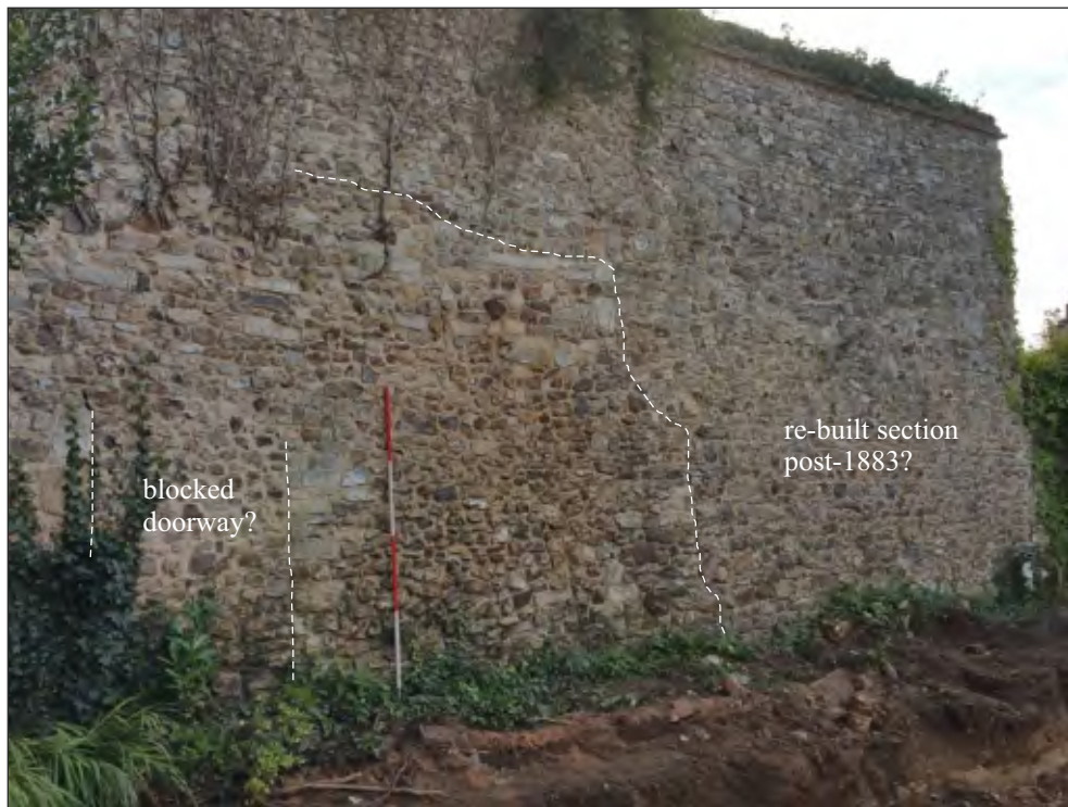
Pl. 8 General view of eastern boundary wall showing blocked doorway (left) and area of rebuilding (right). 2m scale. Looking southeast.
