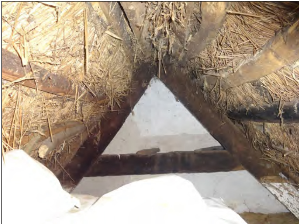
Pl. 24 View of the roof over the parlour wing, looking east, showing smoke blackened trusses of probable 17th-century date.
