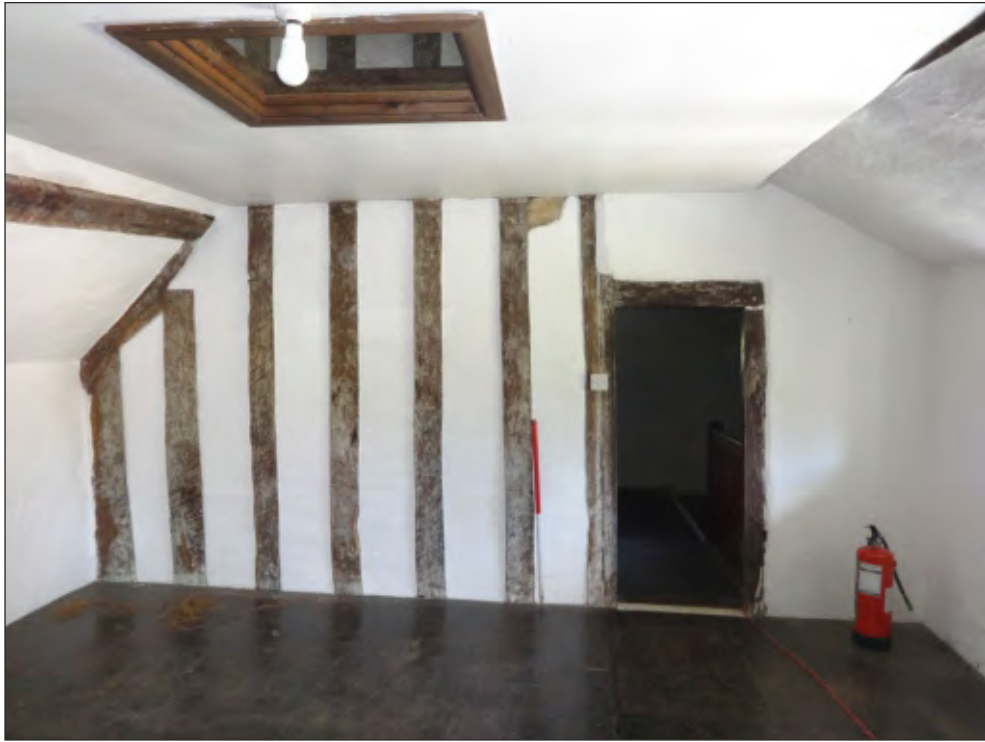
Pl. 17 View of the hall chamber showing the stud partition separating the room from the upper part of the inner room. 1m scale. Looking north.
