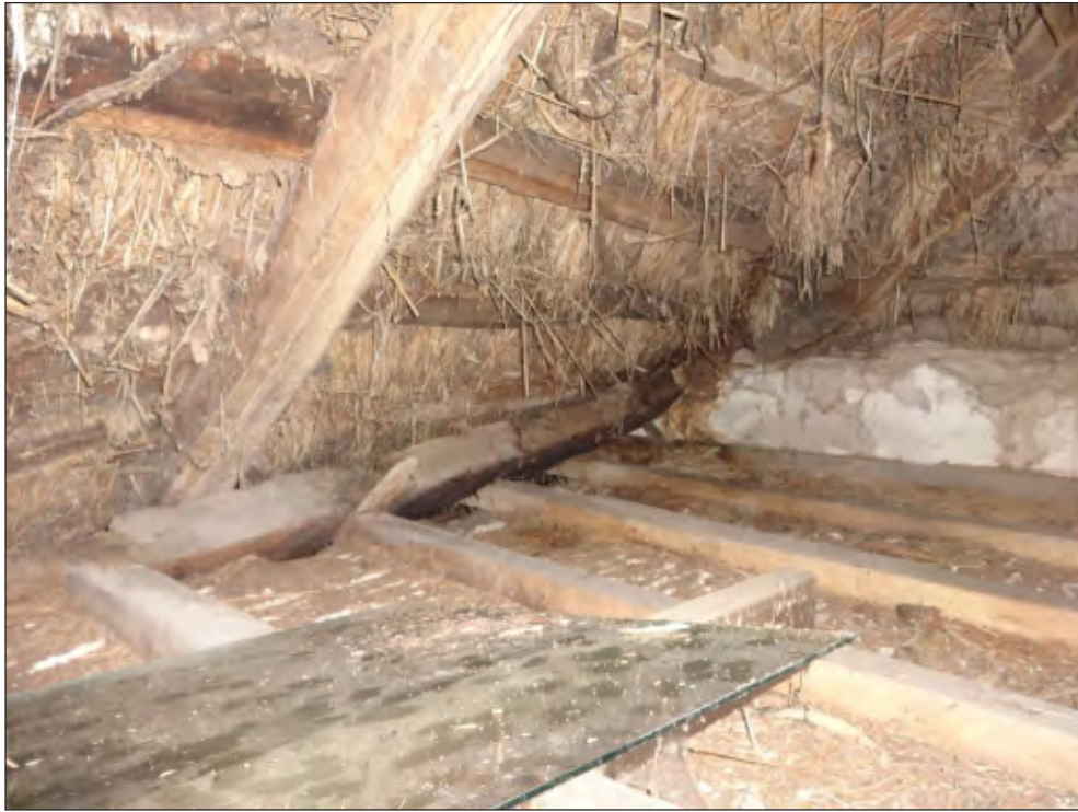
Pl. 23 The northern end of the roof, looking north, showing a smoke blackened purlin over the inner room.
