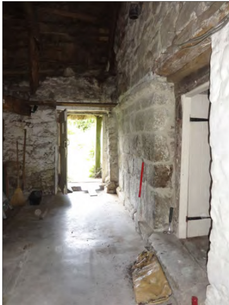
Pl. 8 View of the cross passage following the demolition of the modern partition, showing the granite ashlar of the inserted chimney. 1m scale. Looking west.
