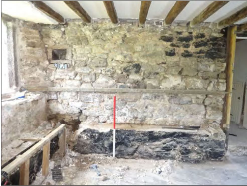
Pl. 7 View of the north end of the hall following the demolition of the modern bench. 1m scale. Looking north.
