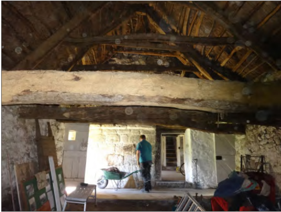
Pl. 15 View of the shippon following the demolition of the modern partition. Looking north.
