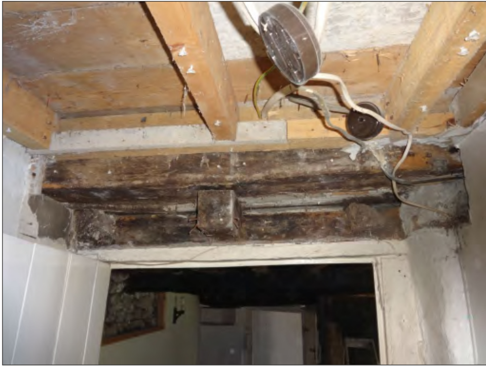
Pl. 3 Detail of the jetty over the doorway from the inner room to the hall, showing alternating long and short joists beneath the jetty. Looking south.
