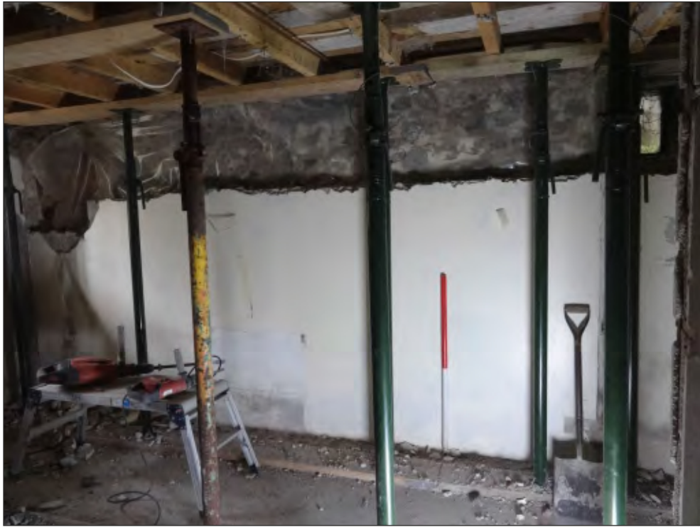
Pl. 1 Demolition works in the inner room, showing the tanking of the north wall behind the modern walling. 1m scale. Looking southeast.
