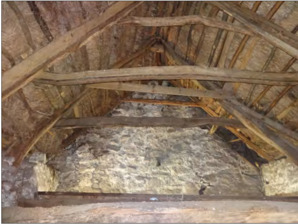
Pl. 21 View of the early 14th-century truss at the north end of the shippon.
