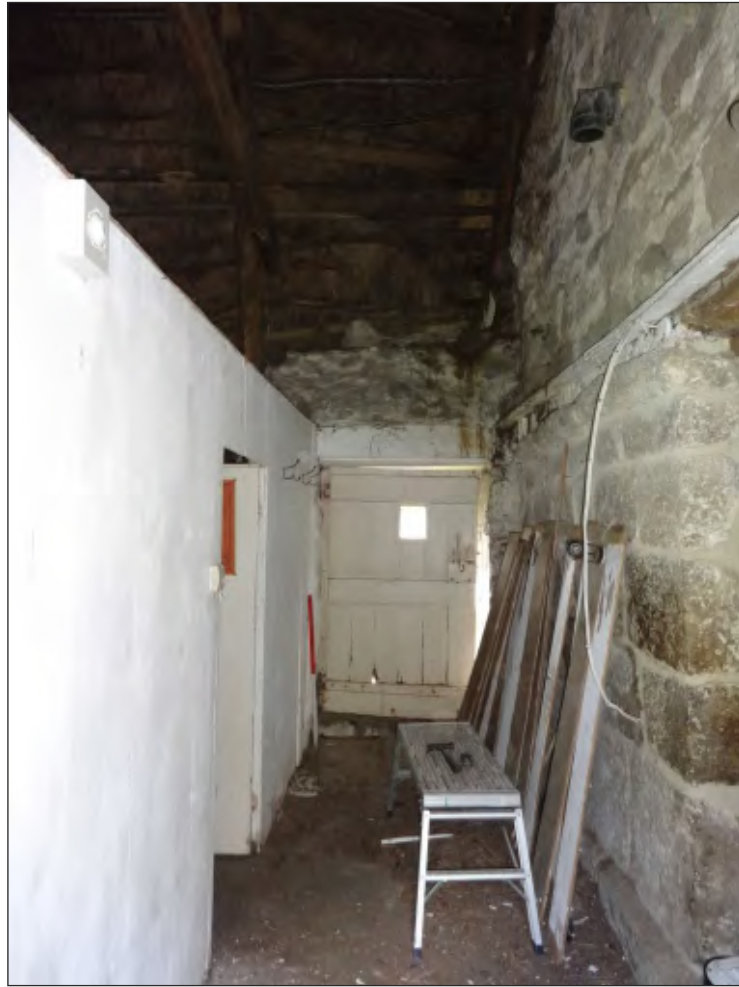
Pl. 9 View of the cross passage prior to the demolition of the modern screens. 1m scale. Looking west.
