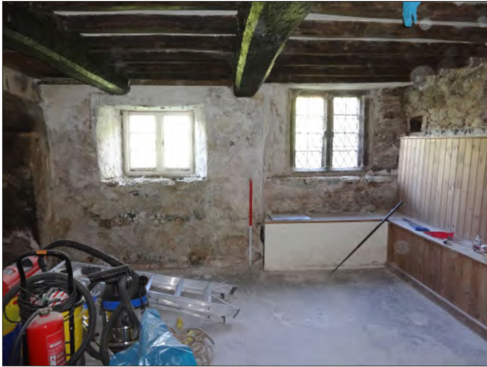
Pl. 5 View of the hall following the removal of modern finishes. 1m scale. Looking west.
