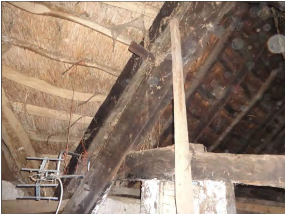
Pl. 22 Detail of the additional rafter added over the eastern principal of the earlier 17th-century truss (looking south-east), showing smoke blackening to both timbers.
