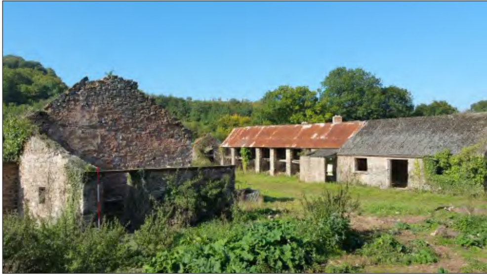
Pl. 21 Close-up showing C19th outbuildings attached to east end off threshing barn. 2m scale. Looking northwest.
