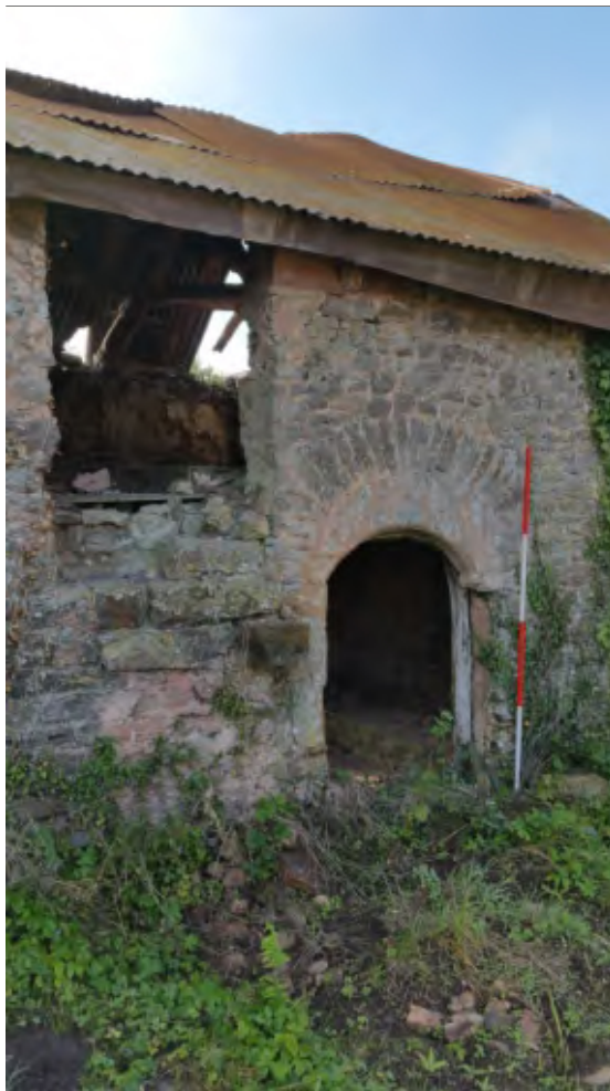
Pl. 10 Close-up of C15th chapel entrance and C18th first floor stair and doorway. 2m scale. Looking southwest.
