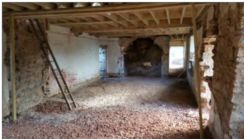
Pl. 4 General view towards room G03 after removal of solid cross walls showing fireplace with sgraffito decoration. 2m scale. Looking east.
