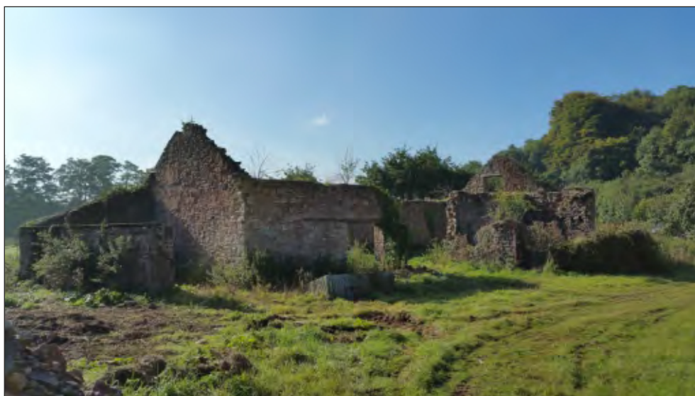
Pl. 19 General view of threshing barn and horse engine house. 2m scale. Looking southwest.
