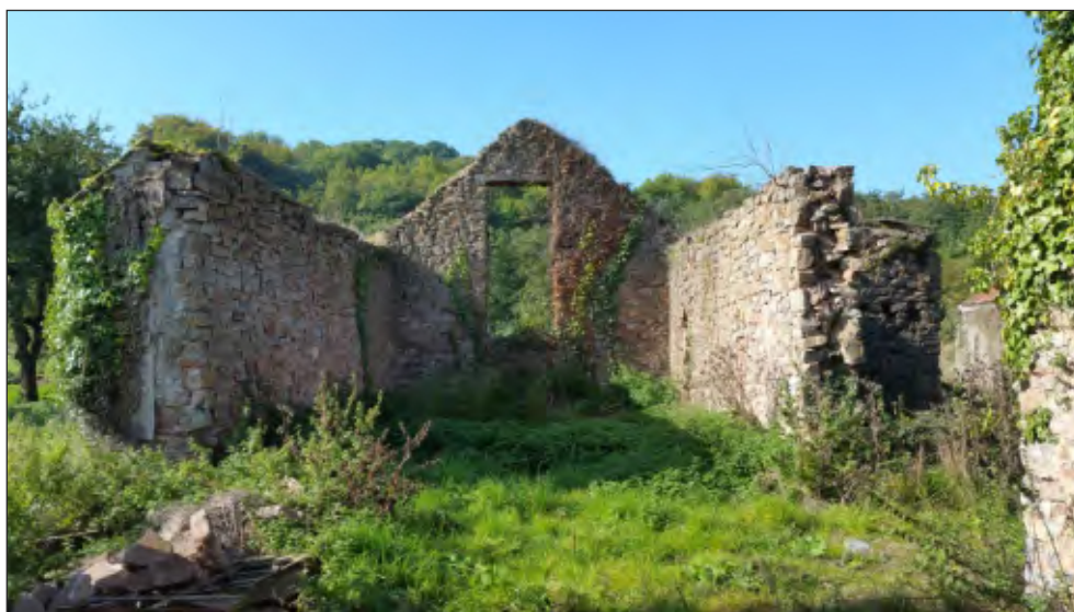
Pl. 23 General view of threshing barn interior showing large window in west gable. Looking west.
