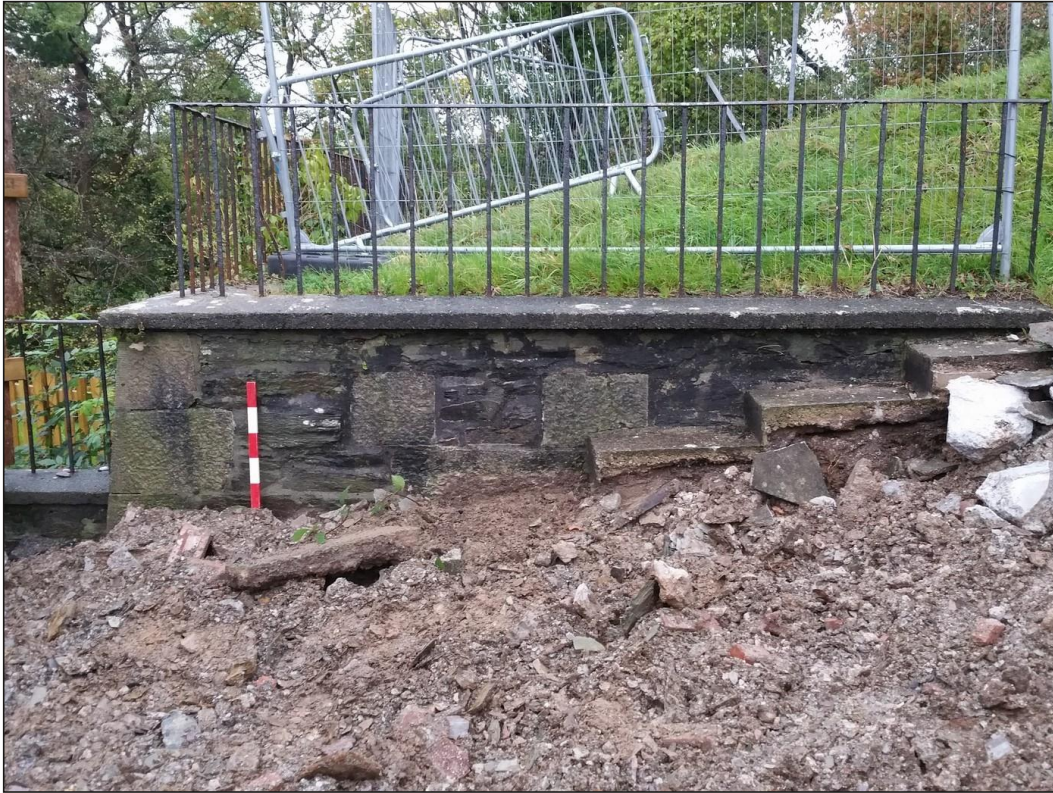
Fig. 6 View of the flank wall with granite detail (centre) indicating location of gun opening, looking north-west (0.5 m scale).
