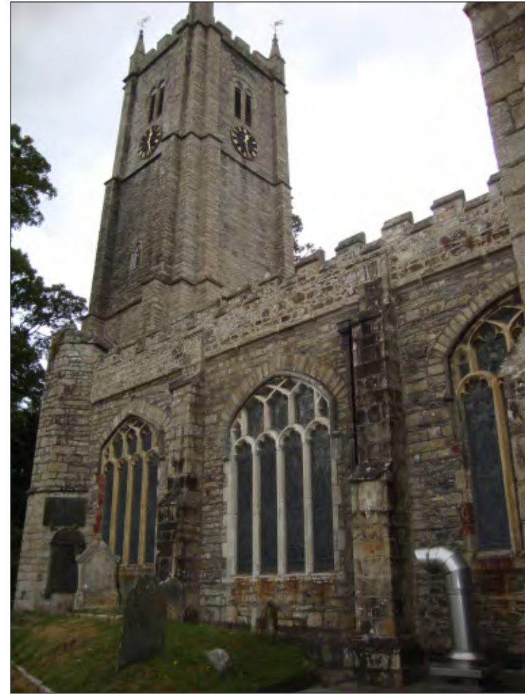
Fig. 5 General view of south aisle wall showing blocked doorway and later enlarged window. Looking northwest.
