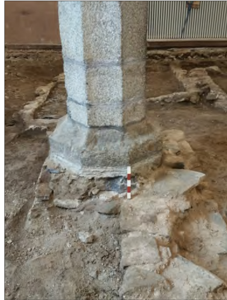
Fig. 26 Close-up showing 12th century wall overlain by early 15th century pier base. 0.25m scale. Looking east.
