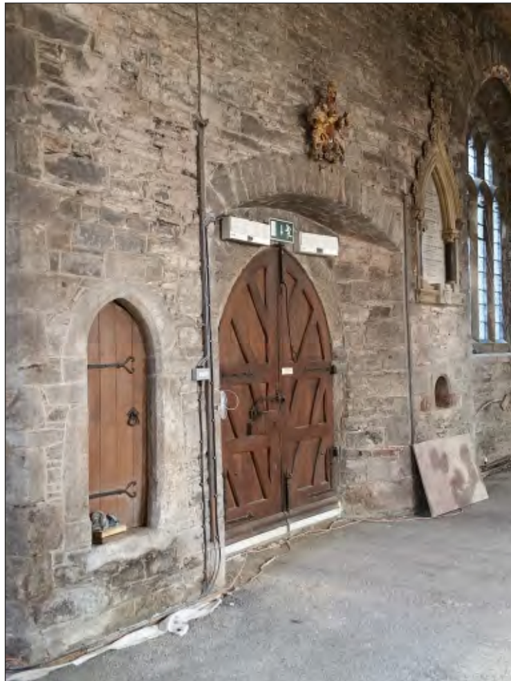
Fig. 6 General view of north doorway (centre) and staircase to porch room (left). Looking northeast.
