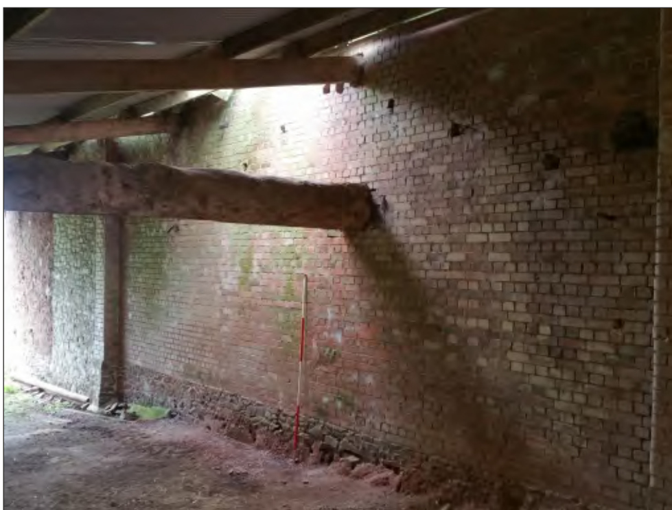
Fig. 32 General view of rear elevation showing earlier roof line. 2m scale. Looking northeast.
