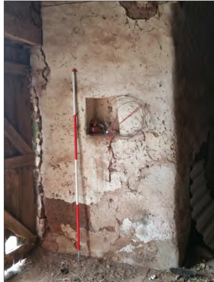
Fig. 40 General view of square recess in internal south elevation of south porch. 2m scale. Looking south.
