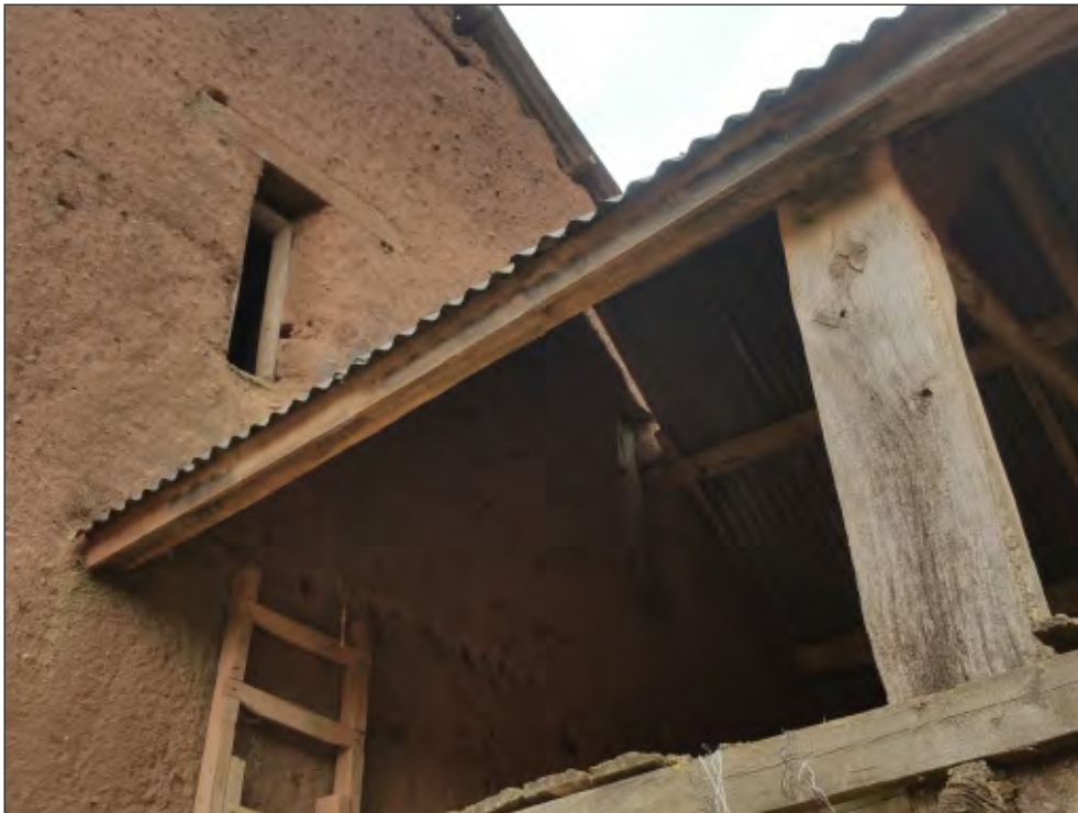
Fig. 36 Close-up of northern elevation showing blocked window and earlier roof line. Looking southwest.
