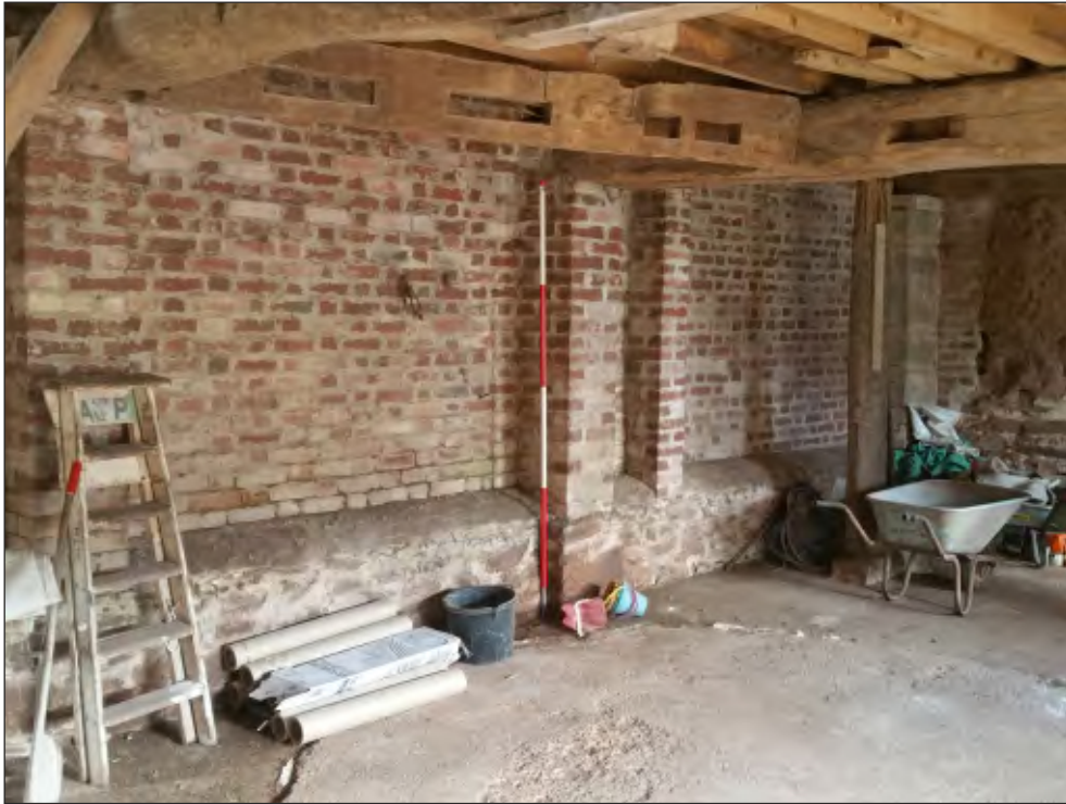
Fig. 14 General view of rear wall showing rebuilt section. 2m scale. Looking northeast.
