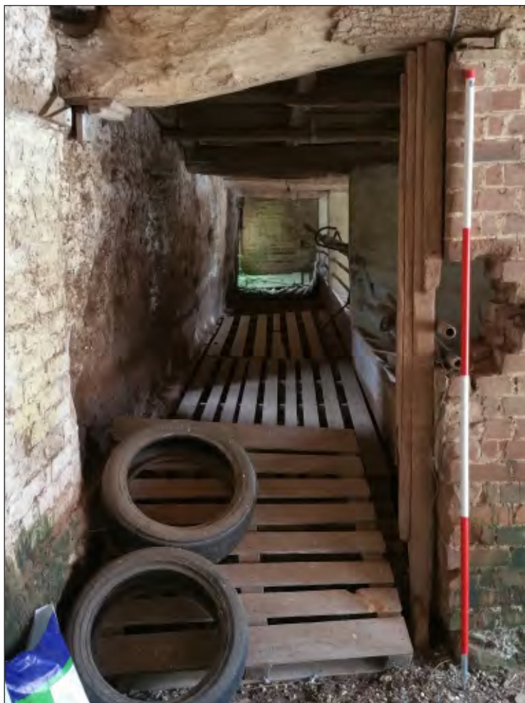
Fig. 19 General view of feeding passage and livestock stalls. 2m scale. Looking east.
