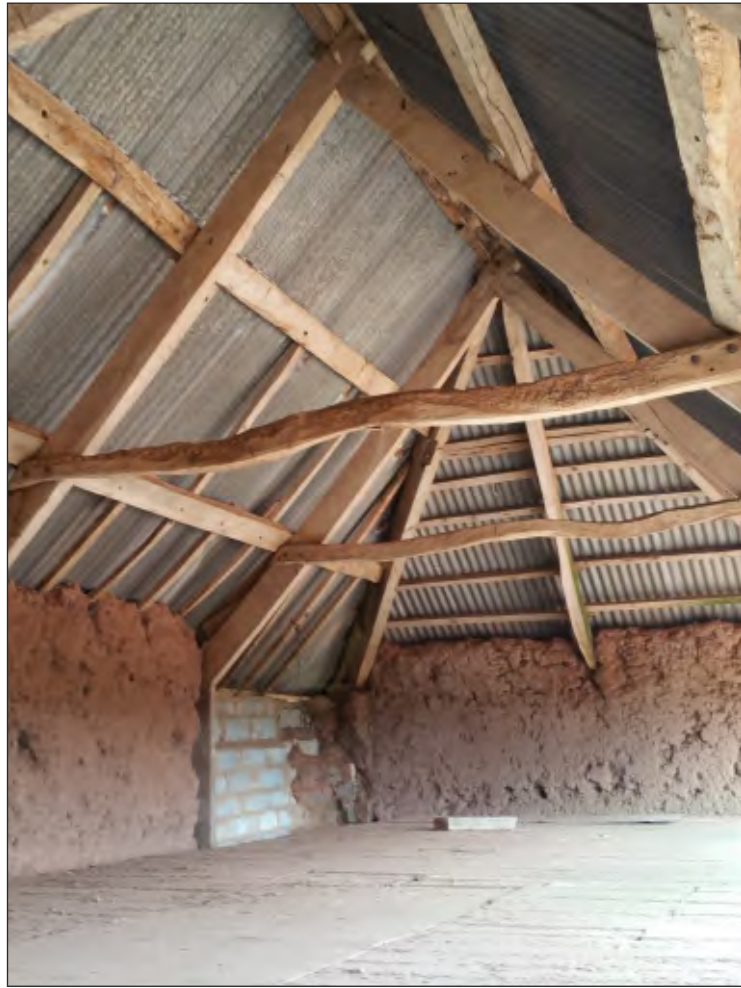
Fig. 47 General view of first floor of linhay showing roof construction. Looking north.
