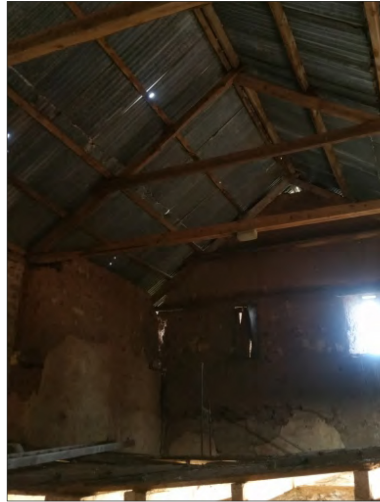
Fig. 44 General view of north elevation of threshing barn showing blocked window. Looking north.
