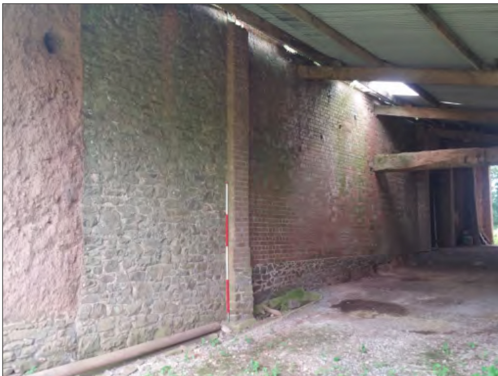
Fig. 31 General view of rear elevation showing blocked northern doorway (left) and rebuilt section (right). 2m scale. Looking southeast.
