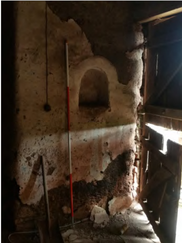
Fig. 39 General view of recess in internal north elevation of south porch with curved head. 2m scale. Looking northeast.
