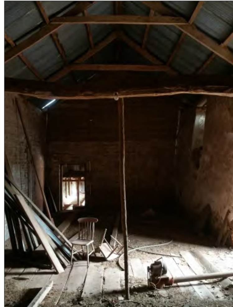
Fig. 38 General view of upper threshing barn interior showing brick partition and doorway to lower threshing barn. 2m scales. Looking north.
