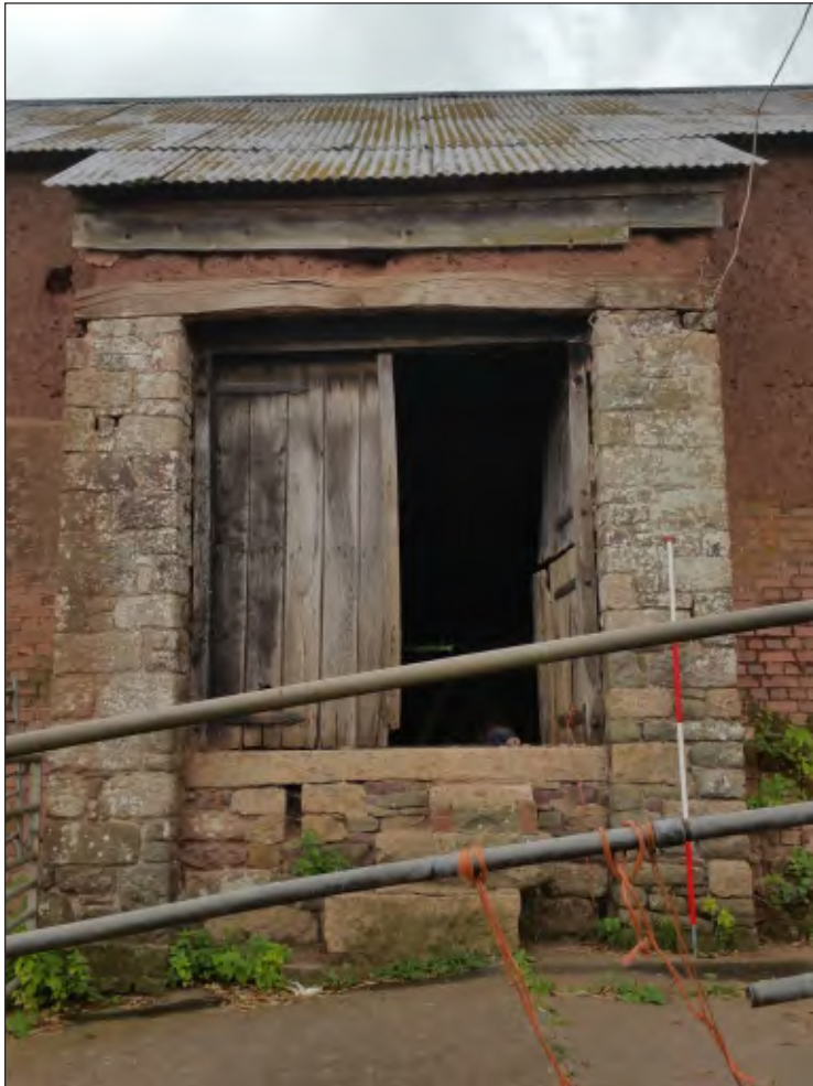
Fig. 29 General view of east doorway (farmyard side) with ventilation shafts. 2m scale. Looking west.
