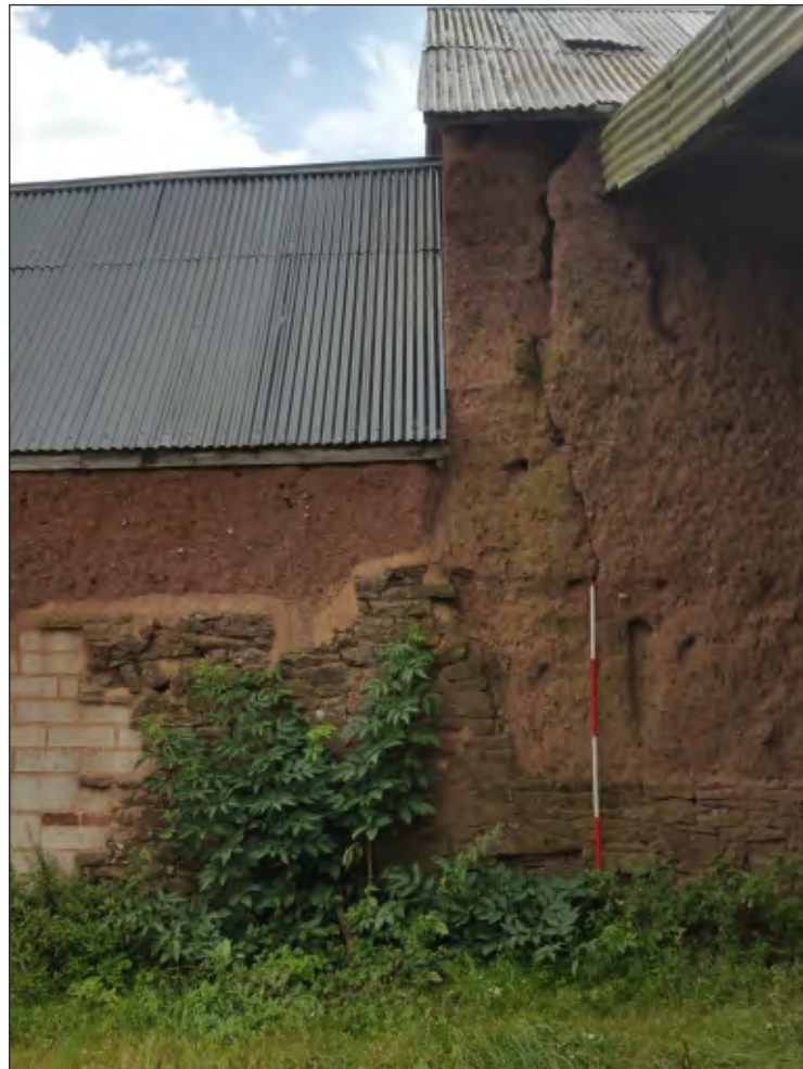
Fig. 46 Close-up of junction between threshing barn and linhay showing difference in height of stone foundations. 2m scale. Looking east.
