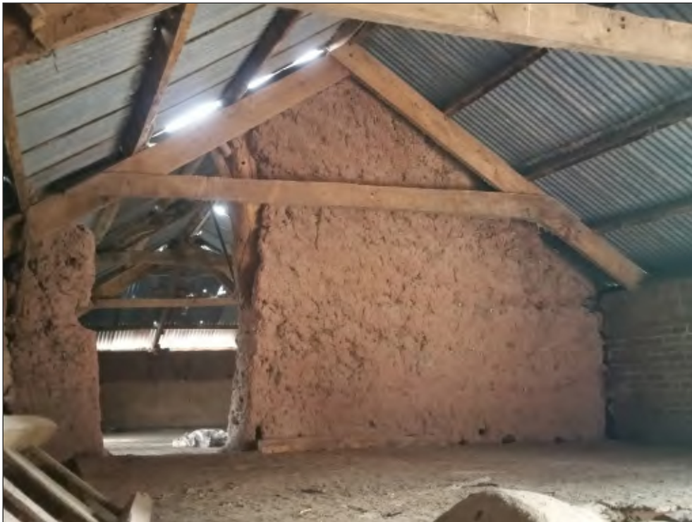
Fig. 24 General view of cob partition running to the apex with later opening. Looking east.
