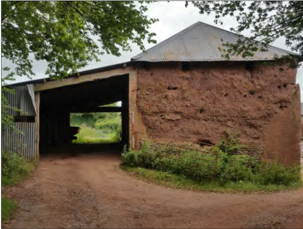
Fig. 35 General view of southern elevation showing owl holes. 2m scales. Looking north.
