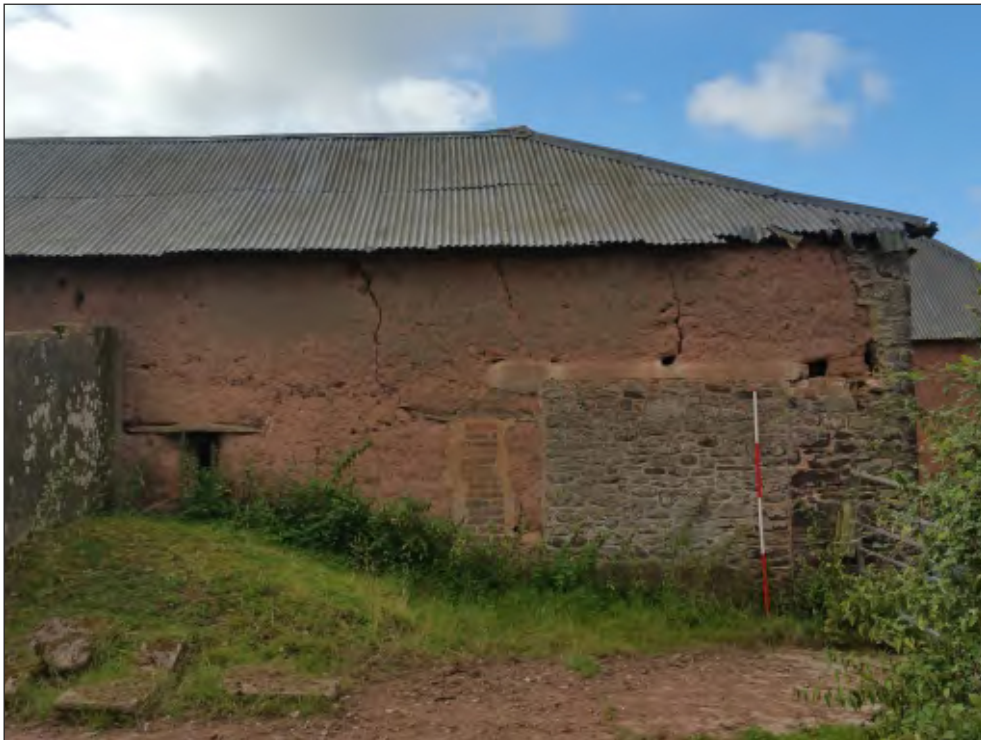
Fig. 22 General view of rear elevation showing blocked openings. 2m scale. Looking south.
