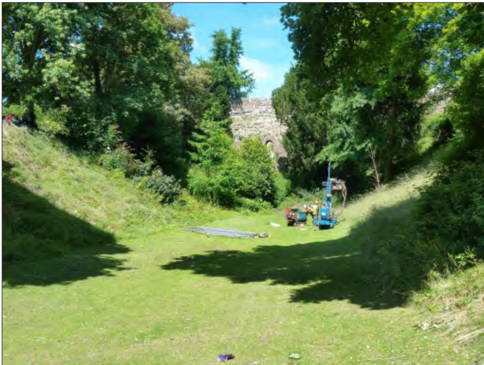
Pl. 6 General view of tracked percussive auger rig excavating Borehole 5a. Looking northwest.
