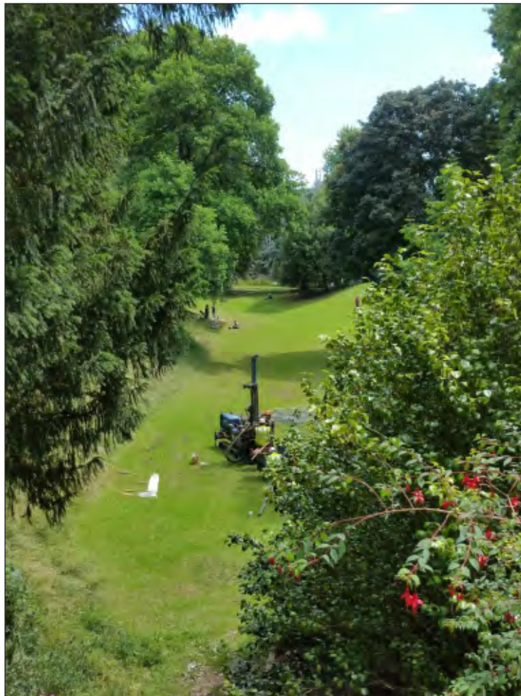
Pl. 8 General view of tracked percussive auger rig excavating Borehole 5b. Looking southeast.
