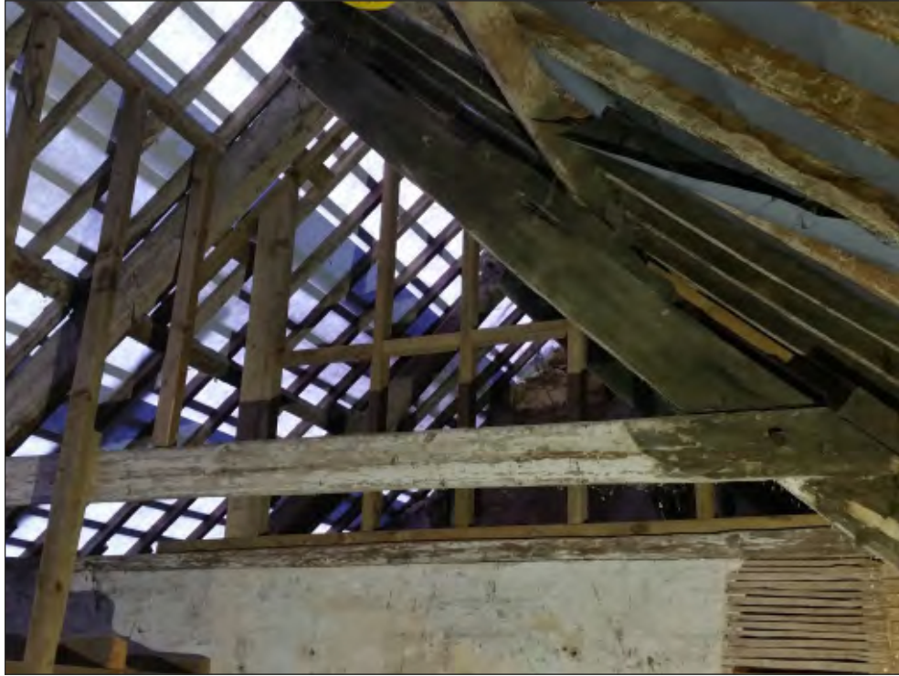
Pl. 33 General view of late 18th - early 19th century roof construction above landing F4. Looking southwest.
