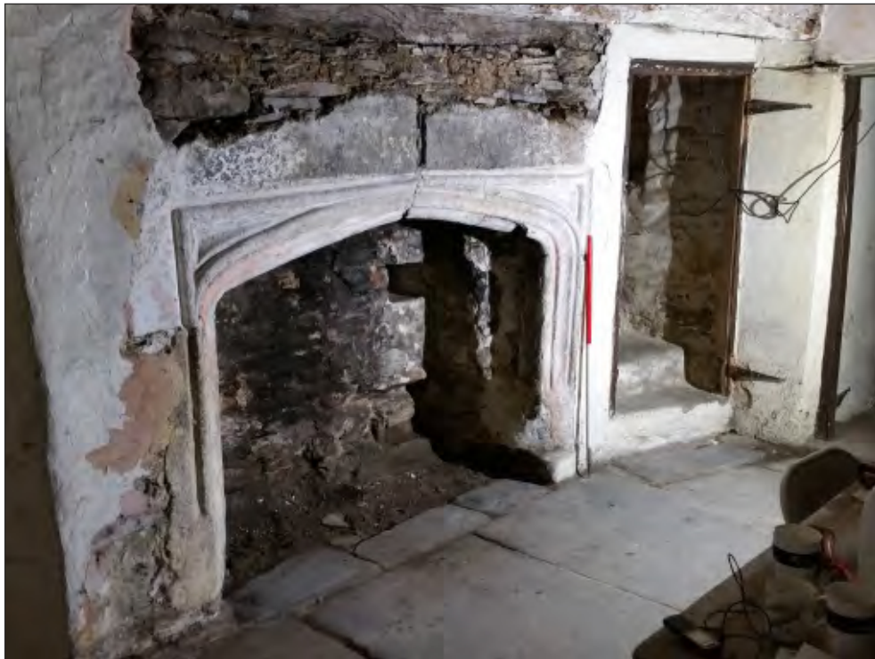
Pl. 14 General view of the 16th- or 17th-century fireplace in room G6 with contemporary stair (right). 1m scale. Looking northwest.
