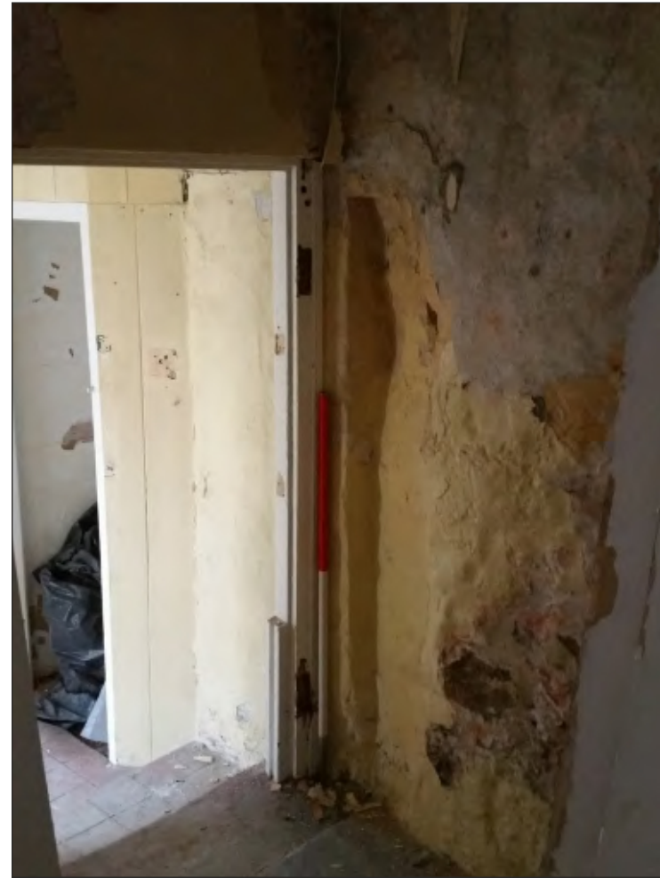
Pl. 20 General view of wall scar between rooms G1 and G2 indicating the possible location of a stair turret. 1m scale. Looking southwest.
