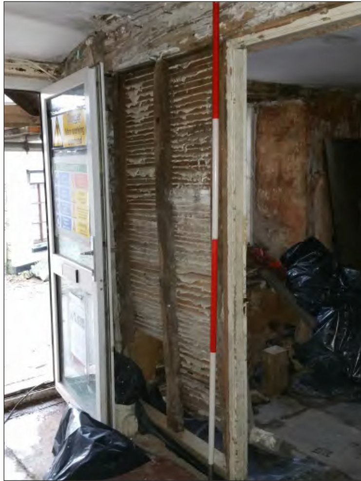
Pl. 7 General view of partition between corridor G3 and room G4 showing late 19th century doorway. 2m scale.
