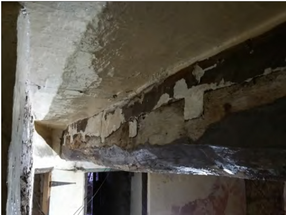
Pl. 16 Close-up of former jetty bresummer beam in room G6 showing infilled joist holes and the raising of the main beam height to insert the later floor above. Looking northeast.
