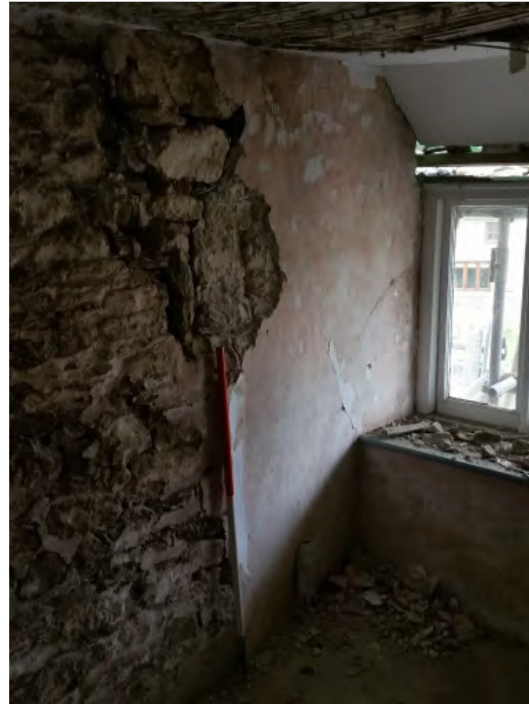
Pl. 30 Close-up of vertical building break showing re-fronting of the western end of Staddons House. 1m scale. Looking southeast.
