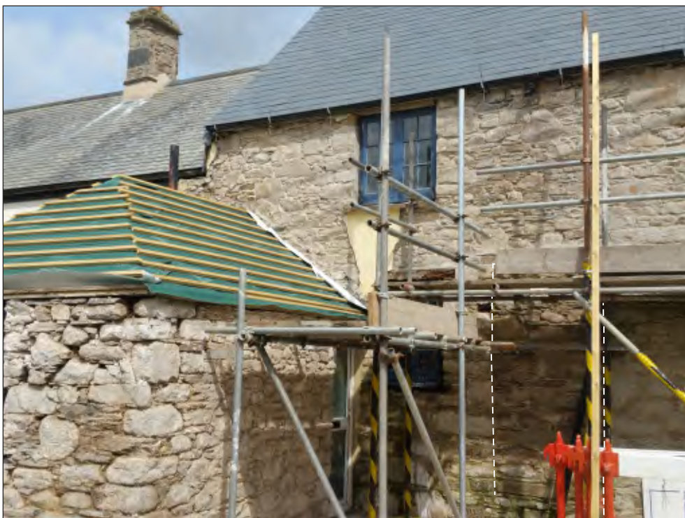
Pl. 2 General view of western end of Staddons after removal of render showing blocked doorway into room G4 (right). Looking northwest.
