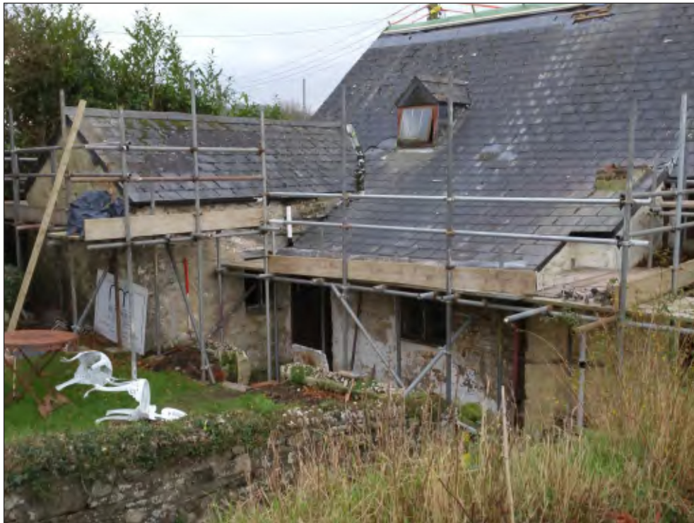
Pl. 4 General view of late 19th century dairy (left) and scullery (center) after removal of render. 1m scale. Looking southeast.
