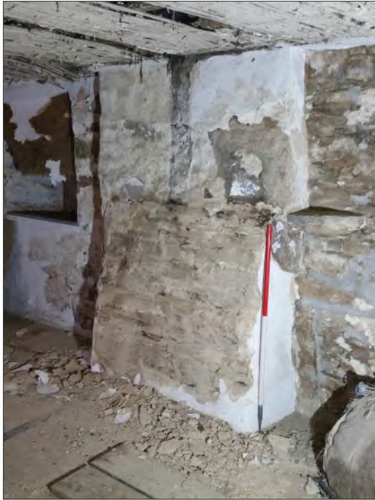
Pl. 29 General view of blocked medieval window (left) and medieval fireplace with later blocking in room F1/3. 1m scale. Looking southwest.
