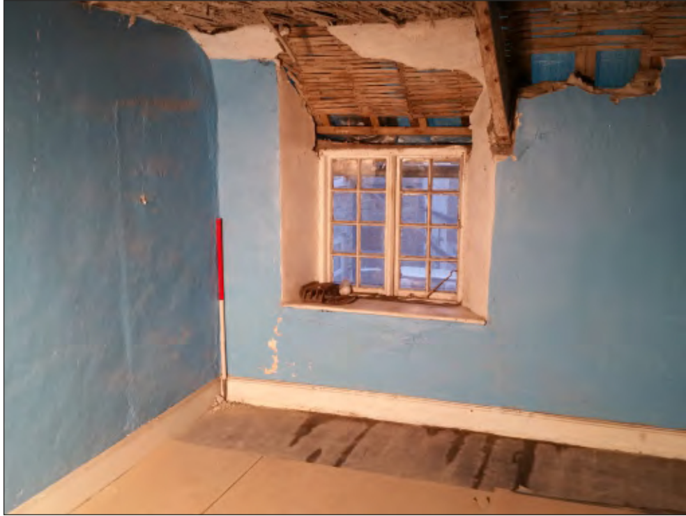
Pl. 25 General view of room F6 showing blocked doorway in eastern partition and window. 1m scale. Looking southeast.
