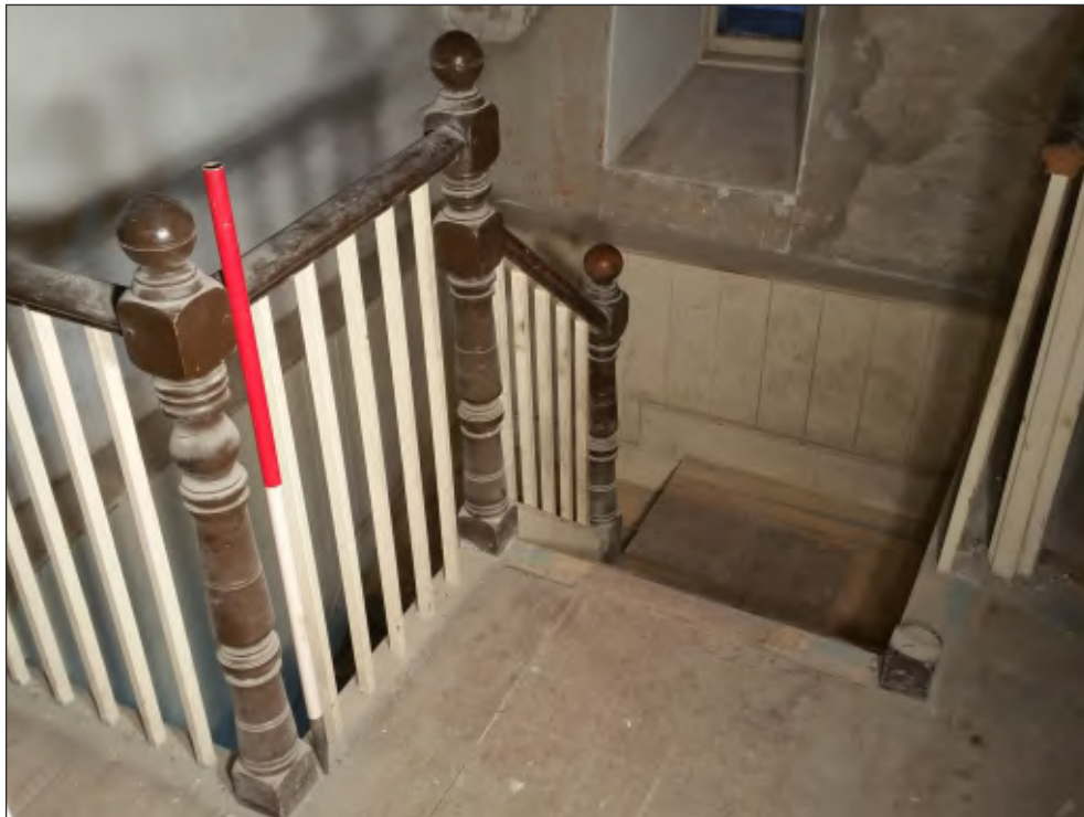
Pl. 22 General view of late 19th century staircase from landing F4. 1m scale. Looking northwest.
