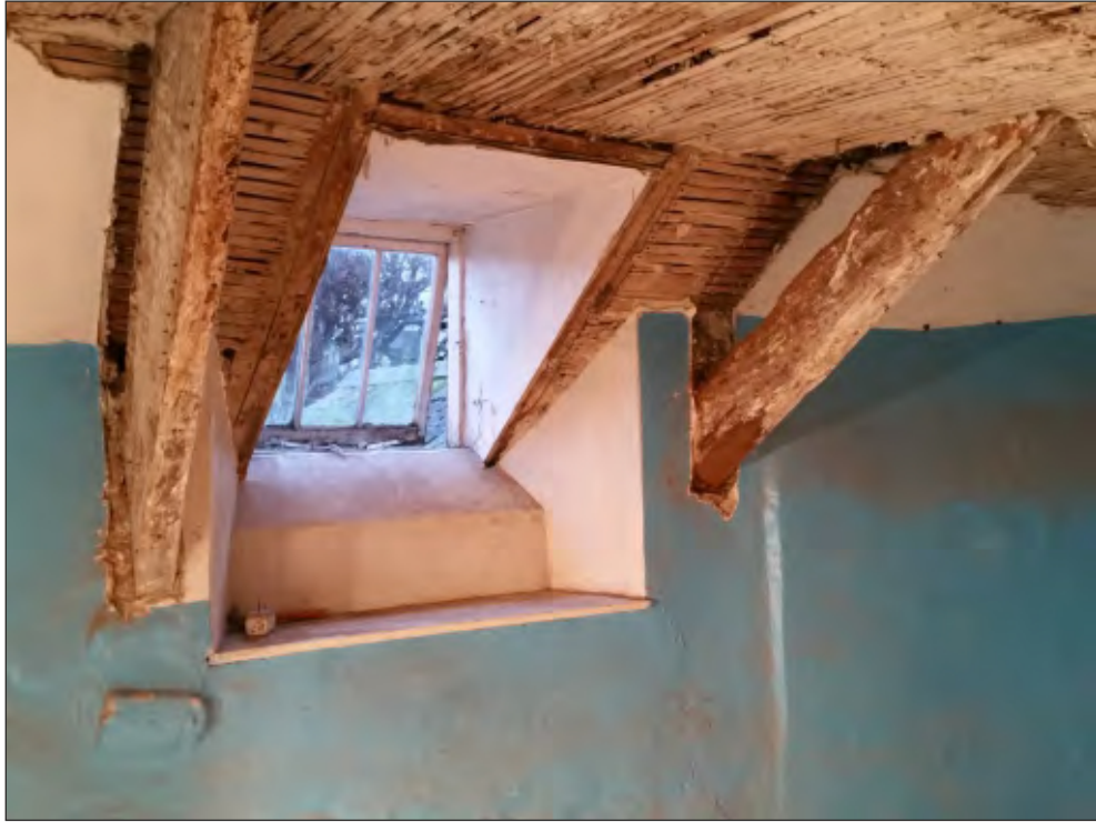
Pl. 27 General view of window in north elevation in room F8. Looking northeast.
