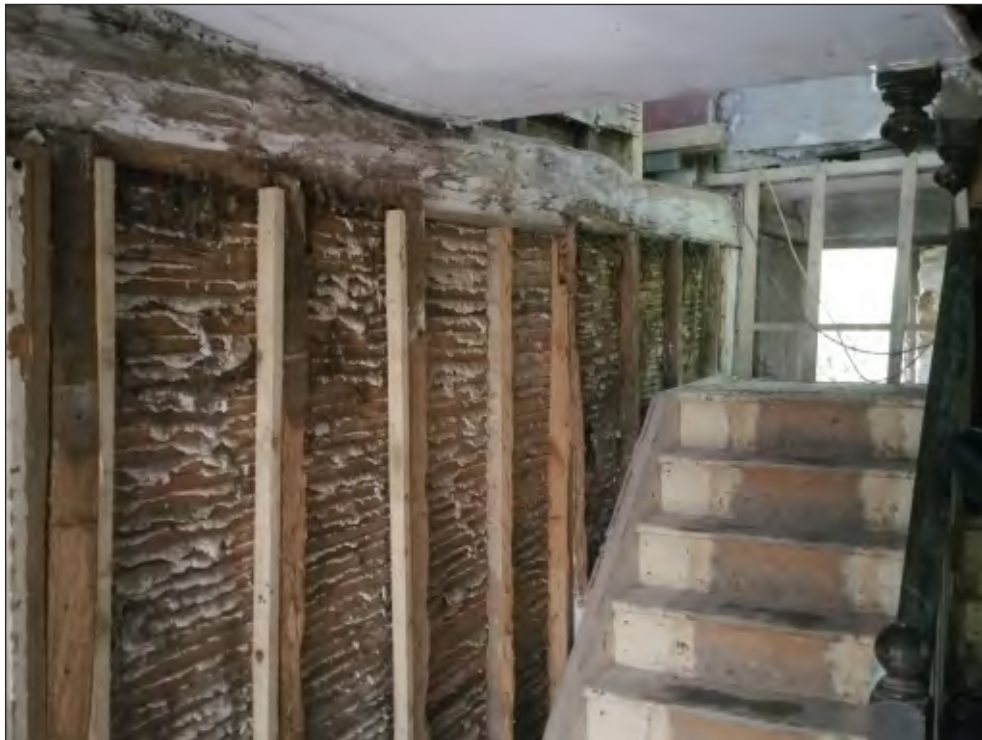
Pl. 8 General view of partition between corridor G3 and room G4 showing blocked doorway in the centre and the random door included within the partition behind the staircase. Looking northwest.
