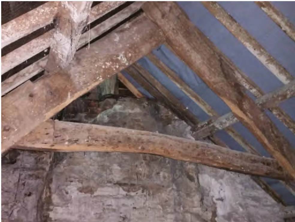
Pl. 34 General view of late 18th - early 19th century roof construction above room F 9. Looking northwest
