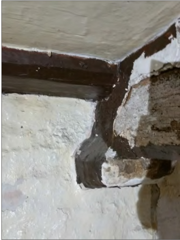
Pl. 17 Close-up of large beam in G6 supported on stone corbel, small beam supported in south wall and additional timber above beam to raise the floor level consistently throughout the first-floor. Looking northeast.
