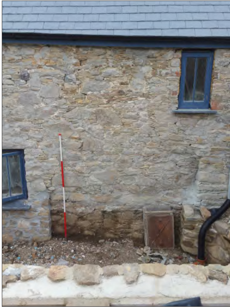
Pl. 5 General view of blocked opening at rear of room G2 after removal of render showing protruding masonry to the left and right defining the original opening. 2m scale. Looking south.
