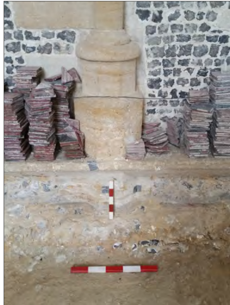
Pl. 8 Close-up showing flint and clay foundations (1016) of west elevation south transept. 0.25m and 0.5m scales. Looking west.
