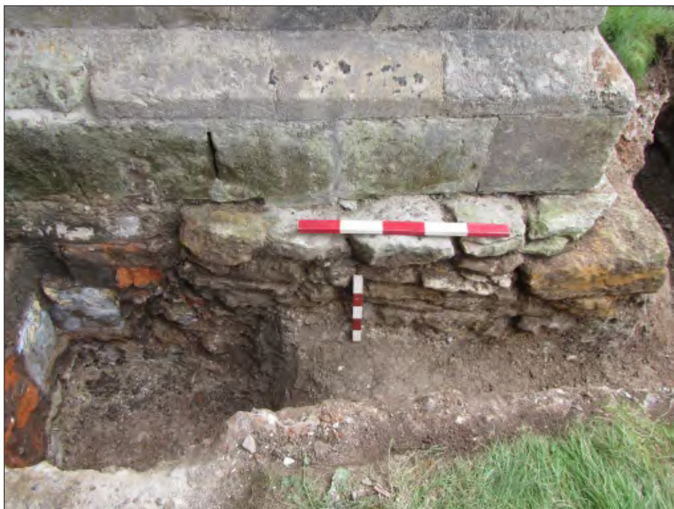
Pl. 11 Close-up of medieval foundation of buttress on south elevation. 0.25m and 0.5m scales. Looking east.
