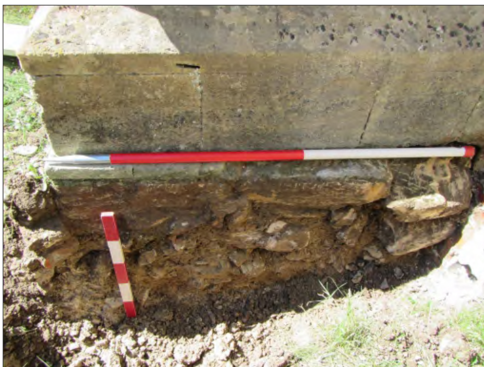
Pl. 12 Close-up of medieval foundation of buttress on south elevation. 0.5m and 1m scales. Looking west.
