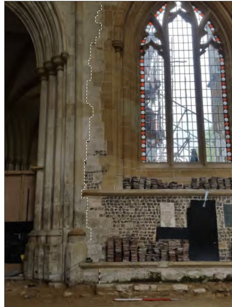
Pl. 6 General view of building break in eastern elevation of south transept (white) and coinciding with change in foundations. 0.25m and 1m scales. Looking east.
