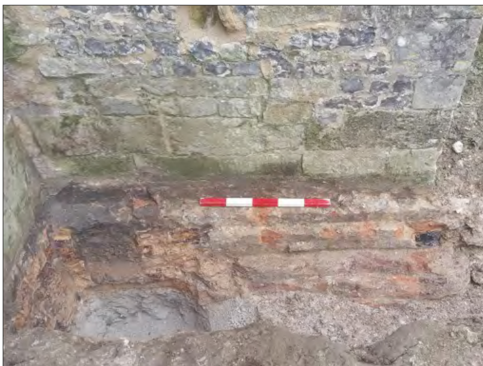
Pl. 22 Close-up of post-medieval brick underpinning of buttress on north elevation. 1m scale. Looking west.
