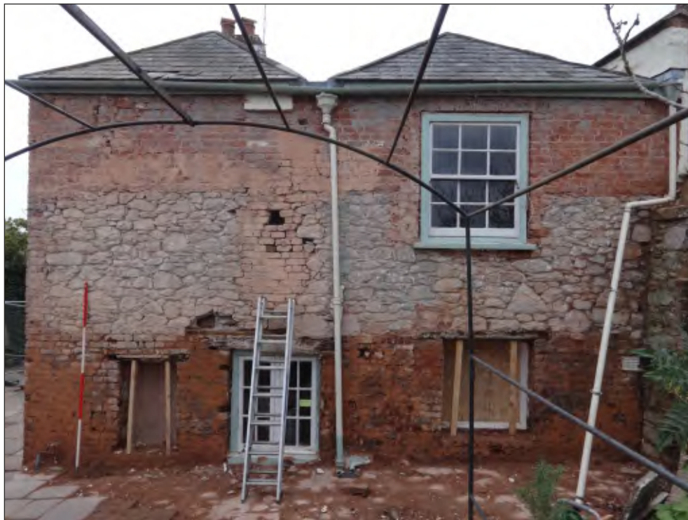
Pl. 8 General view of rear building showing successive raising of rear elevation, the remains of a chimney stack and 18th and 19th century alterations to the window openings. 2m scale. Looking northwest.
