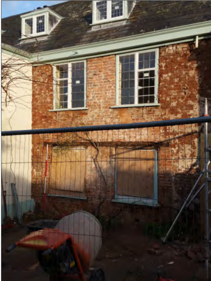
Pl. 3 General view of main house showing early 18th century alterations to the window openings. 2m scale. Looking northwest.
