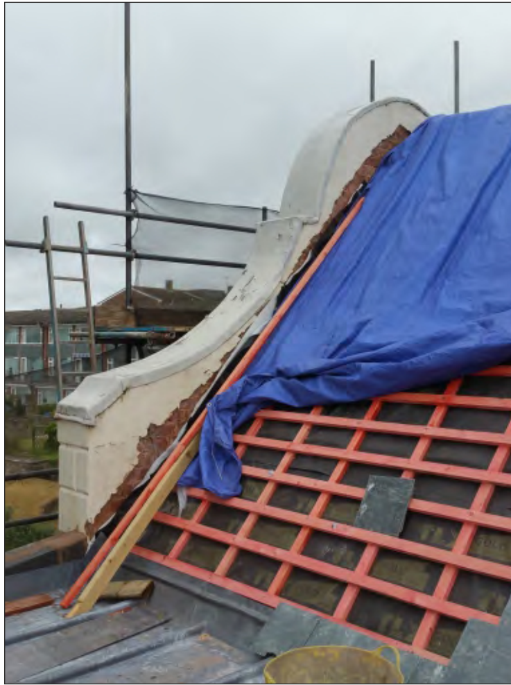
Pl. 35 Close-up of rear of 'Dutch' gable showing substantial modern rebuilding. Looking northwest.
