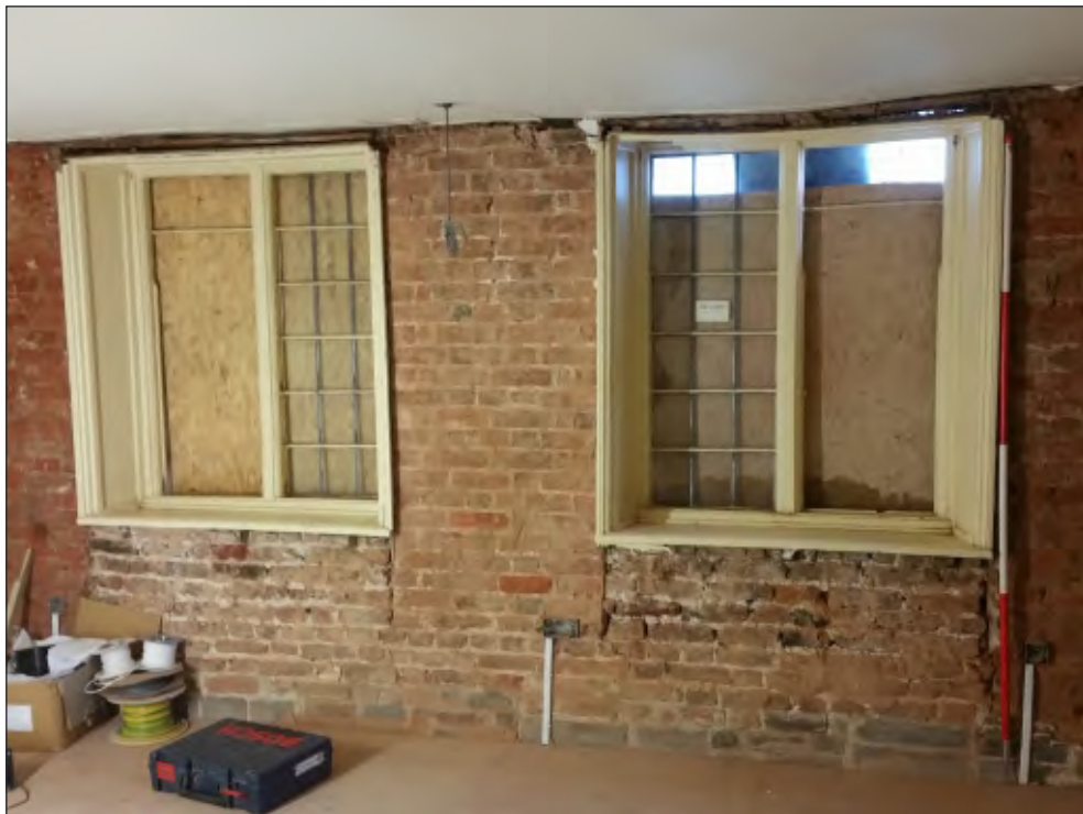
Pl. 32 General view of south elevation first-floor room F04 showing early 18th century alterations to the window openings and blocked-up window seats underneath. 2m scale. Looking southeast.
