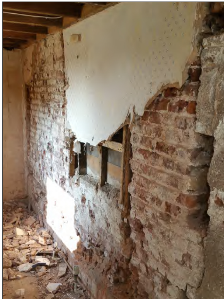
Plate 28 General view of main house elevation showing early window arrangement with early 18th century alteration of the original opening and modern blocking. 2m scale. Looking southwest.
