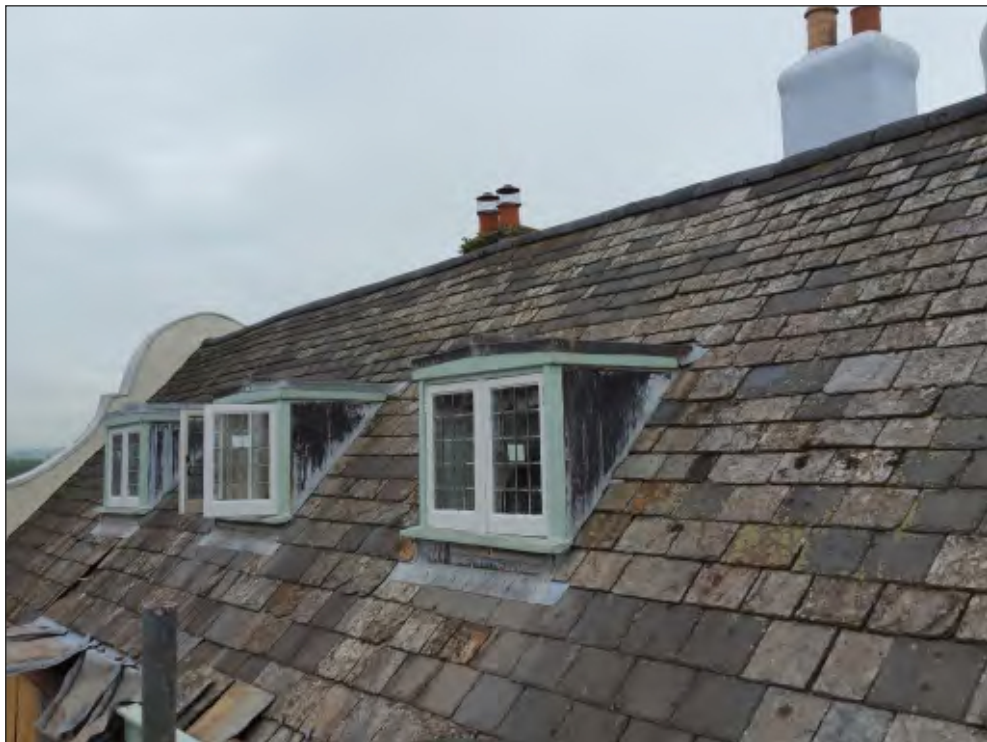
Pl. 36 General view of roof showing dormer windows and decreasing size of slates. Looking northwest.
