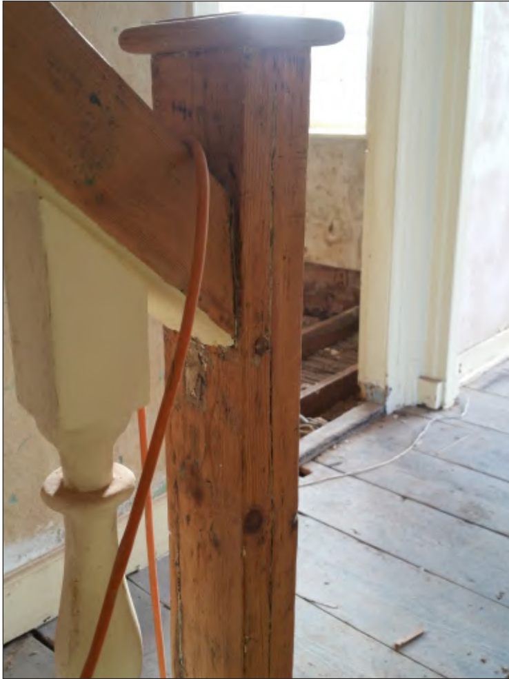
Pl. 25 Close-up of stair construction showing earlier socket and peg hole. Looking southeast.
