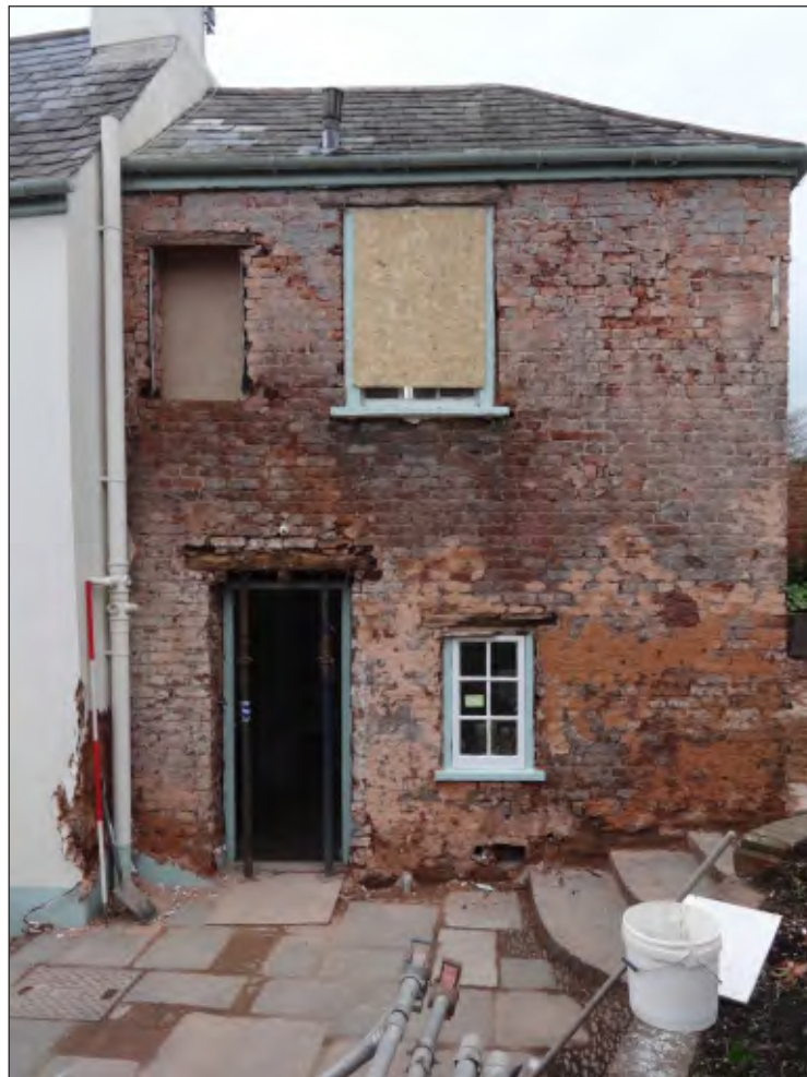
Pl. 6 General view of rear building after removal of render showing early sloping roof line and 18th-20th century alterations to the window openings and doorways. 2m scale. Looking north.
