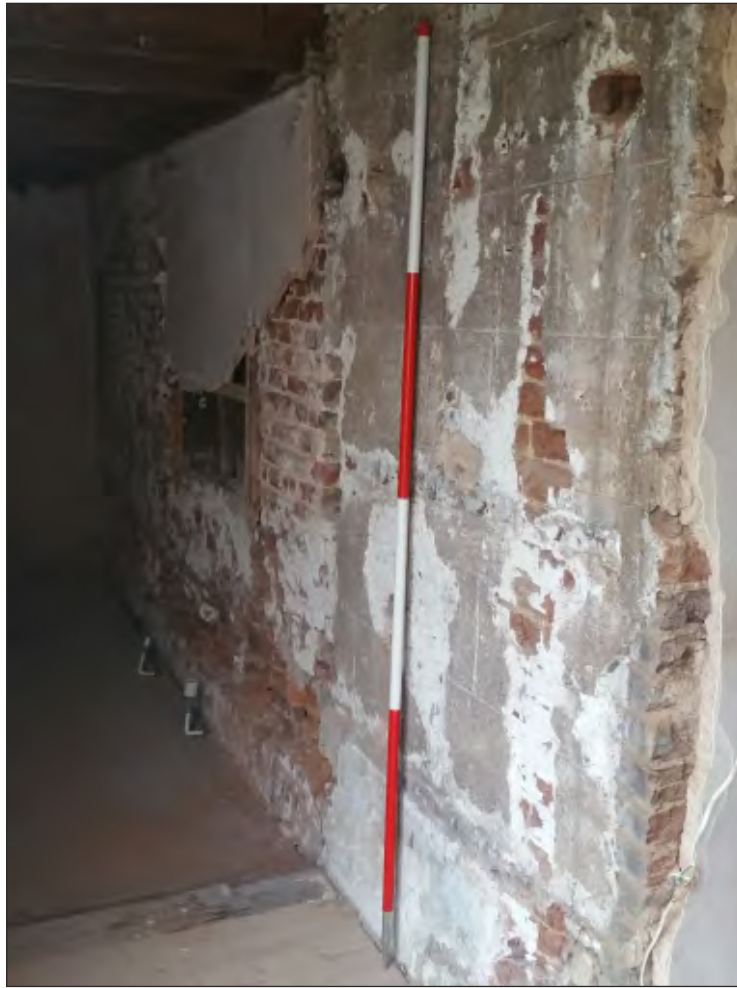
Pl. 29 Small area of surviving 19th century external render with incised ashlar lines. 2m scale. Looking northwest.
