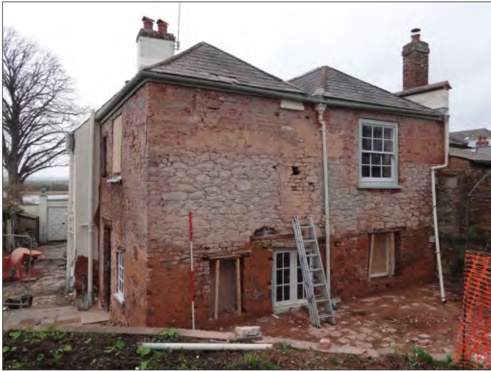
Pl. 7 General view of rear building showing successive raising of rear elevation, the remains of a chimney stack and 18th and 19th century alterations to the window openings. 2m scale. Looking northwest.
