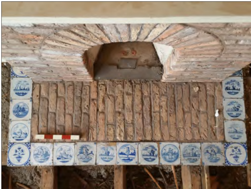
Pl. 30 Close-up of Delft tiles on modern hearth surround first-floor room F02. 0.25m scale. Looking northwest.
