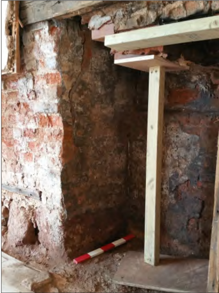
Pl. 13 Close-up of western jamb of fireplace showing black-and-white chequerboard painted plaster decoration. 0.5m scale. Looking northwest.
