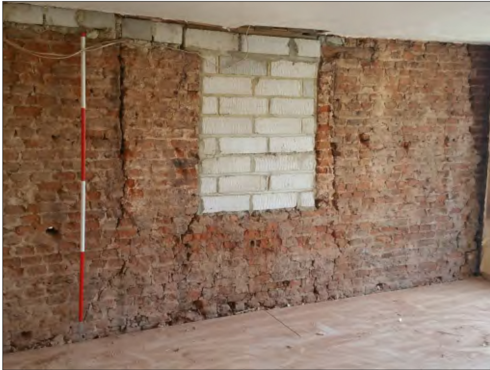
Plate 27 General view of south elevation first-floor room F02 showing early window arrangement with early 18th century alteration of the original opening and modern blocking. 2m scale. Looking southwest.
