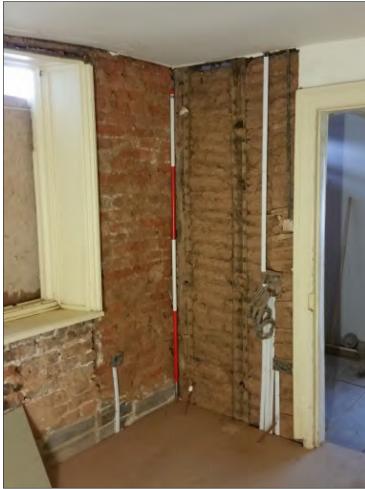
Pl. 31 General view of primary cob partition in first-floor room F04. 2m scale. Looking southwest.
