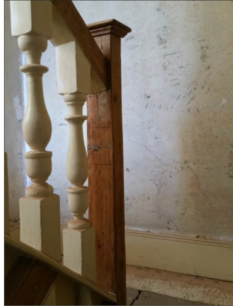
Pl. 26 Close-up of stair construction showing not only the earlier socket and peg hole, but also the inscribed carpenter's marks denoting the intended junction with the lower bannister. Looking southeast.
