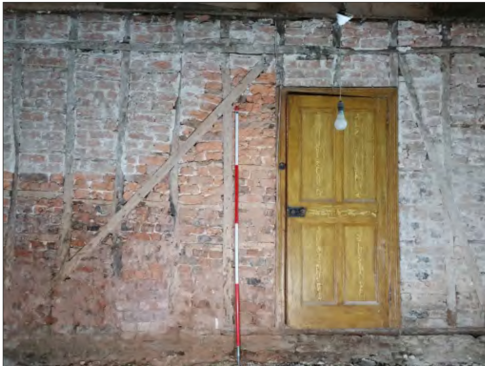
Pl. 6 General view of east elevation ground-floor room G02 showing early 18 th century partition with later brick infill and doorway. 2m scale. Looking east.
