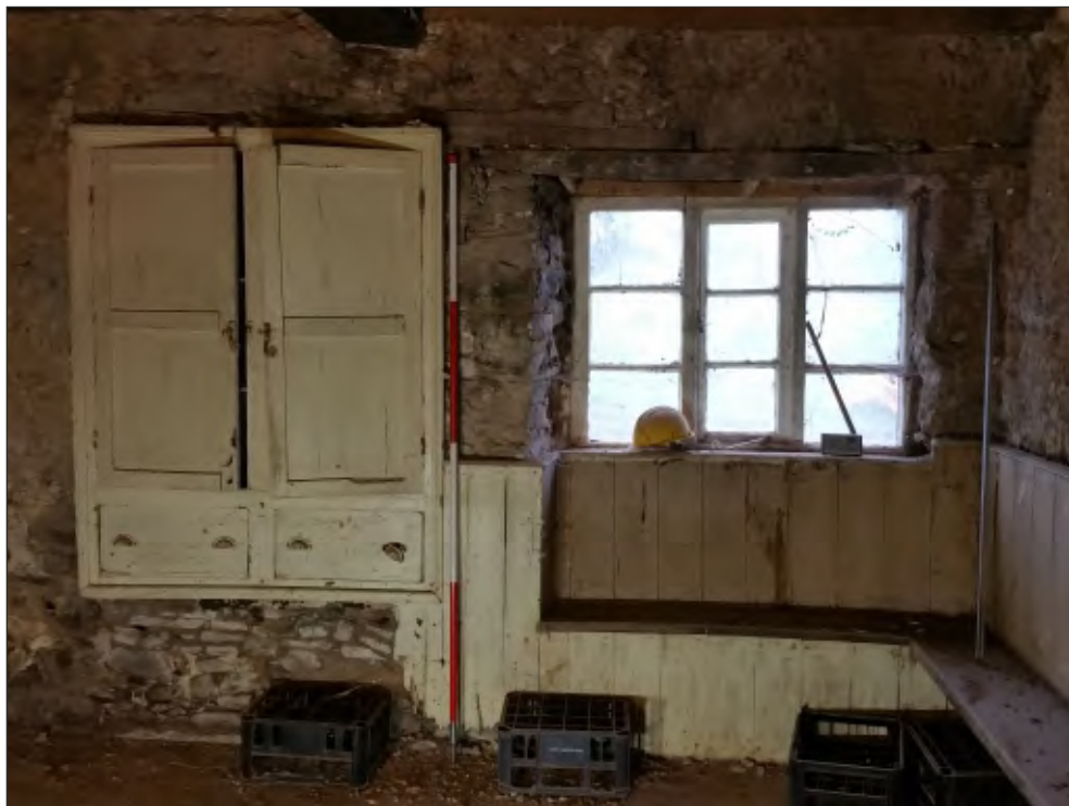
Pl. 14 General view of east elevation ground-floor room G06 showing cupboard inserted into blocked window, with current window inserted to right of blocking. 2m scale. Looking east.
