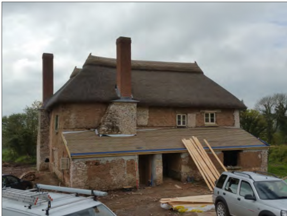
Pl. 4 General view of north elevation showing original chimneystack and early 19th century outshuts. 2m scale. Looking southwest.
