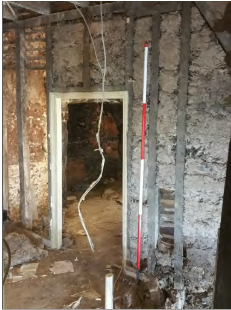
Pl. 11 General view of west elevation ground-floor room G06 showing doorway in cob-infilled partition with corridor G04. 2m scale. Looking southwest.
