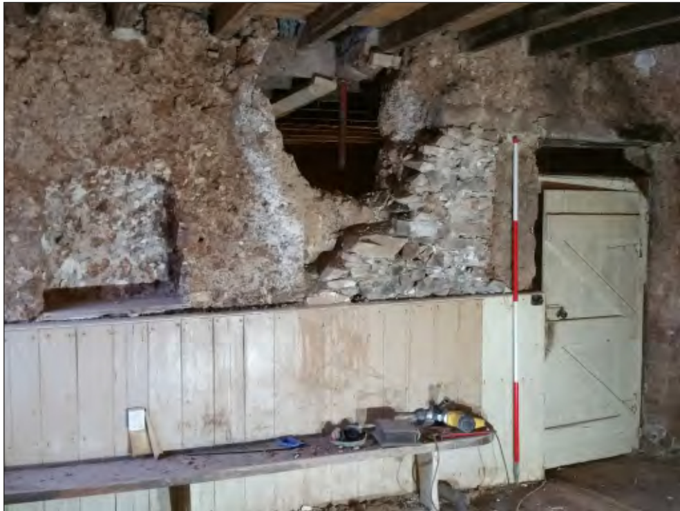
Pl. 13 General view of south elevation ground-floor room G06 showing doorway to room G03, infilled cupboard and later cupboard. 2m scale. Looking south.
