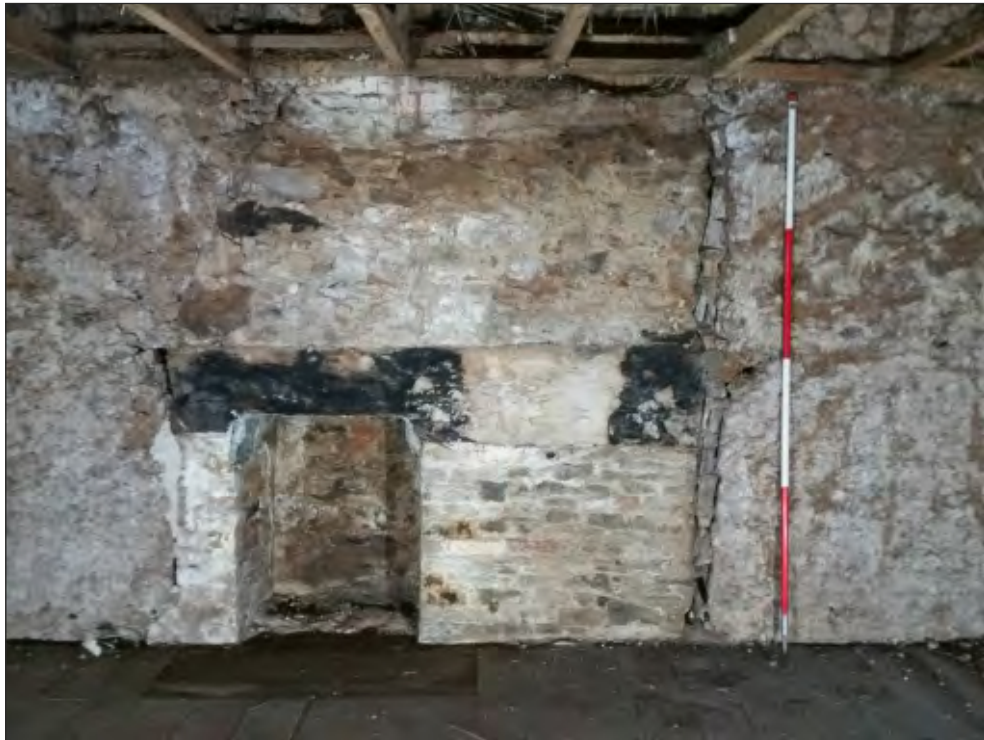
Pl. 19 General view of west elevation first-floor room F02 showing brickwork of small inserted fireplace. 2m scale. Looking west.
