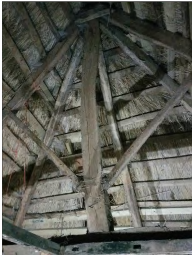
Pl. 24 General view of hip roof arrangement showing reused wall plate timber. Looking east.
