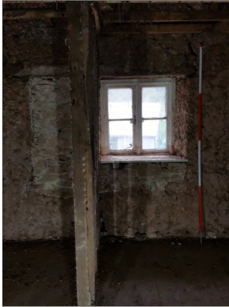
Pl. 21 General view of north elevation first-floor corridor F04 showing window insert through blocking contemporary with late 19th century partition. 2m scale. Looking north.
