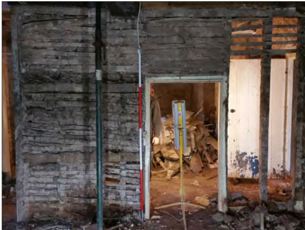
Pl. 12 General view of west elevation ground-floor room G06 showing doorway in cob-infilled partition with corridor G04. 2m scale. Looking west.
