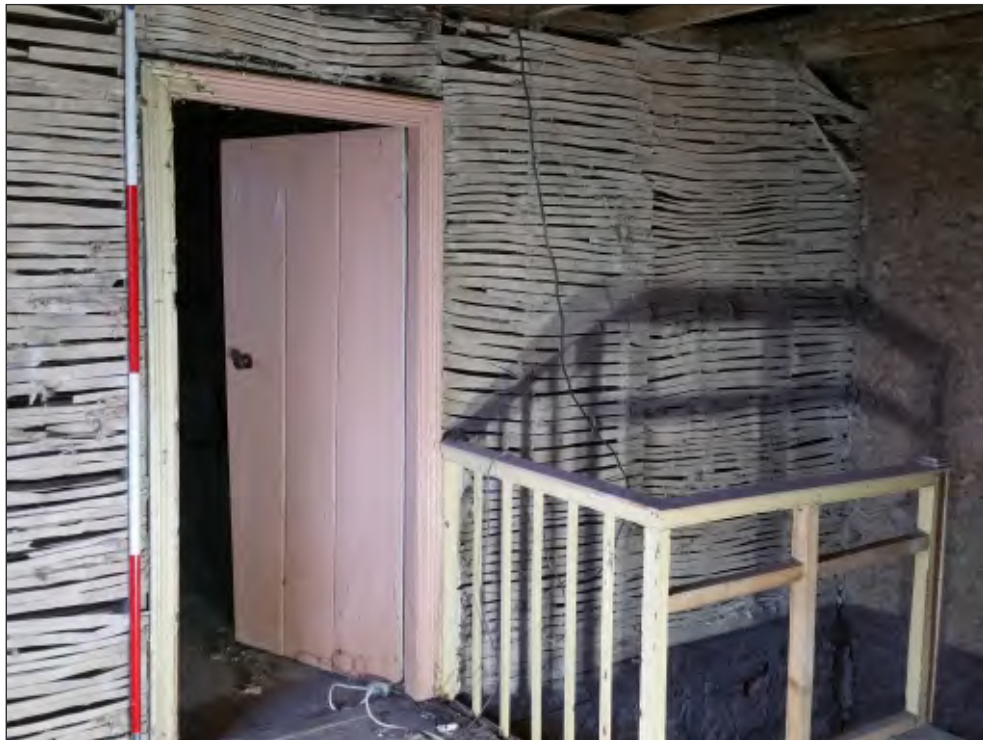
Pl. 18 General view of west elevation landing F01 showing doorway in partition. 2m scale. Looking northwest.
