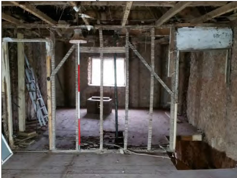
Pl. 22 General view of east elevation first-floor corridor F04. 2m scale. Looking east.
