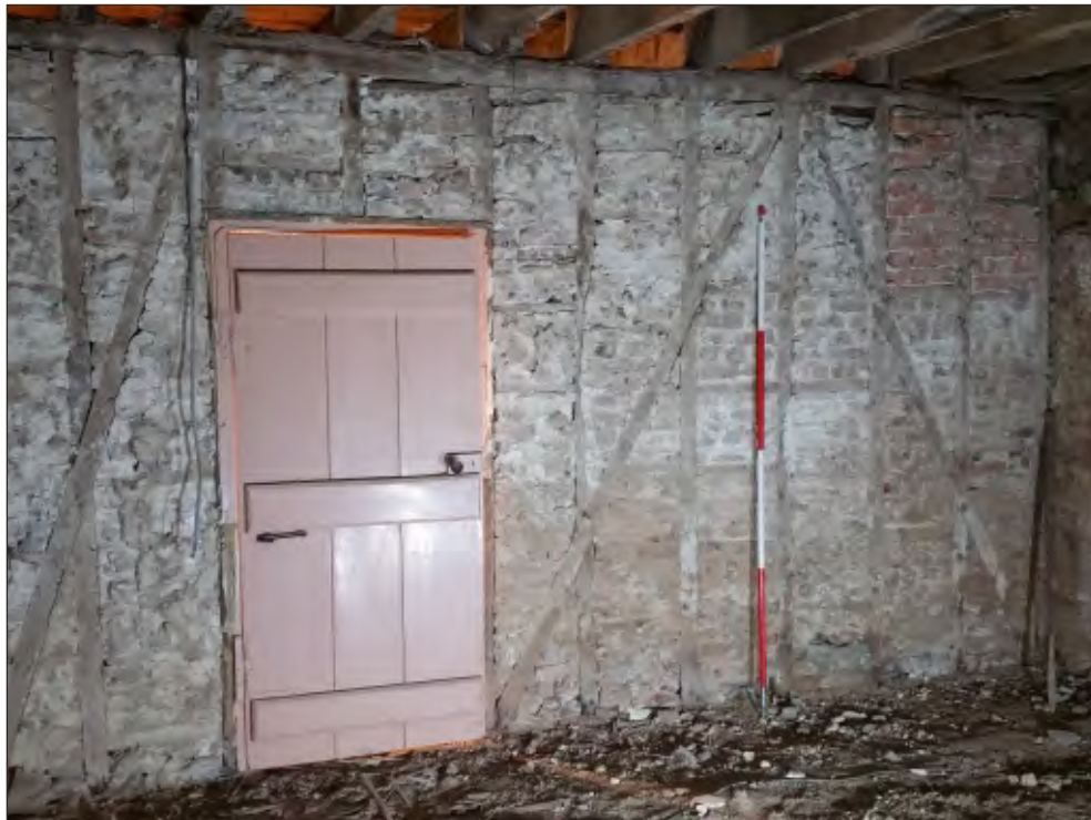
Pl. 8 General view of west elevation room G03 showing early 18 th century partition and doorway with later brick infill. 2m scale. Looking west.
