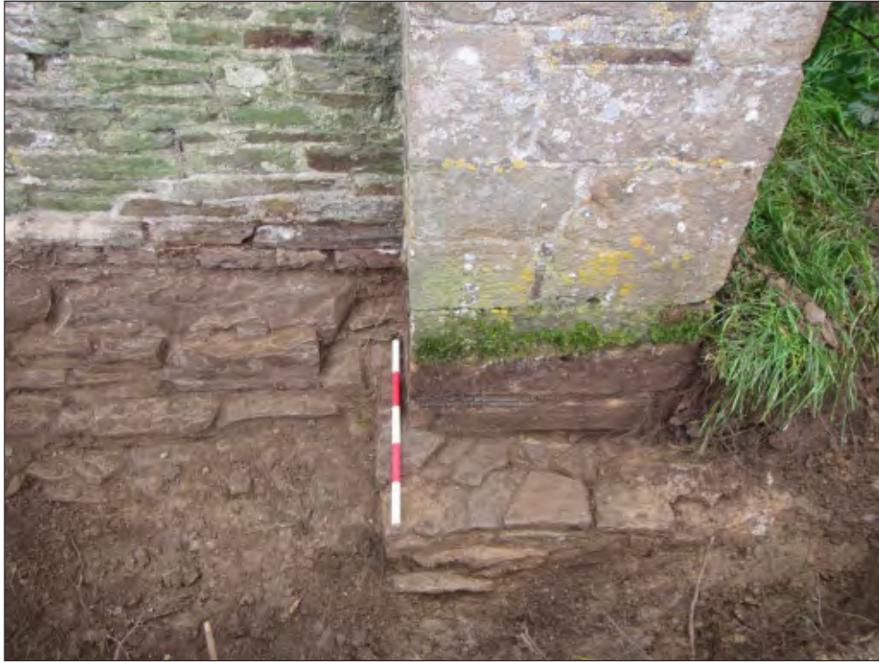
Pl. 10 General view of foundation of north wall and buttress. 0.5m scale. Looking south.
