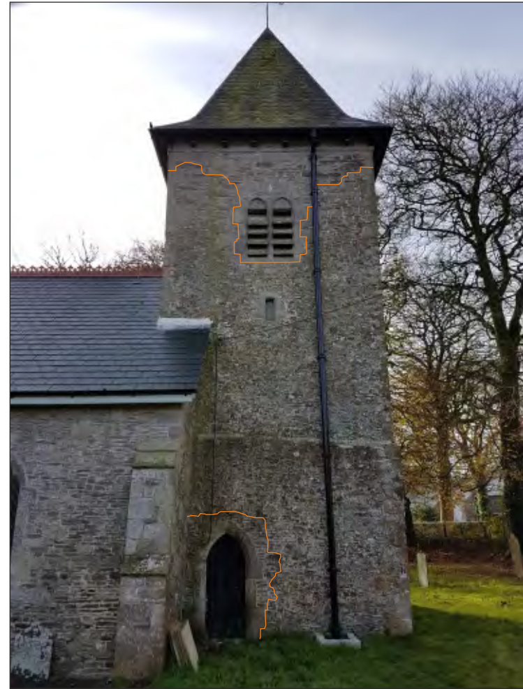
Pl. 13 General view of church tower showing 19th century rebuild (top) and door insert. Looking south.
