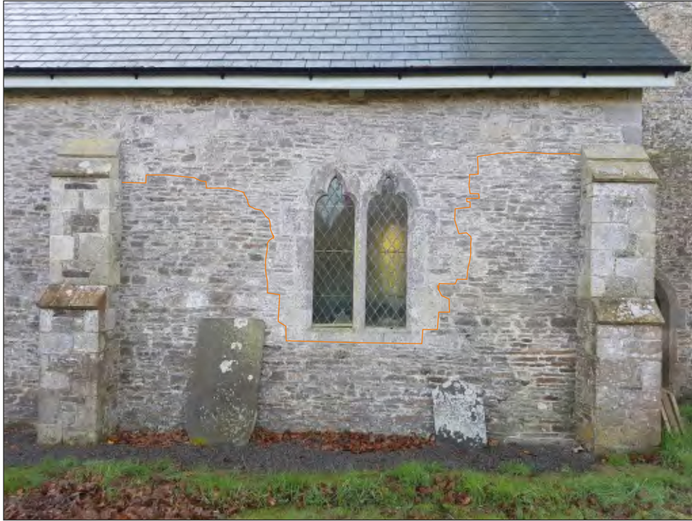
Pl. 18 General view of north elevation showing sections rebuilt in late 19th century. Looking south.
