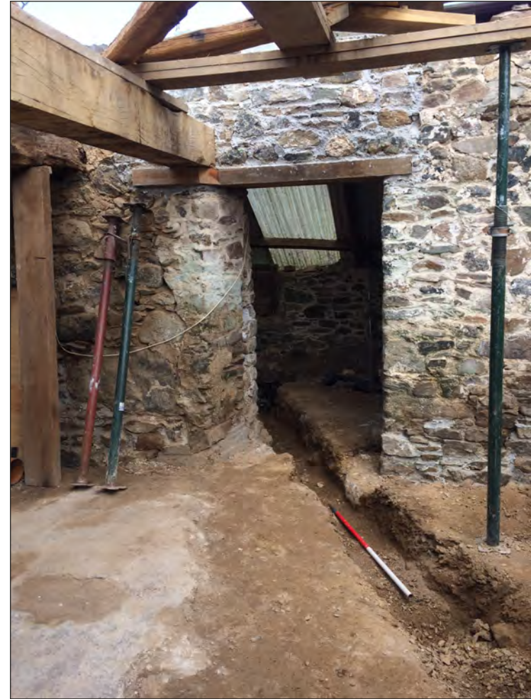
Pl. 2 General view of service trench in former hall and western outshut. 1m scale. Looking north.
