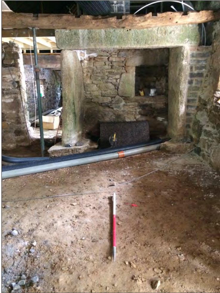
Pl. 1 General view of former hall following removal of concrete floor-slab. 1m scale. Looking east.
