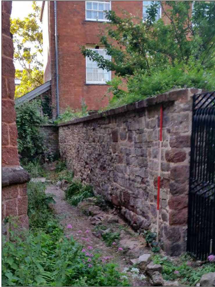
Pl. 1 General view of boundary wall showing No. 26 Bartholomew Street in the background. 2m scale. Looking southwest.
