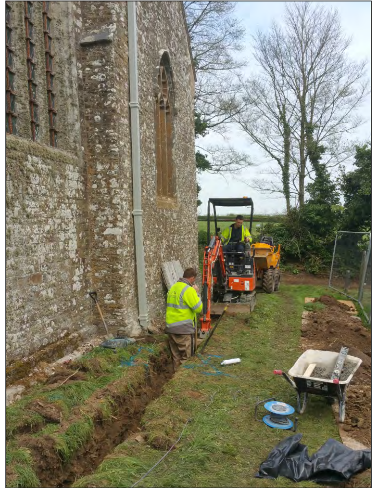
Pl. 2 Excavation of drainage trenching to east of St Pancras church. Looking north.
